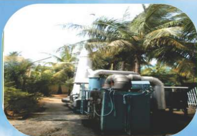
Incinerators provided at Diesel Loco Shed/Gooty, Guntakal, Kazipet, Moula Ali, Workshop & Electric Loco Shed /Lallaguda
