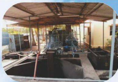
Effluent Treatment Plant provided in Diesel Loco Shed/Gooty, Guntakal, Kazipet, Moula Ali & Vijayawada
