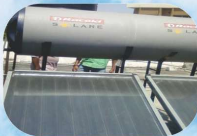
Solar Water Heaters provided at various places 1,70,000 LPD
