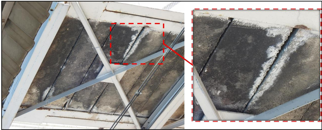
leaching effect observed at bottom of slab panels for 1 st span of FOB
