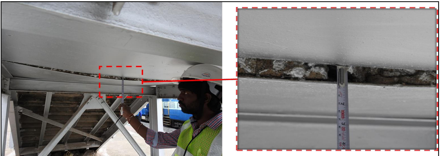
Deformation in MS plate below slab
