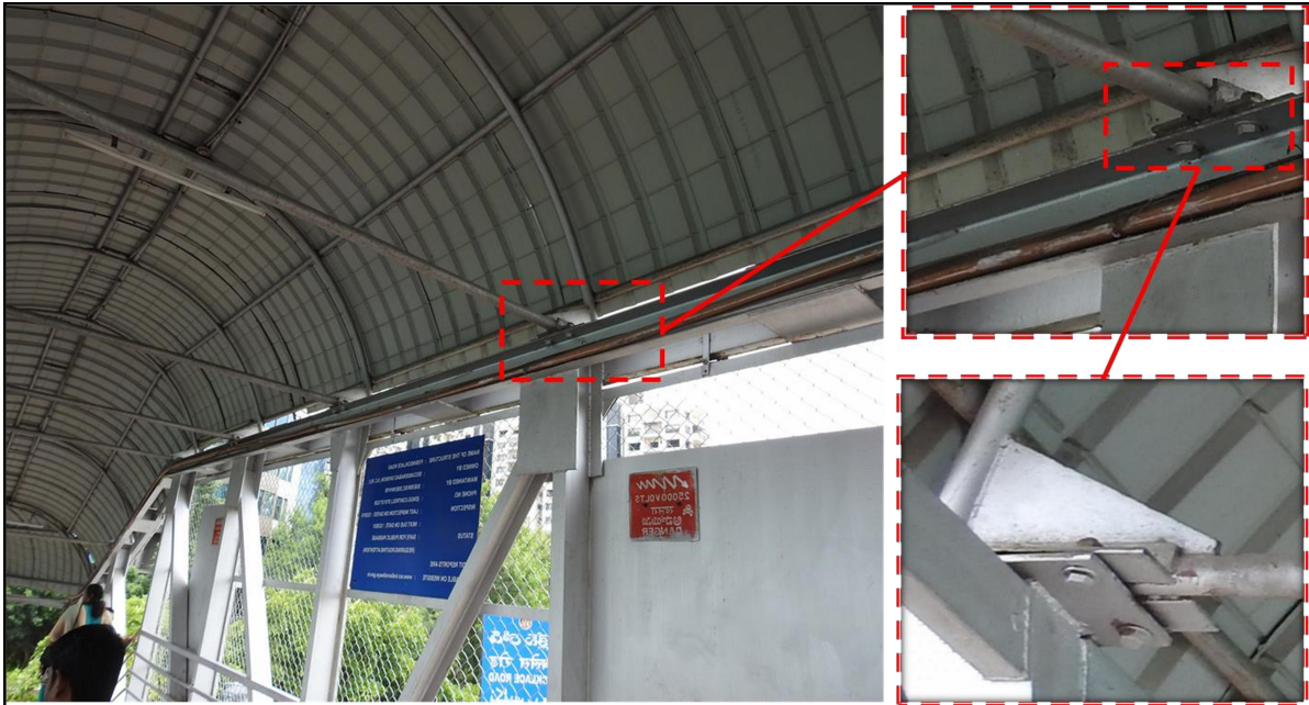
Fig 1: Electrical Cables, Roof truss and Roof sheet and bolted connection
