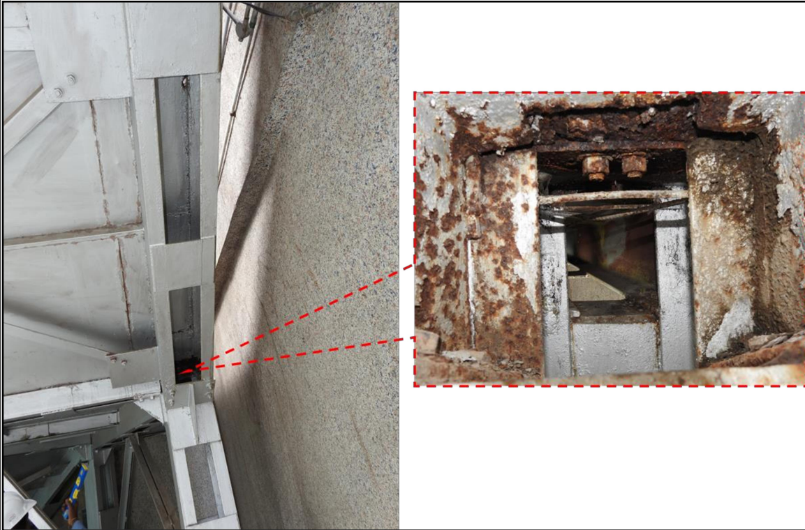
Corrosion observed at Channel built-up section
