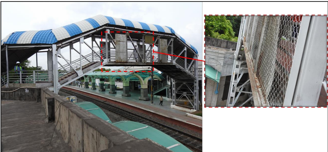
Fig 2: Protective screening mesh for passengers
