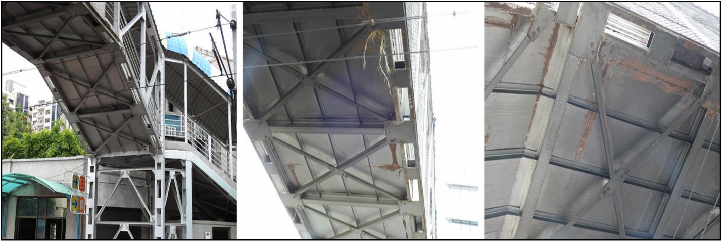
Fig 7: Rusting of sacrificial plate
