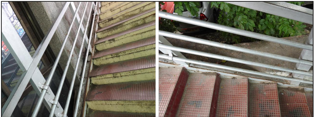
Fig 9: Rusting of staircase supporting channels on both sides
