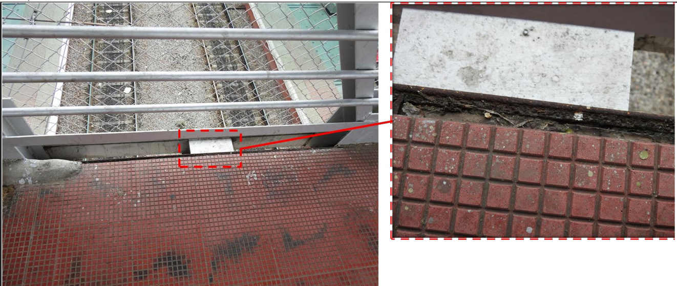
Corrosion observed at slab resting area & tie member
