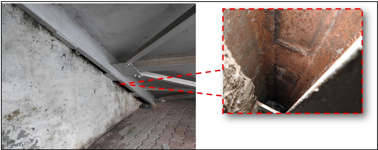
Fig 8: Rusting of Channel section at staircase
