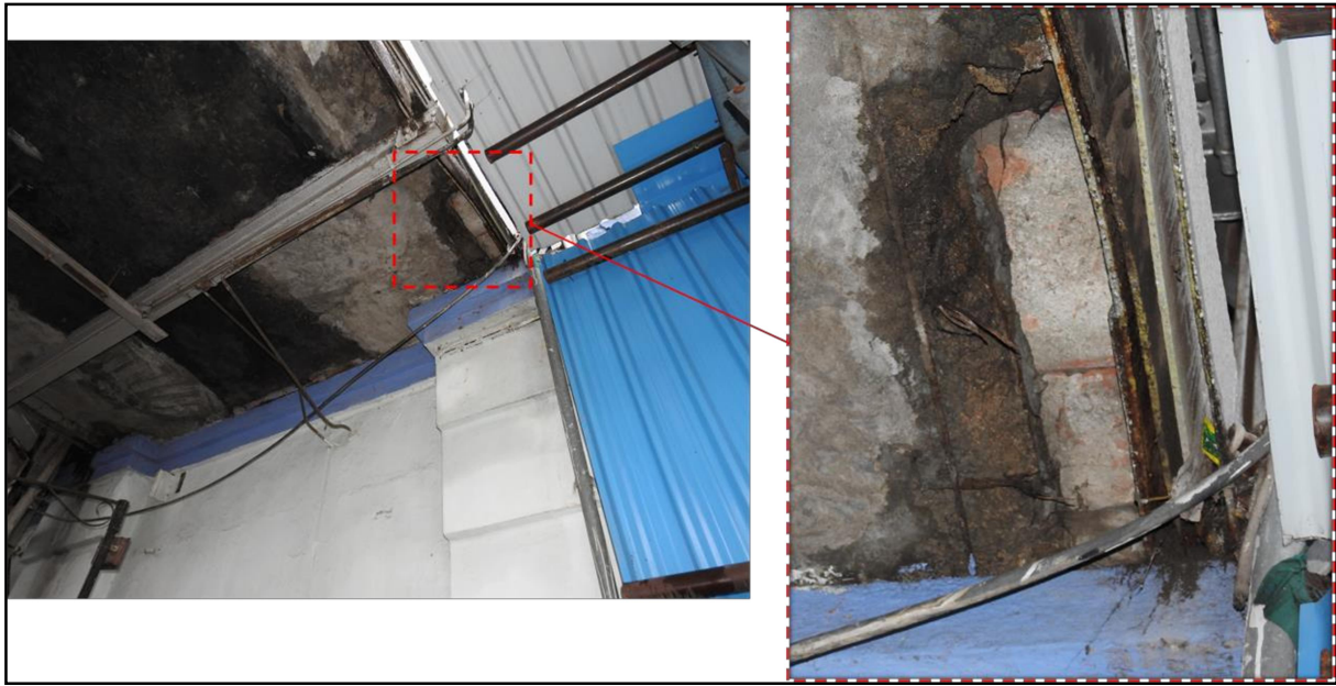
Corrosion is observed in Tie plates
