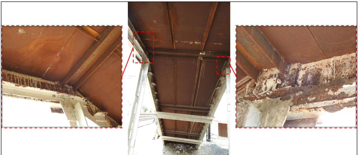
Major Corrosion observed in channel section staircase landing at PF-1
