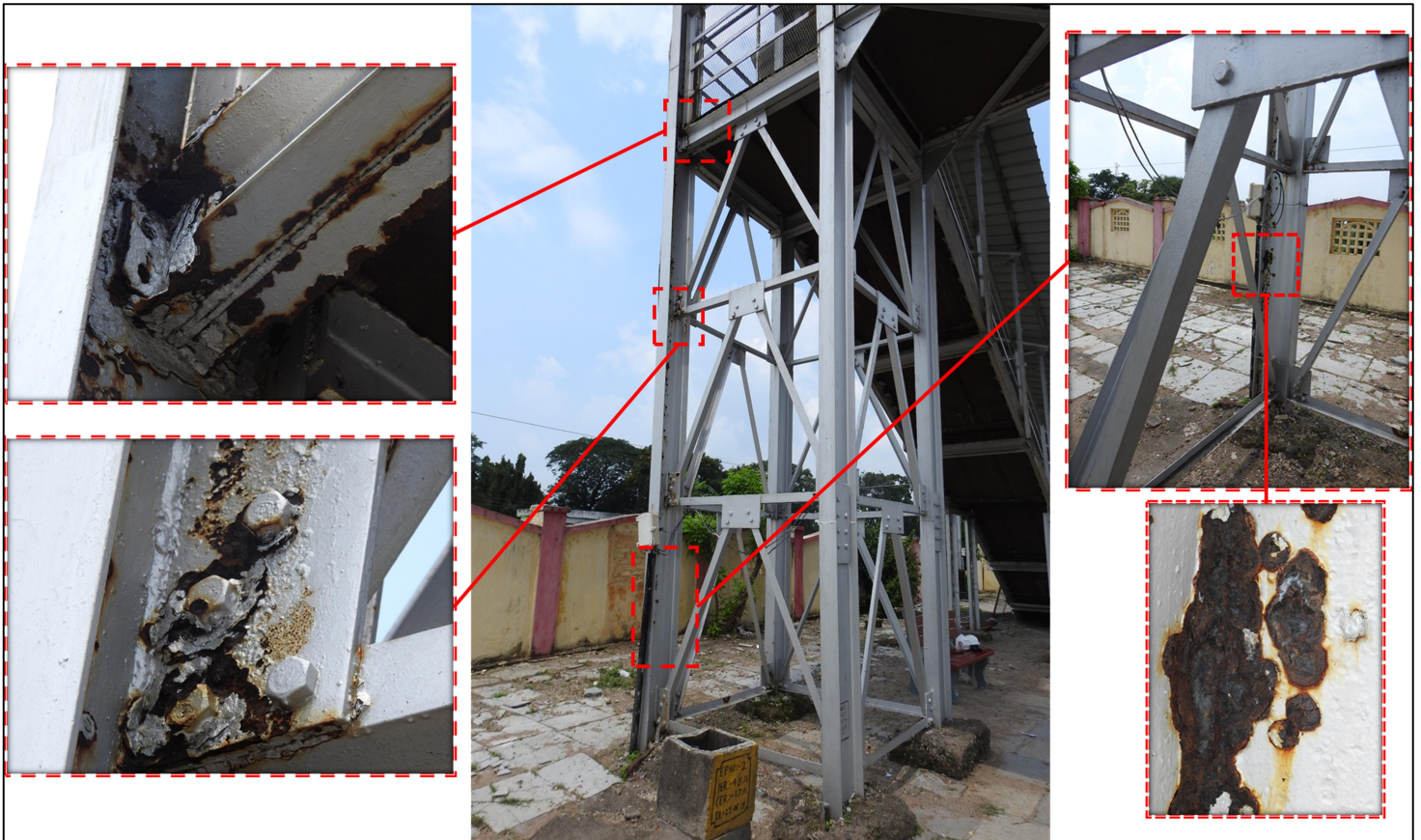
Major corrosion observed
