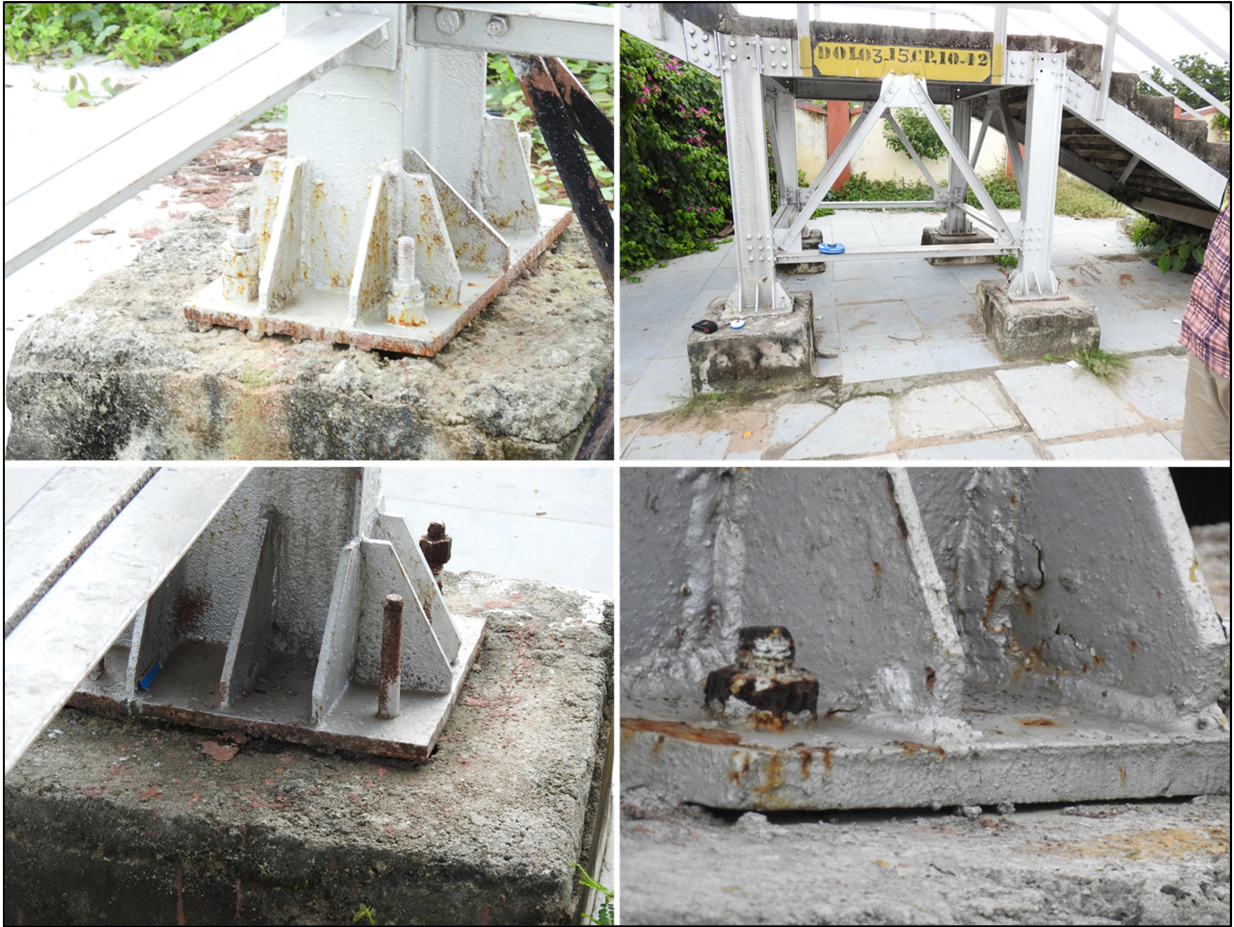
Fig 3: Base plate observed at PF-1 and Stanchions
