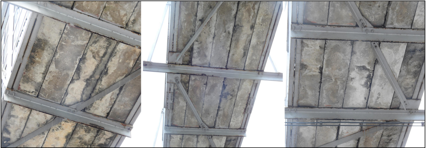
leaching effect observed at bottom of slab panels of FOB
