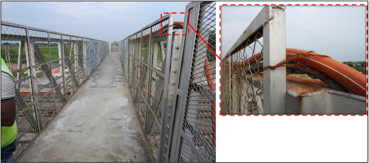
Fig 1: Cables and protective screen
