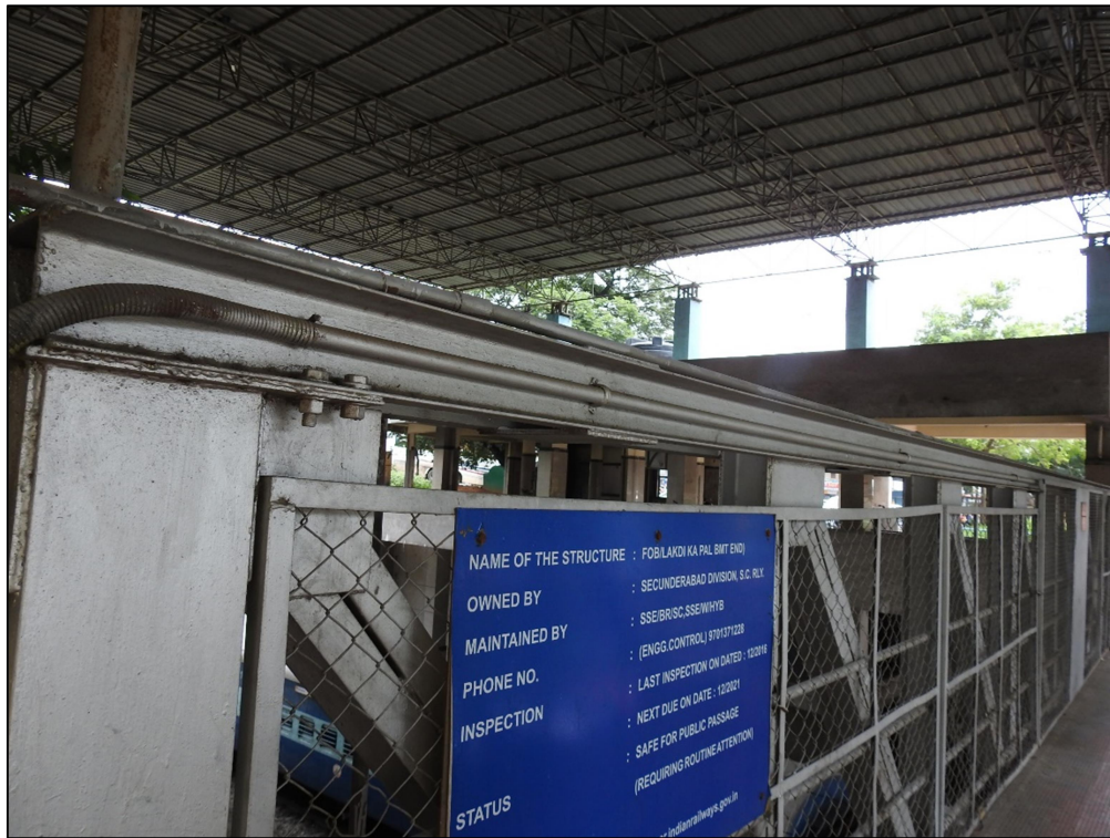
Fig 1: Electrical Cables and Protective screening mesh for passengers
