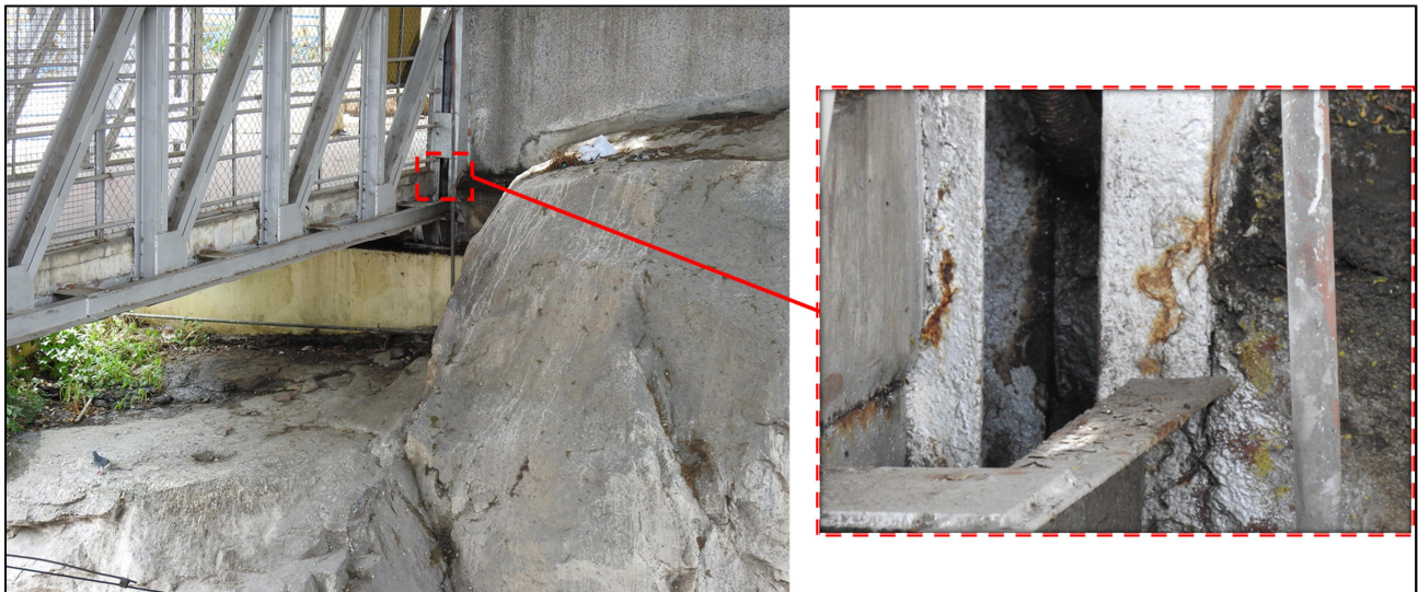
Corrosion observed in Double channel section
