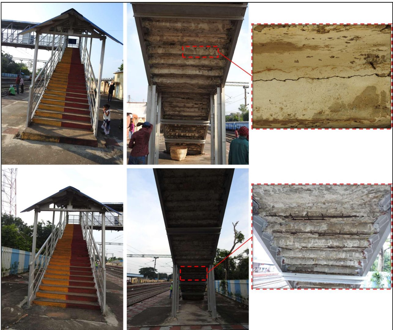
Fig 4: Staircase details, cracks and reinforcement exposure
