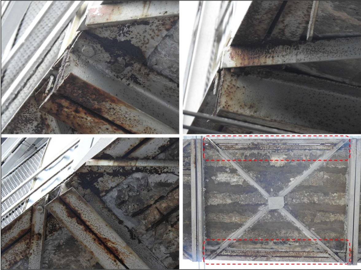
Corrosion observed in Floor beams joints
