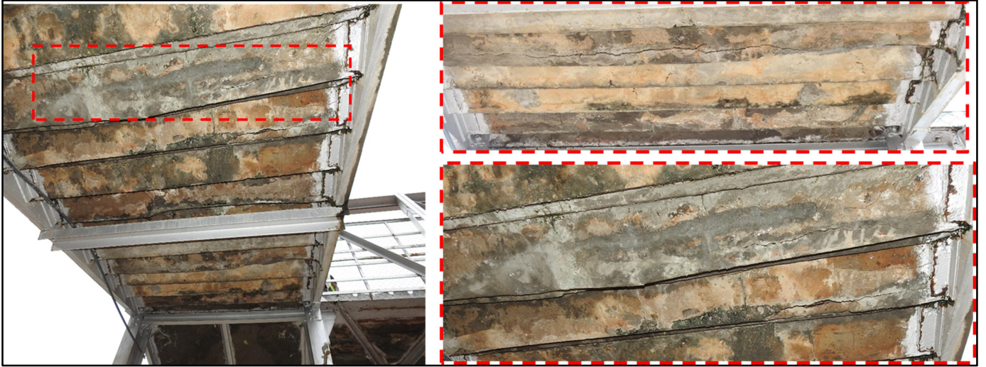
Fig 10: cracks are observed in staircase slabs
