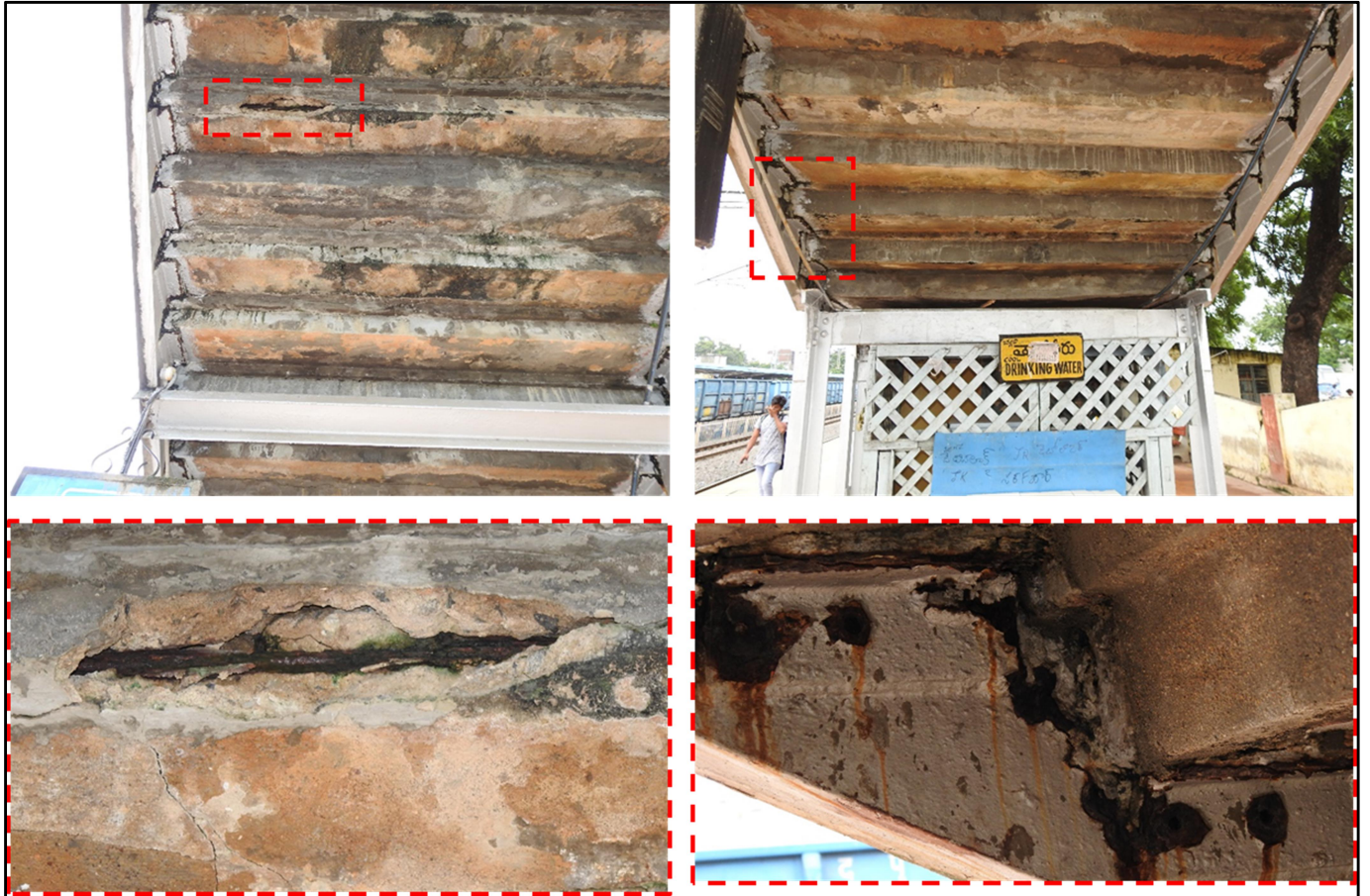
Fig 8: Spalling in staircase slabs
