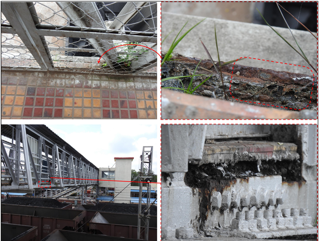
Fig 6: Corrosion is also observed at steel concrete joint
