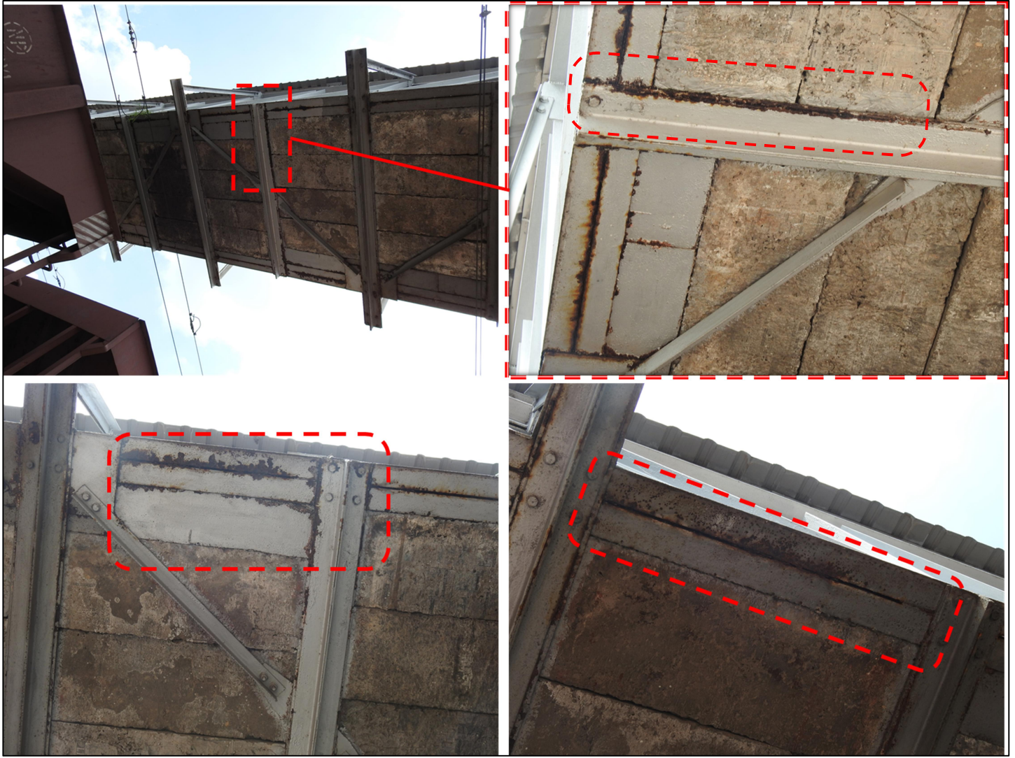
Corrosion of Floor beam and rusting of bottom chord members
