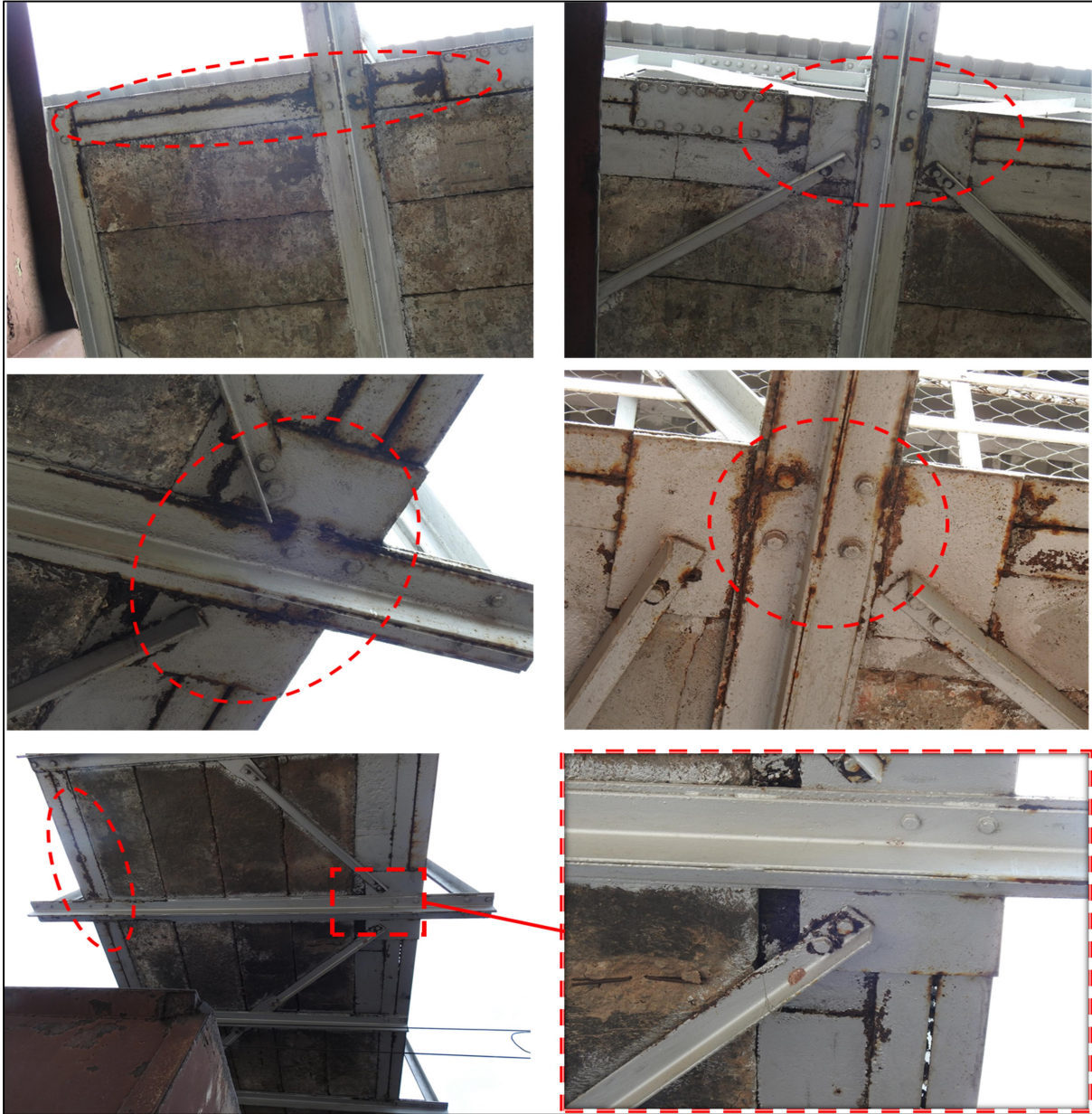
(a) Corrosion in gusset plate joints and bottom chord double angle section
