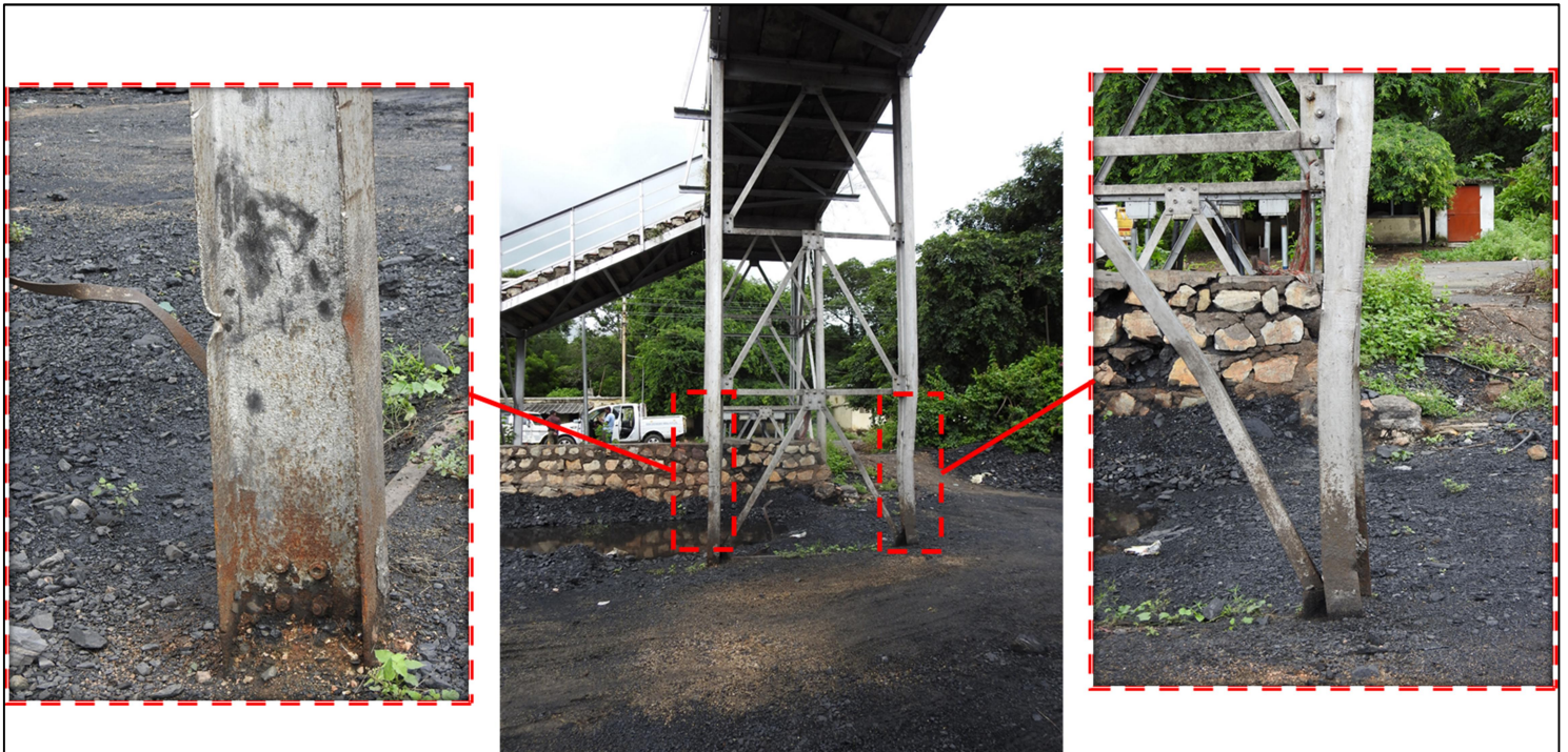
Fig 6: Accidental damage observed at stanchion in coal yard
