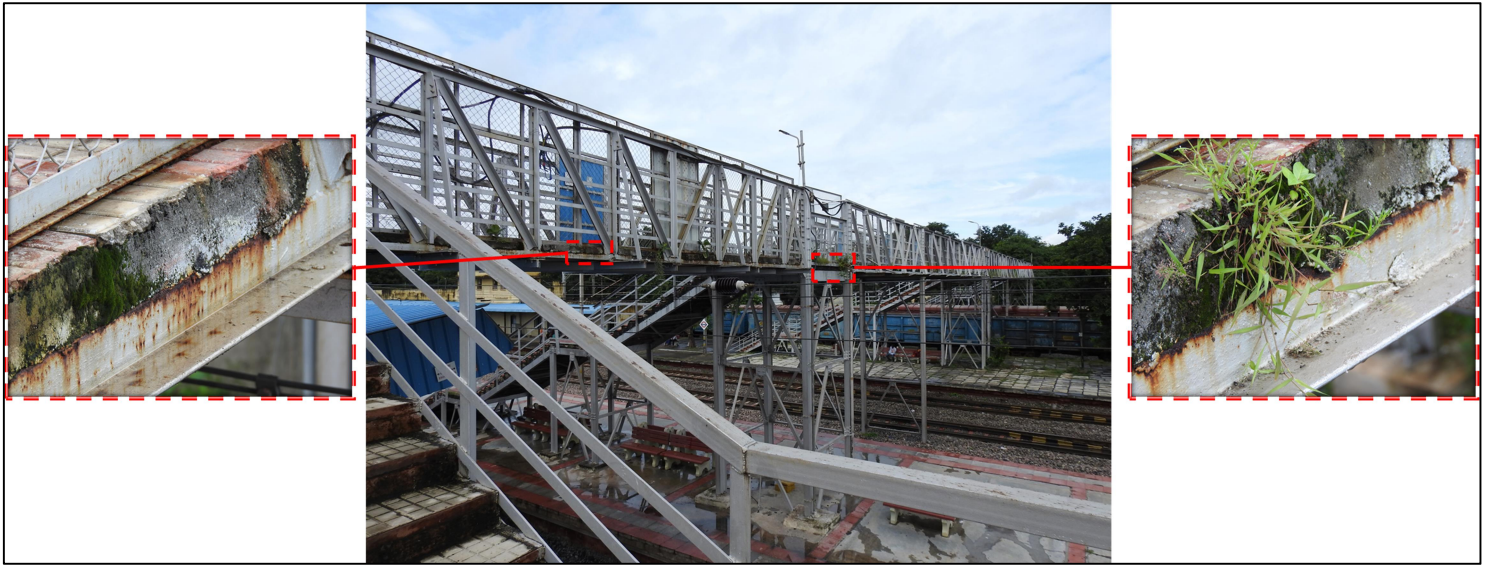
Fig 7: Corrosion and vegetation
