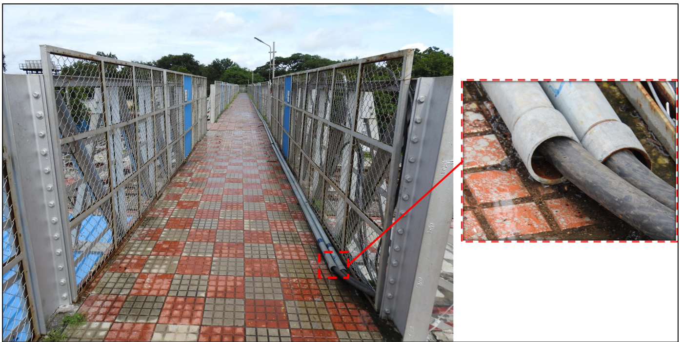
Fig 1: Cables, Flooring and protective screen
