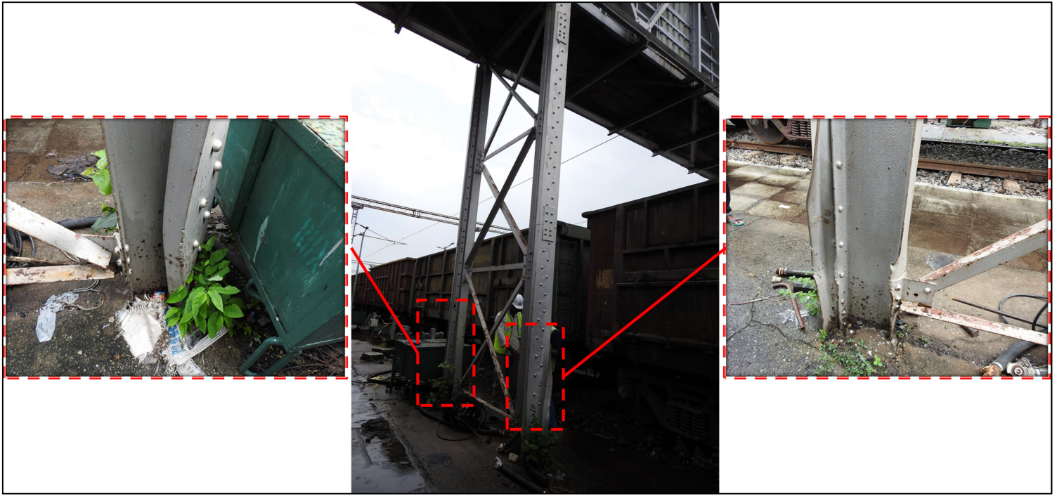
Fig 6: Accidental damage observed at stanchion 1
