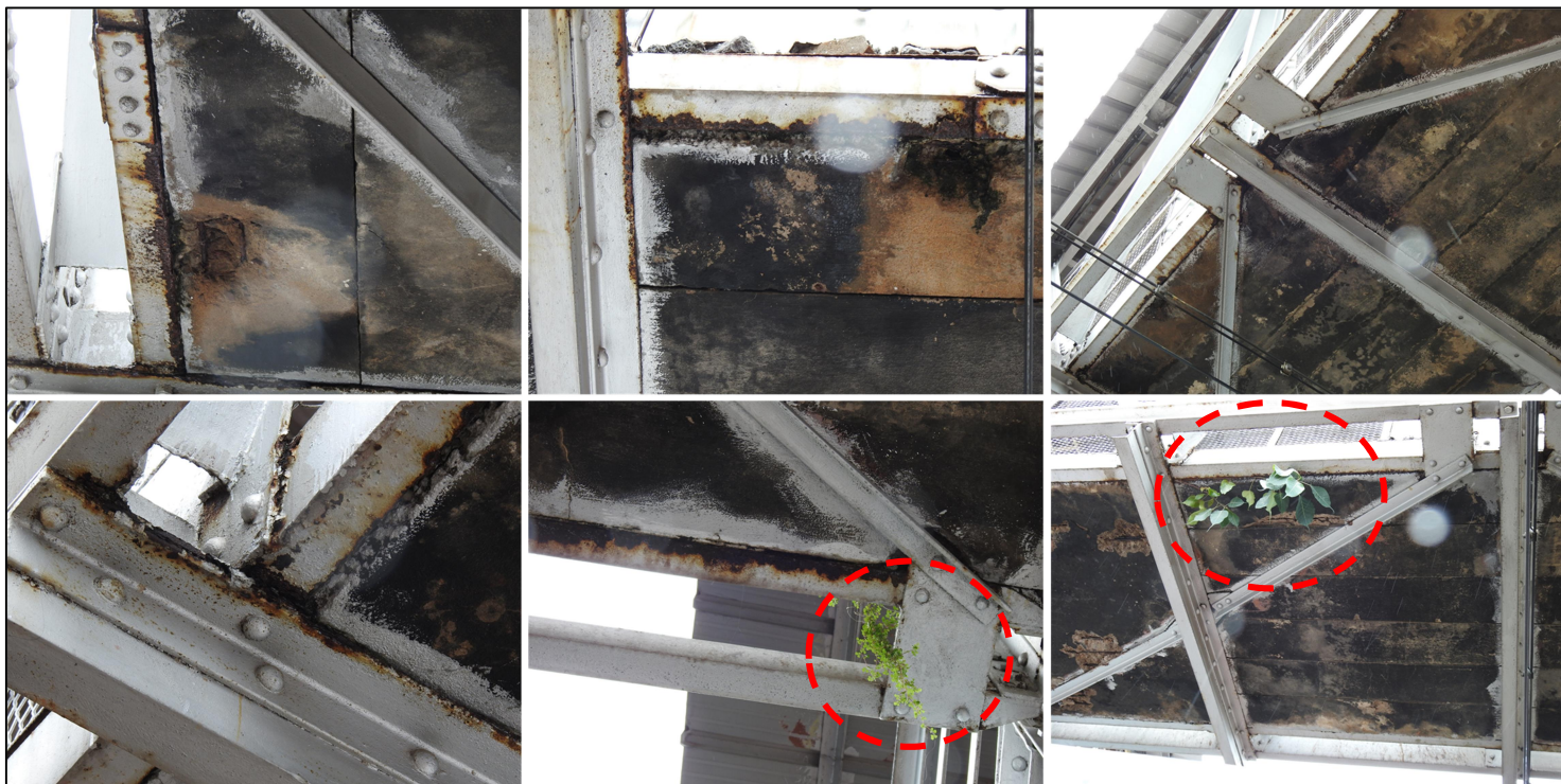
Corrosion and vegetation
