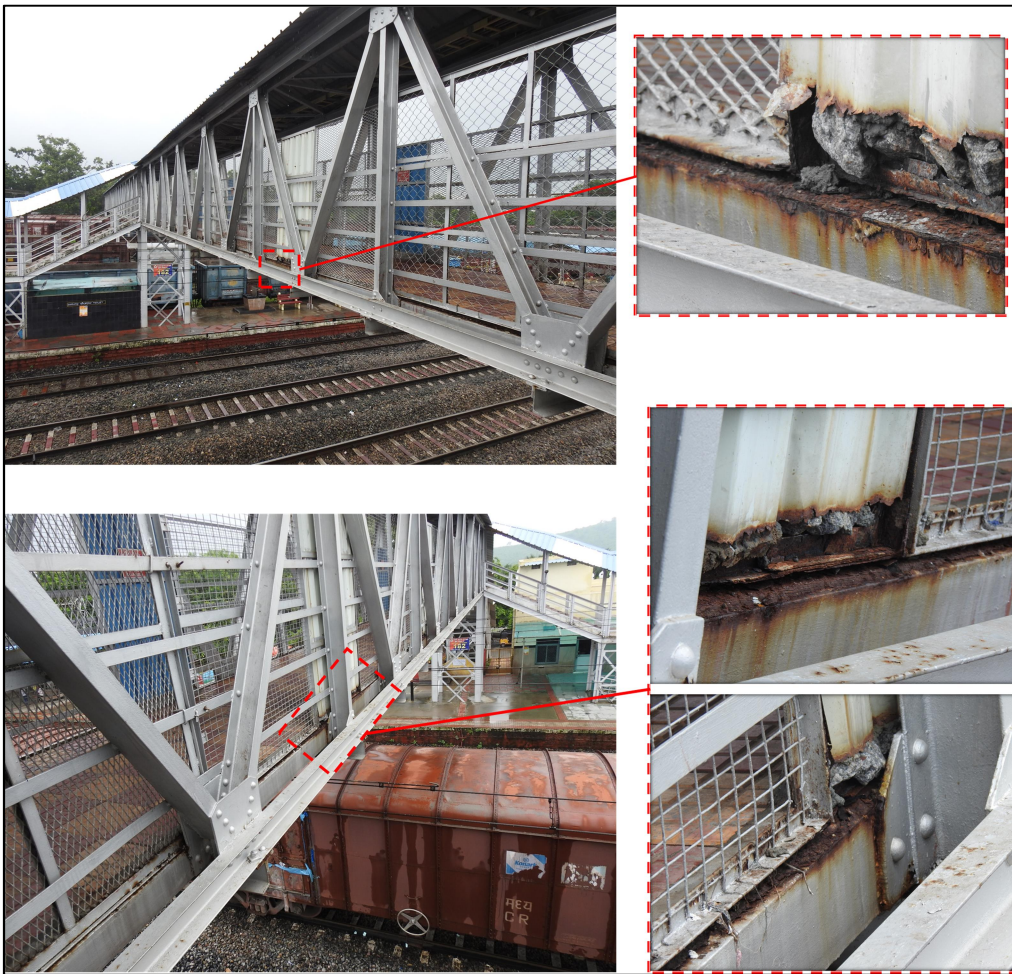
Leaching and Cracks in Pre-cast panels of 1 st span
