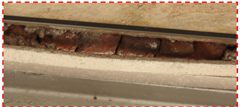
Fig 6: Gap above floor beam
