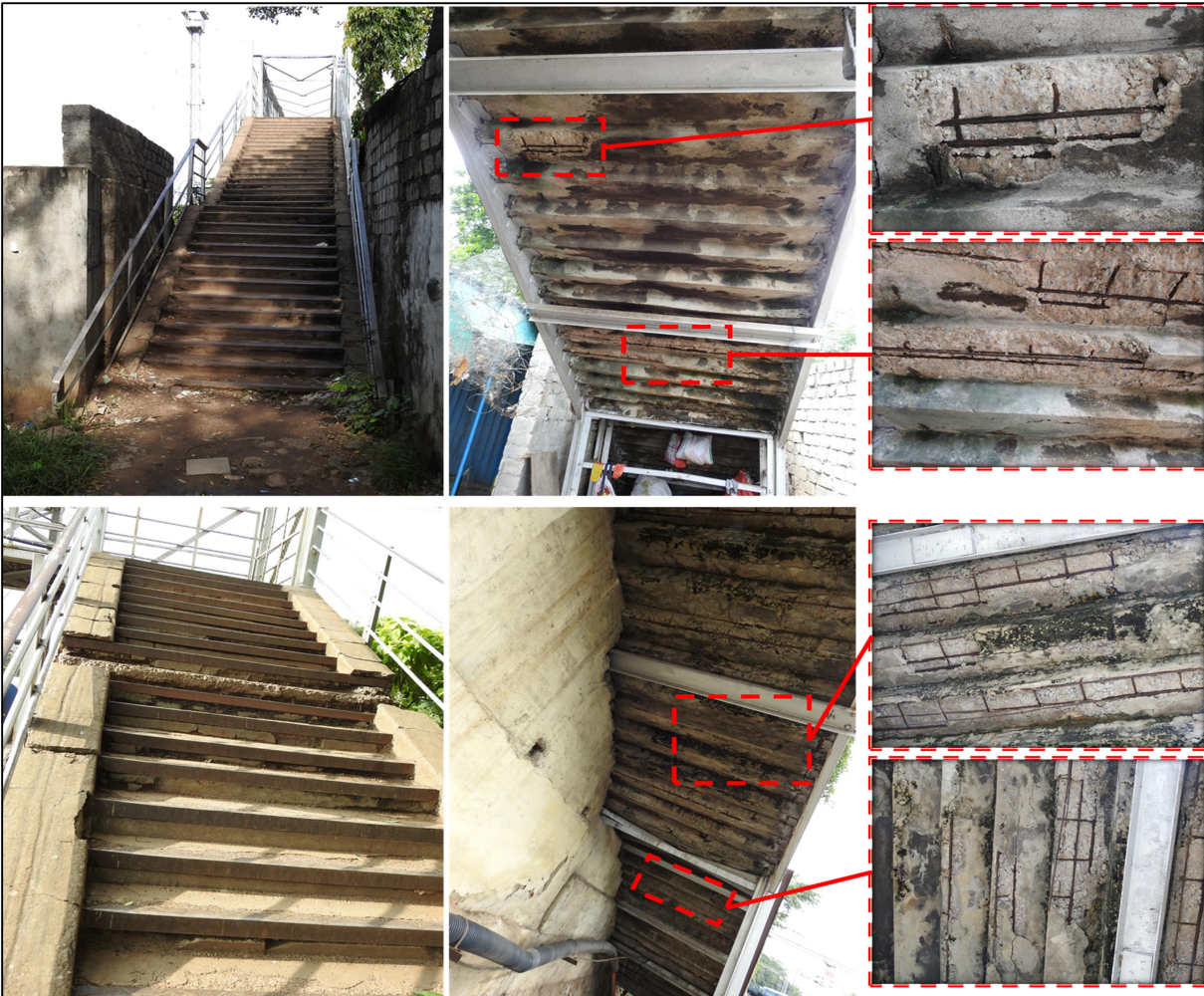
Fig 5: Staircase details, Spalling & exposure of reinforcement
