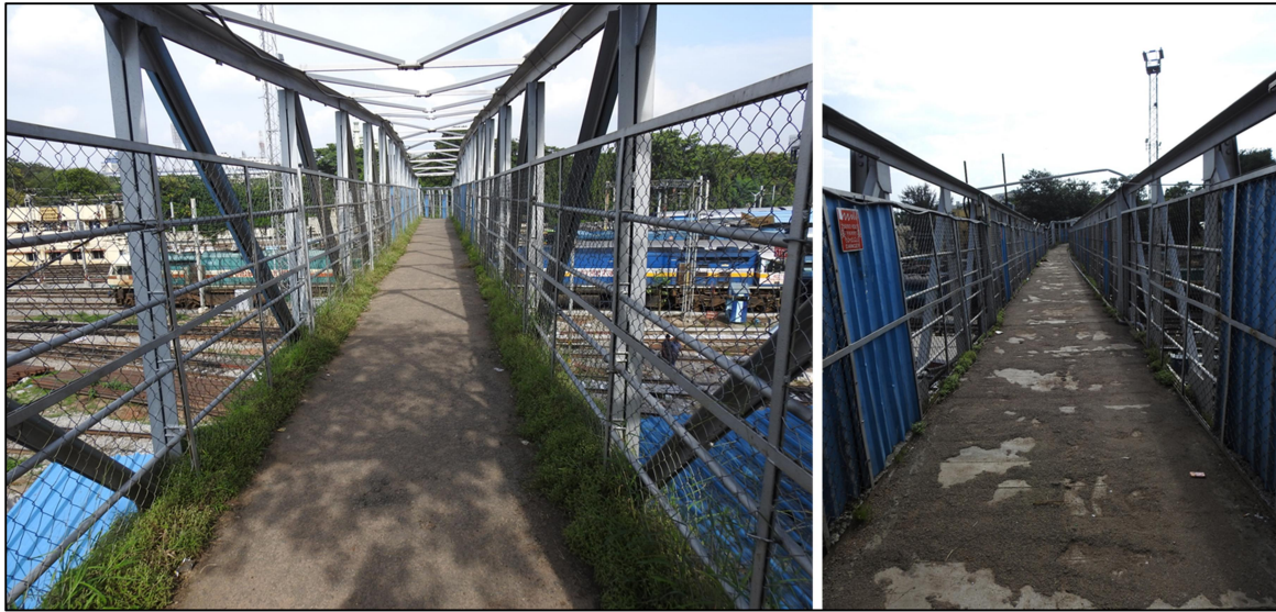
Fig 1: Cables, Flooring, vegetation and protective screen
