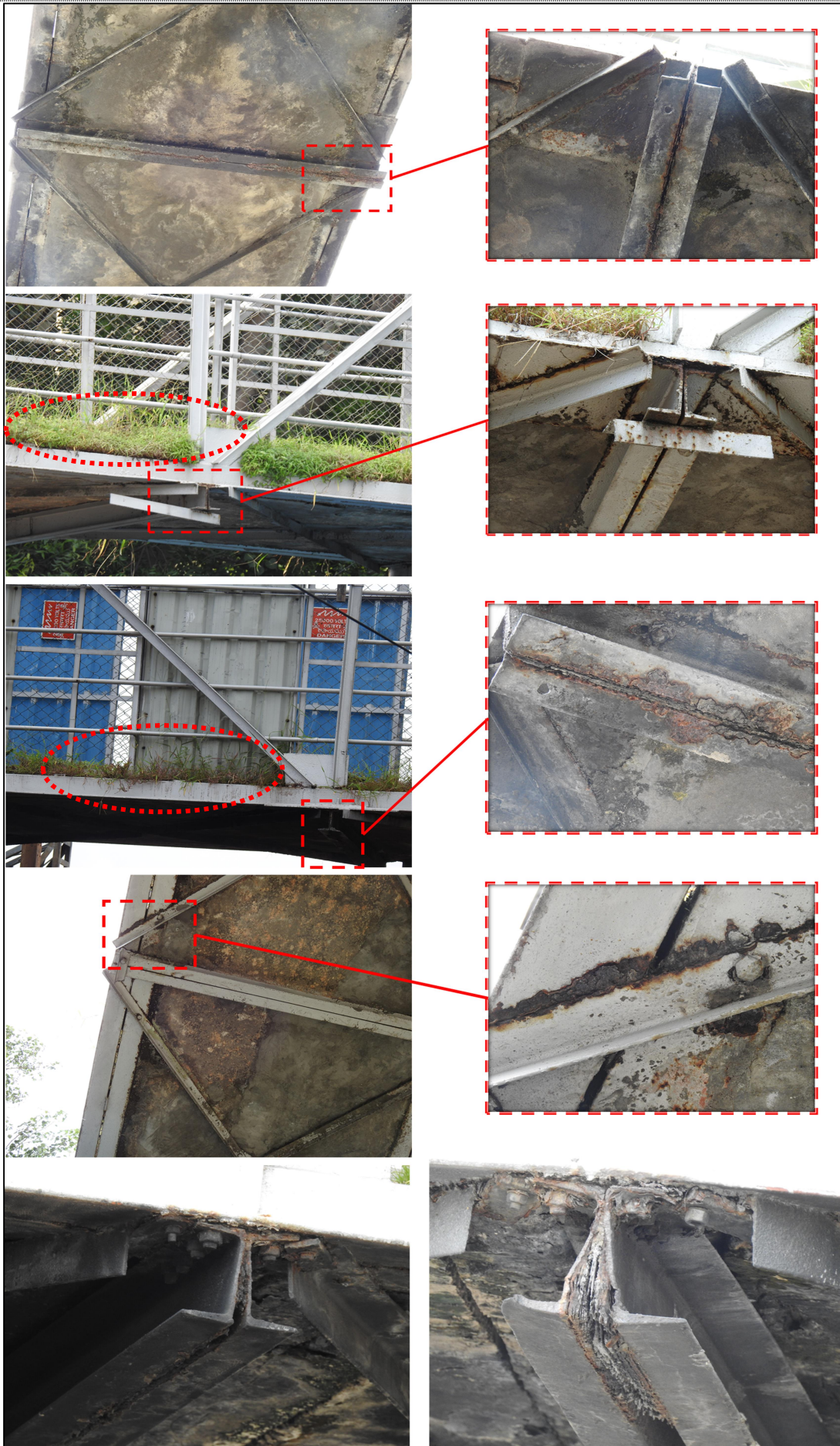
Corrosion and deformation of floor beam
