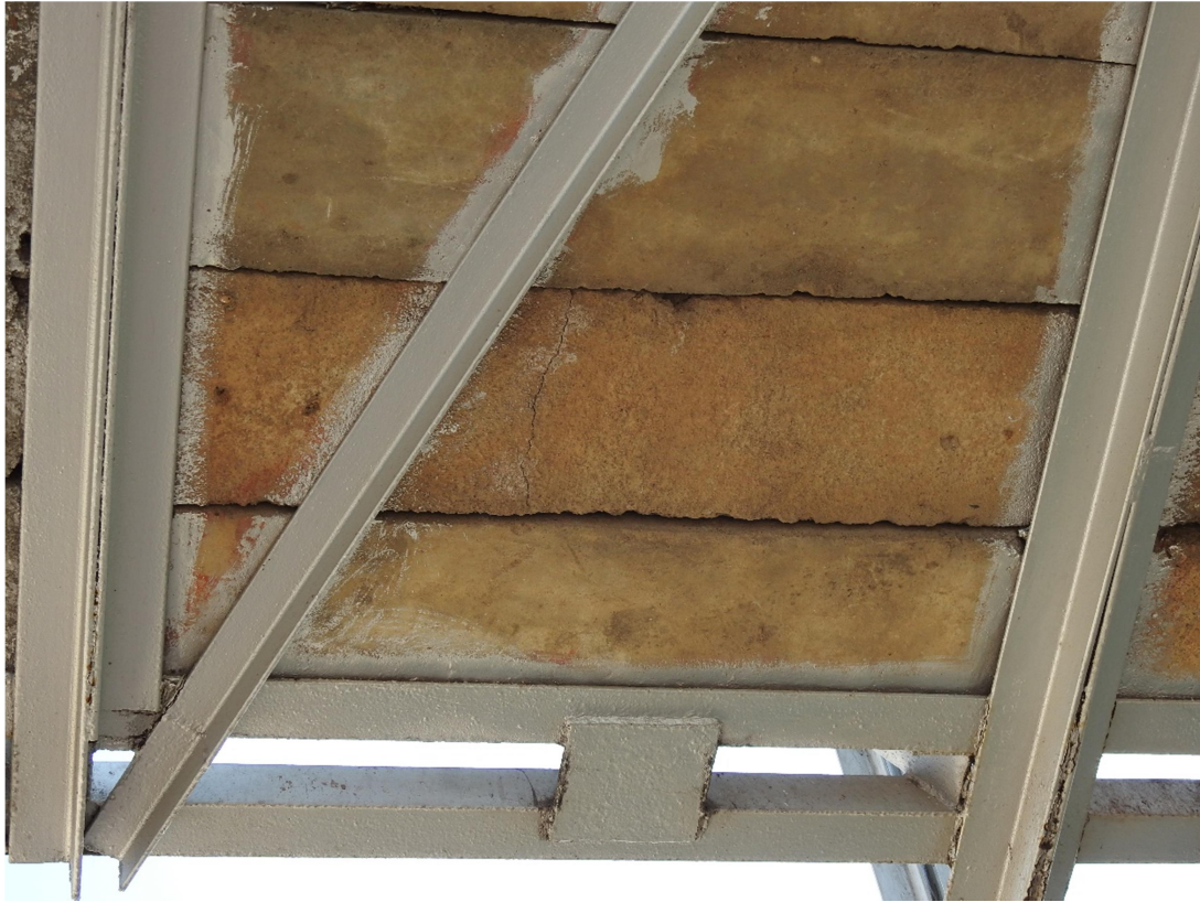
Fig 4: Cracks are observed in Pre-cast RCC slab panels (bottom view)
