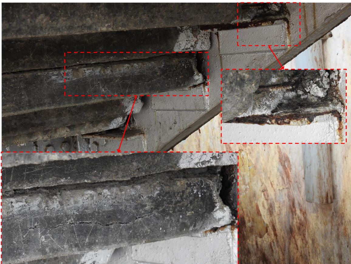
Fig 4: Cleat angle below staircase steps are corroded
