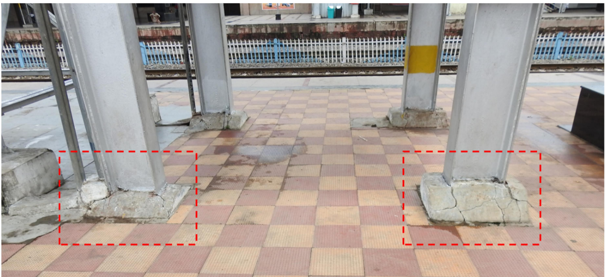
Fig 6: Concrete Encasement for vertical trestles on platform 2 are damaged
