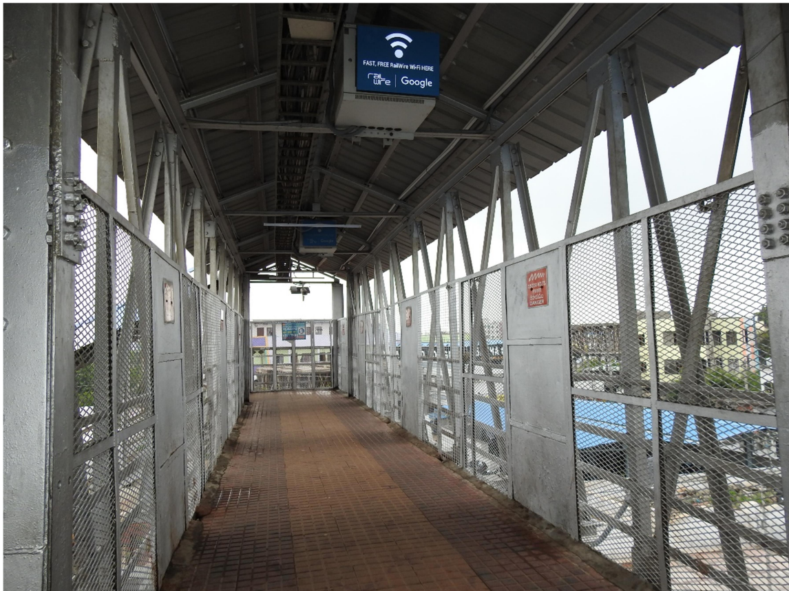
Fig 3: Rail Wi-Fi units are supported on roof truss
