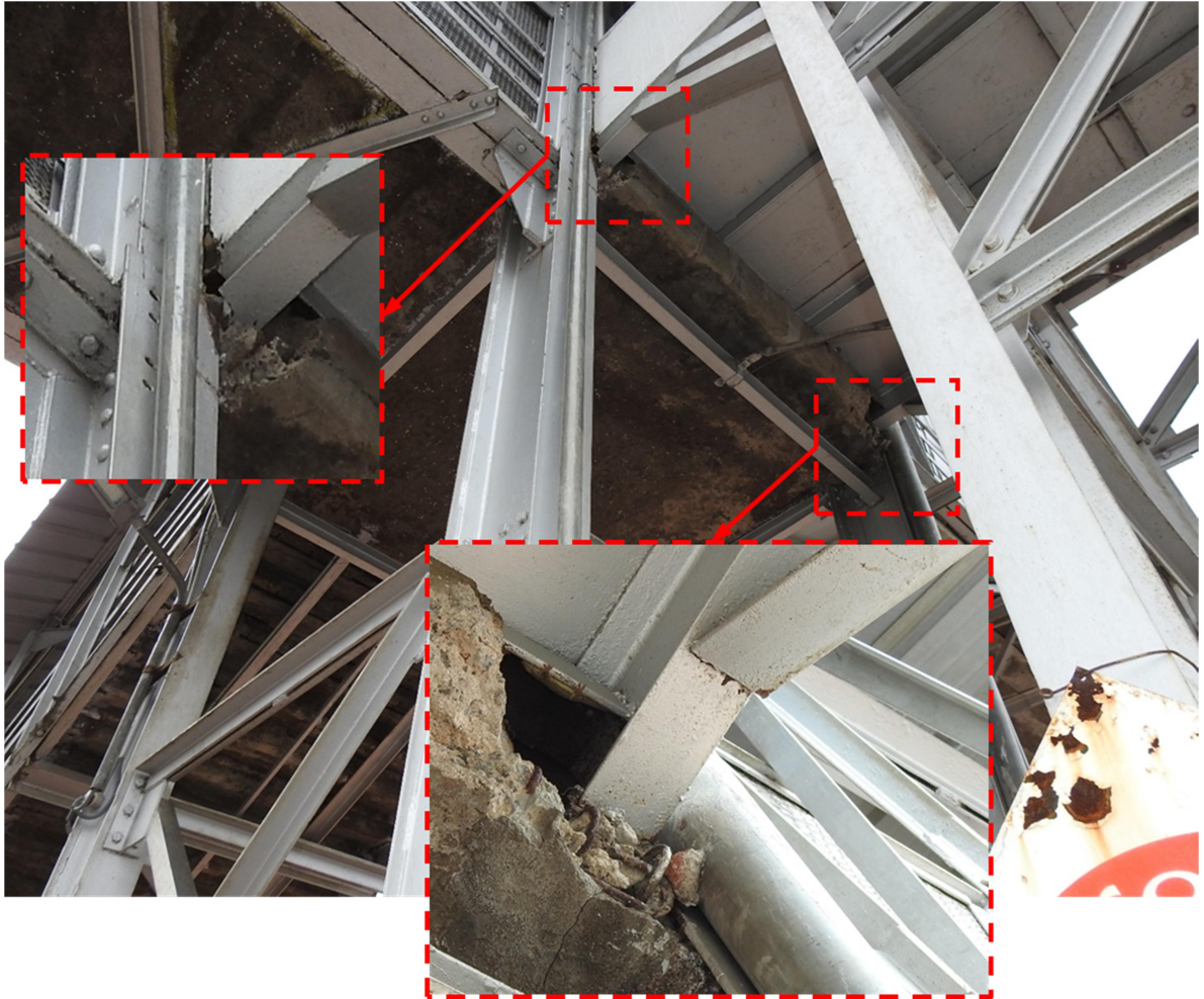
Fig 5: RCC slab broken to support elevator: reinforcement left exposed
