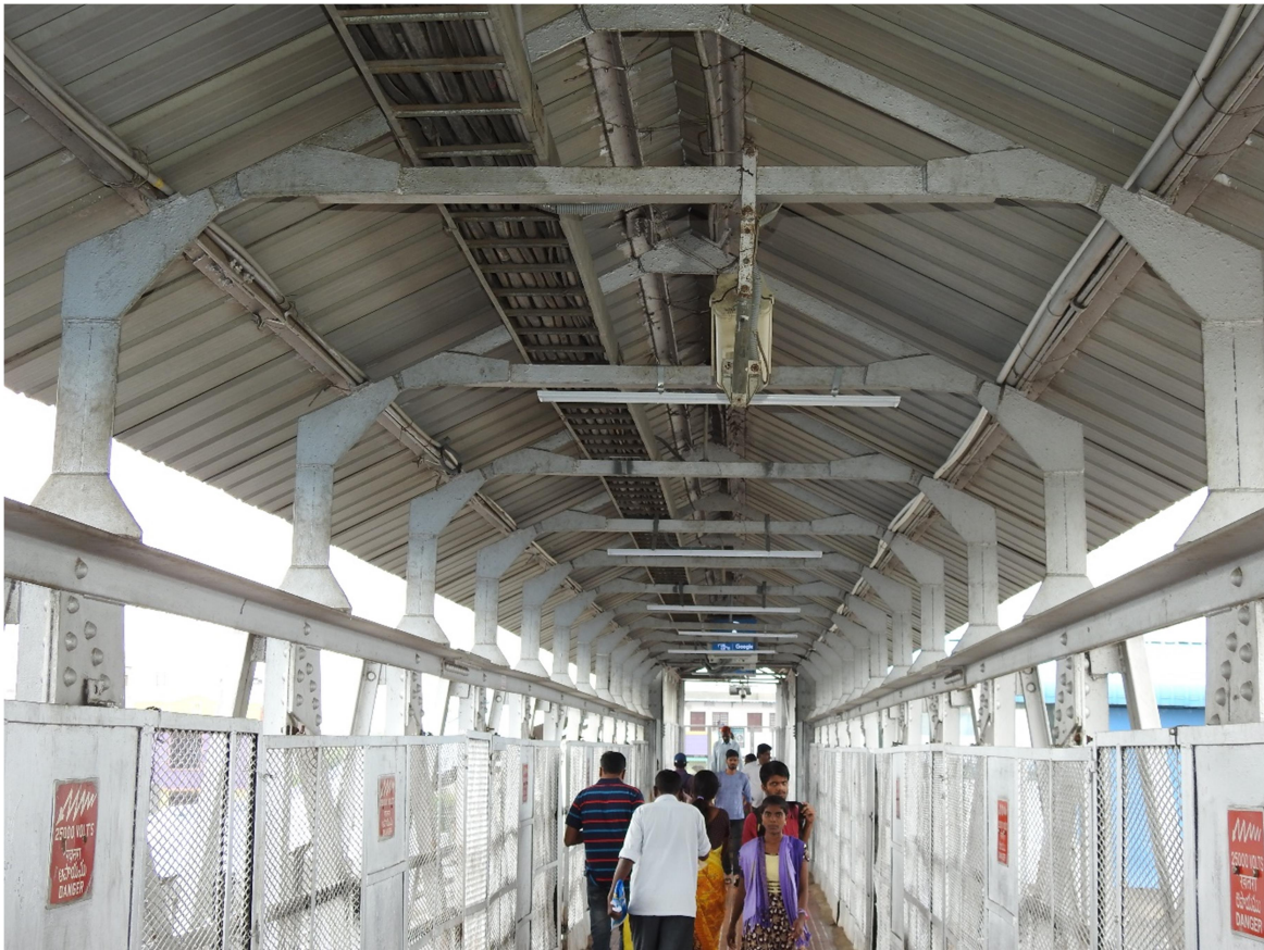
Fig 2: Set of cables running along the length of FOB
