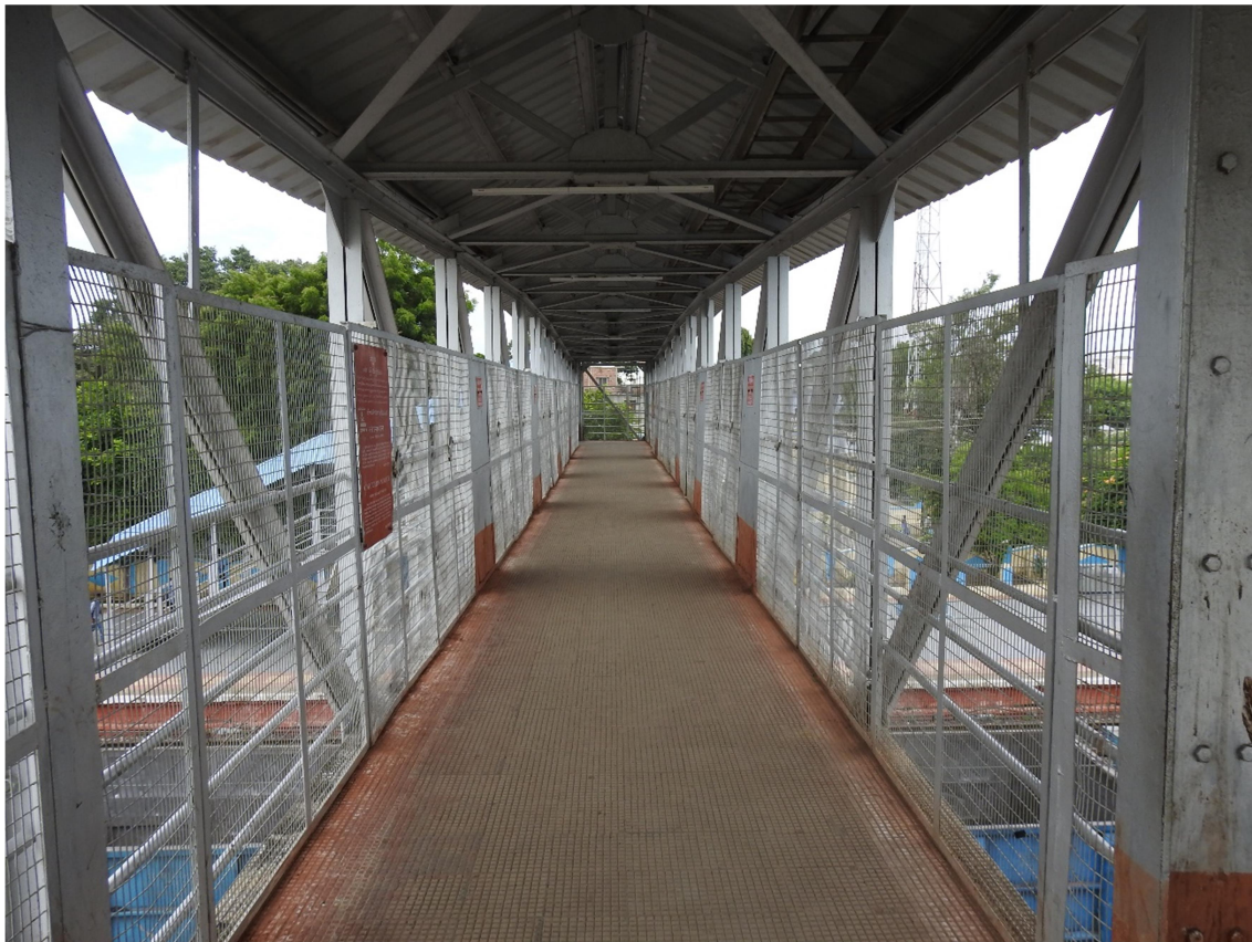
Fig 4: GI 2 mm thick wire rectangle mesh and sheet is provided for passenger protection
