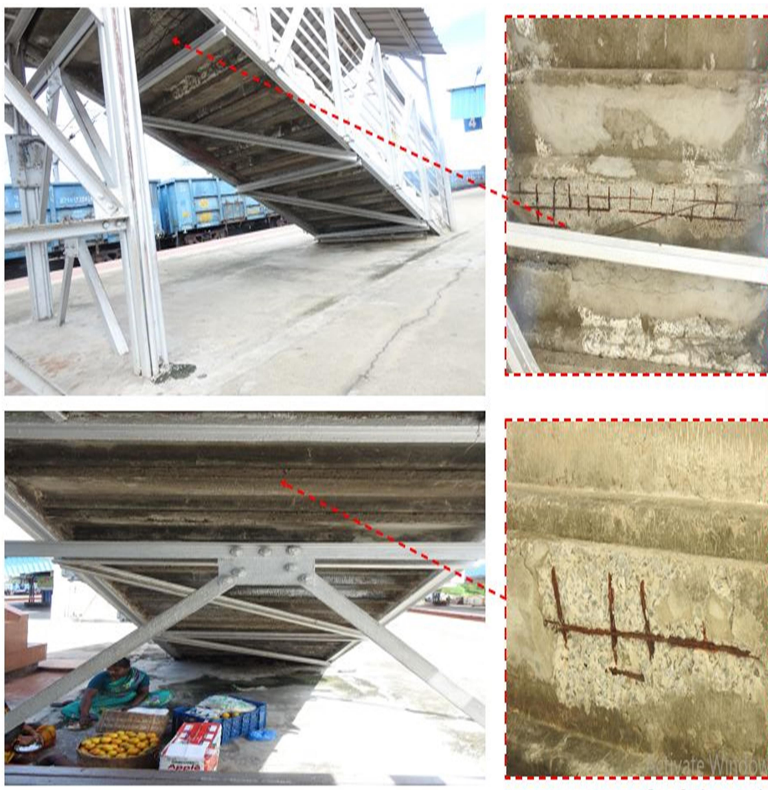
a) Reinforcement exposed in slab panels
