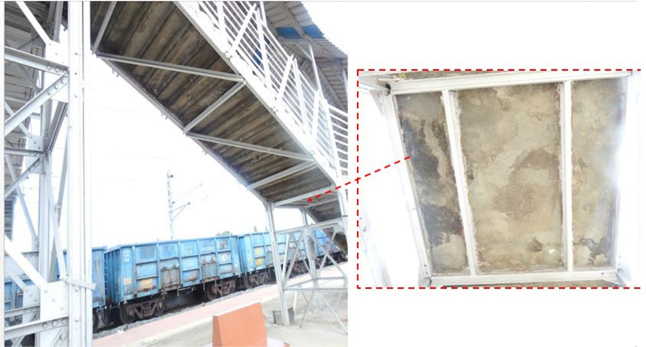
b) Leaching effect on staircase pre cast slab panels
