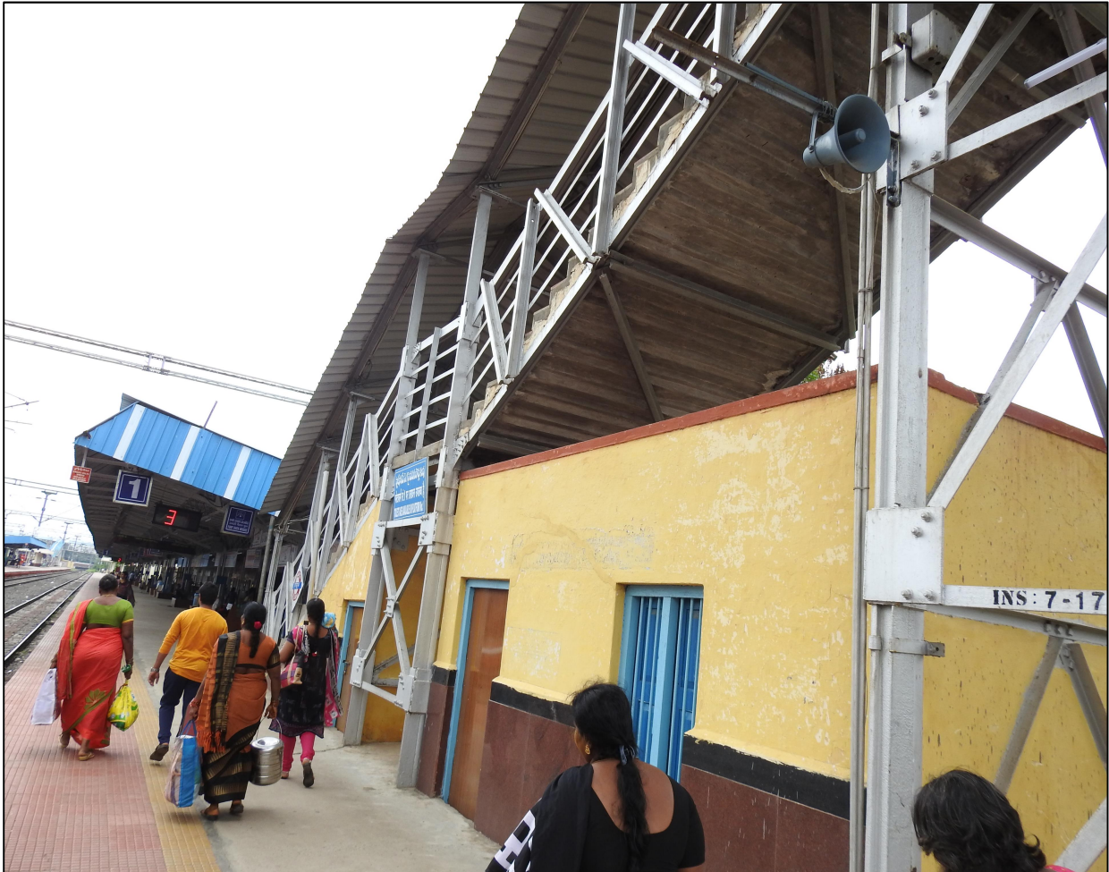
Fig 6: Unable to inspect under stair case due to existing rooms below Stair case flight,
