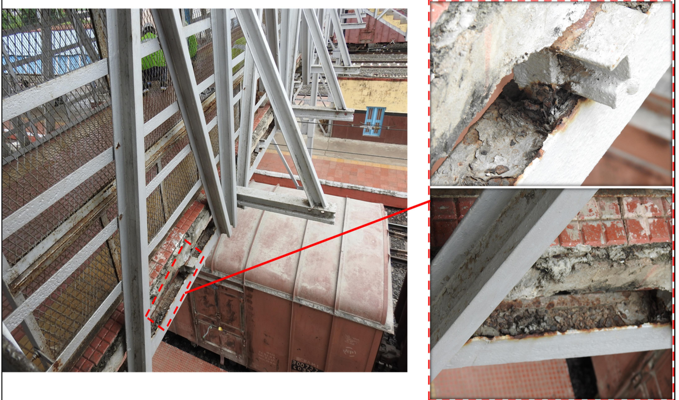
(c) Rusting and corrosion at Bottom chord
