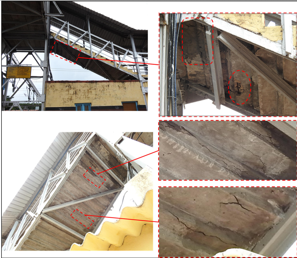
(b) Exposed reinforcement and cracks in steps
