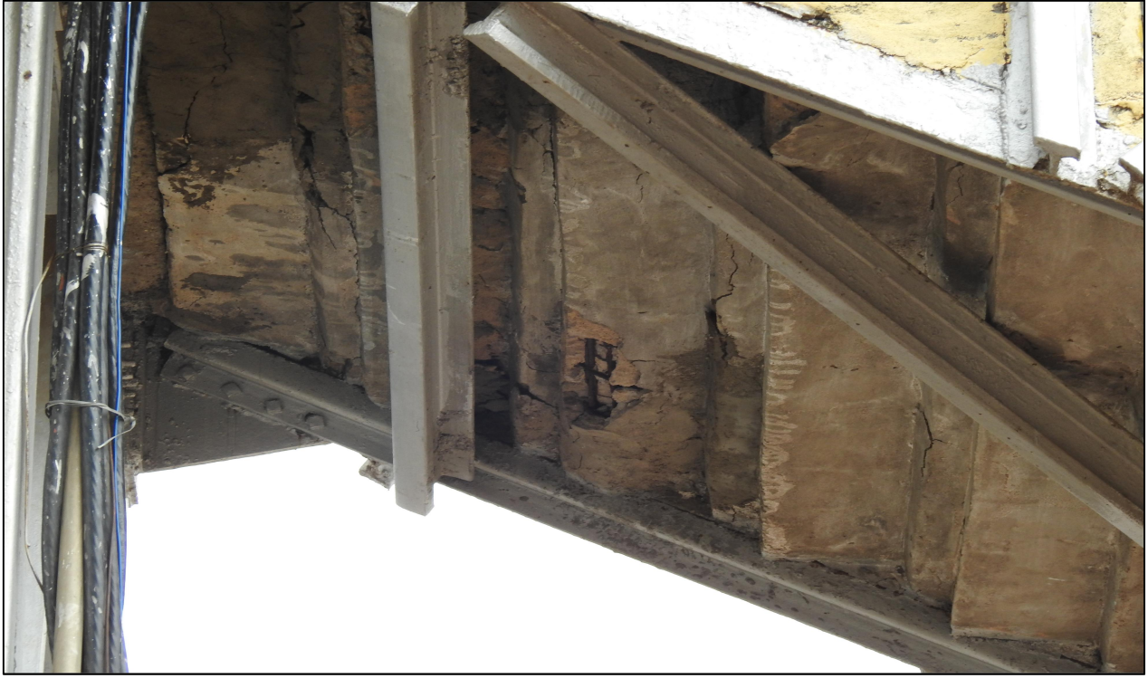
Fig 8: Patch work is observed at PF-2 stair case flight slab panels
