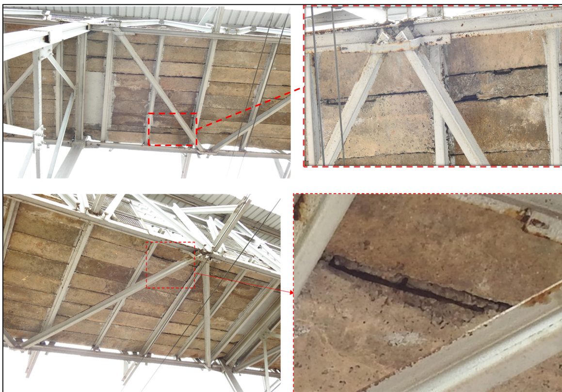
(a) Exposed reinforcement, concrete spalling
