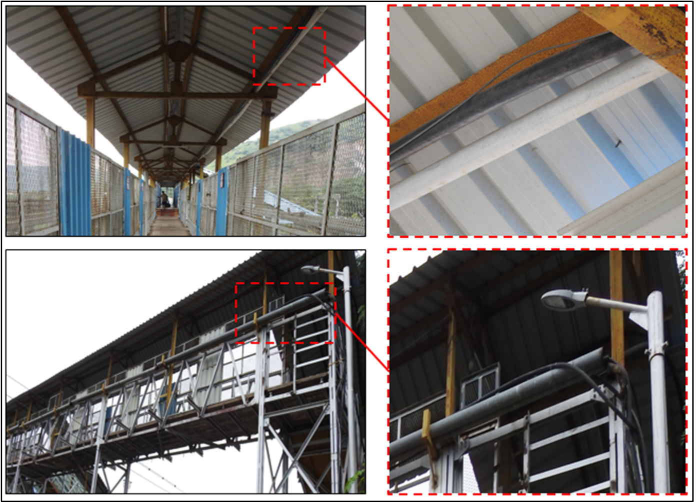
Fig 3: Additional loads of GI, HDPE, PVC pipes
