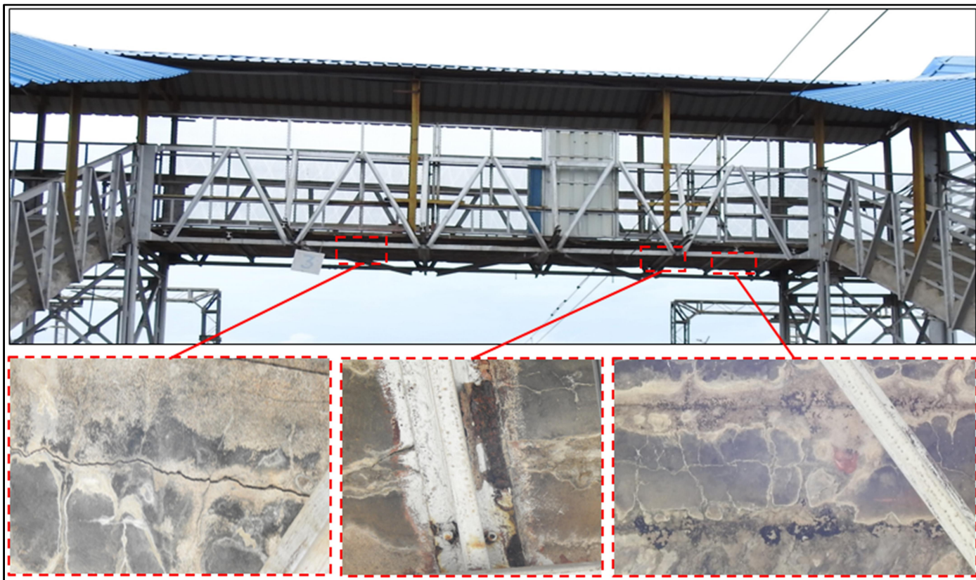
e) Cracks , Corrosion and Leaching in slab panels on Span-3
