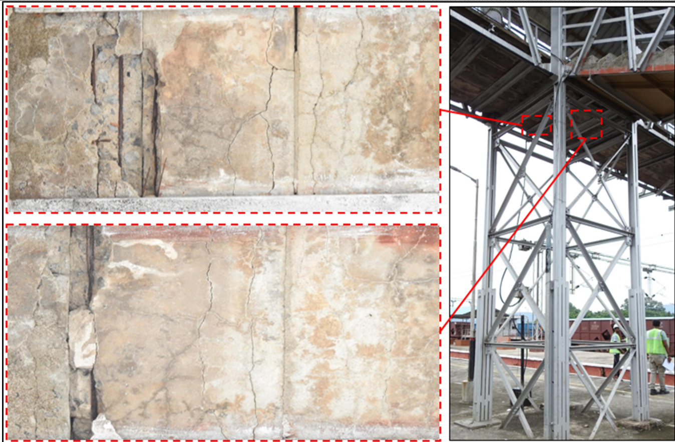
b) Exposed reinforcement and cracks on bottom of slab panels (Staircase 2 - Main landing)
