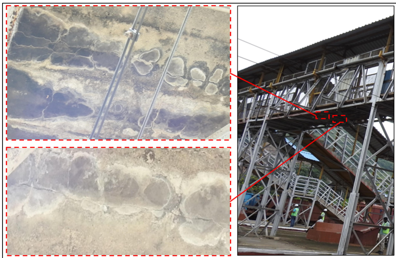
d) Cracks and Leaching in slab panels on Span-2
