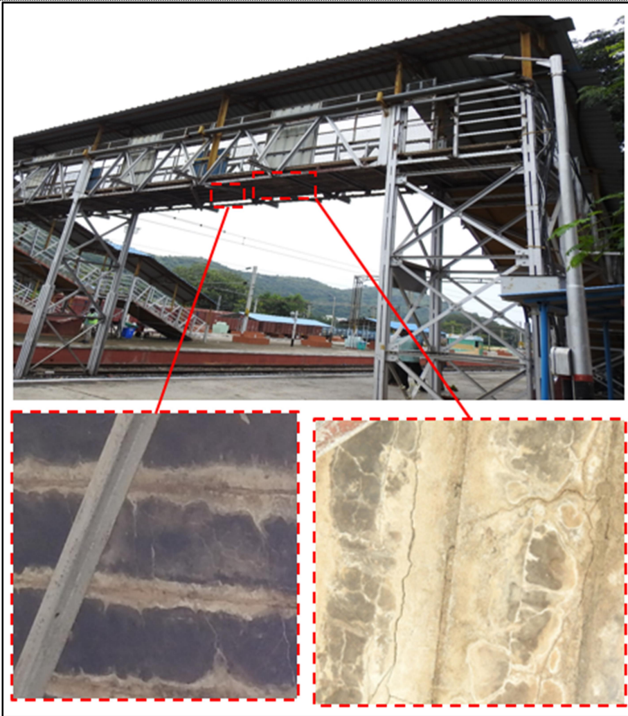
b) Cracks and Leaching on slab panels on Span-1
