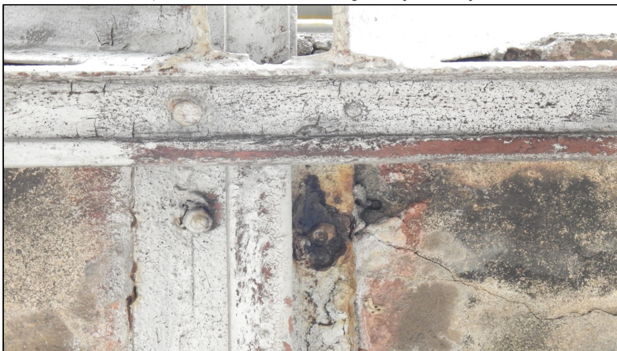
f) Corrosion and rusting observed in Floor beam and bottom chord bolt connection
