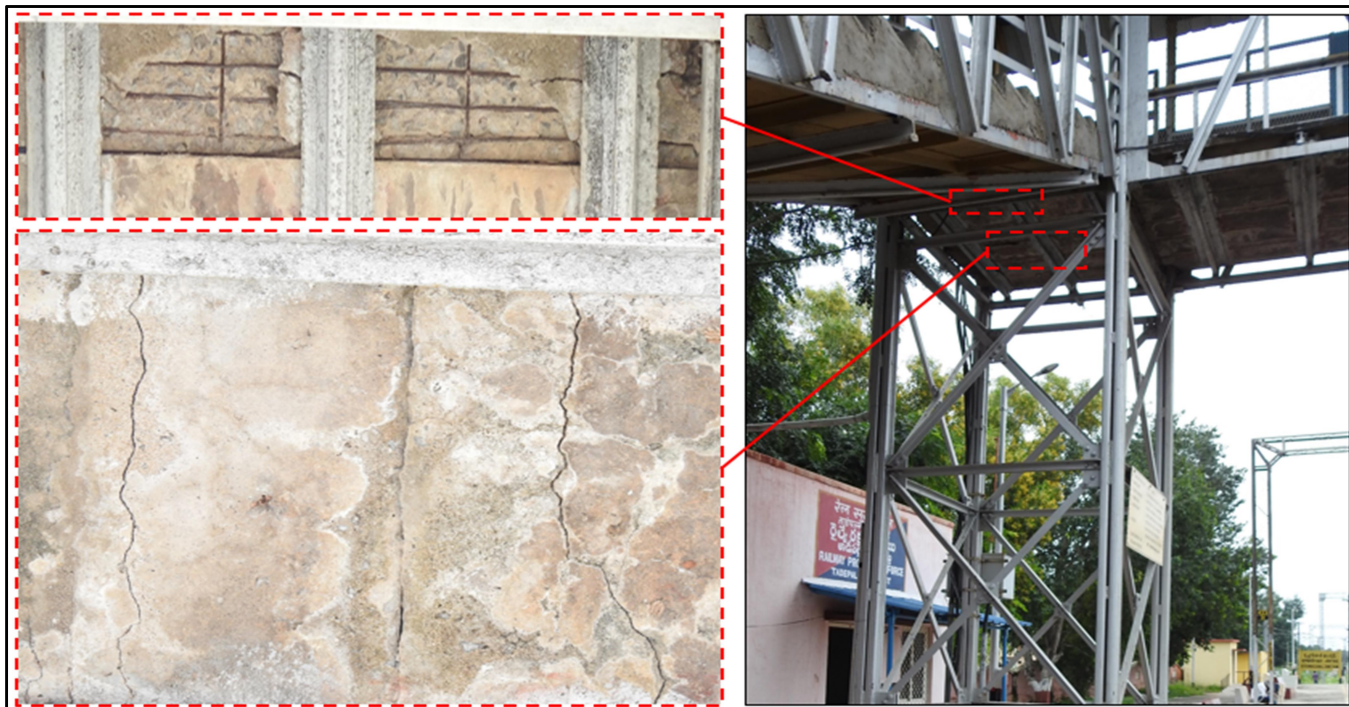
a) Exposed reinforcement and cracks on bottom of slab panels (Staircase 1 Main landing)
