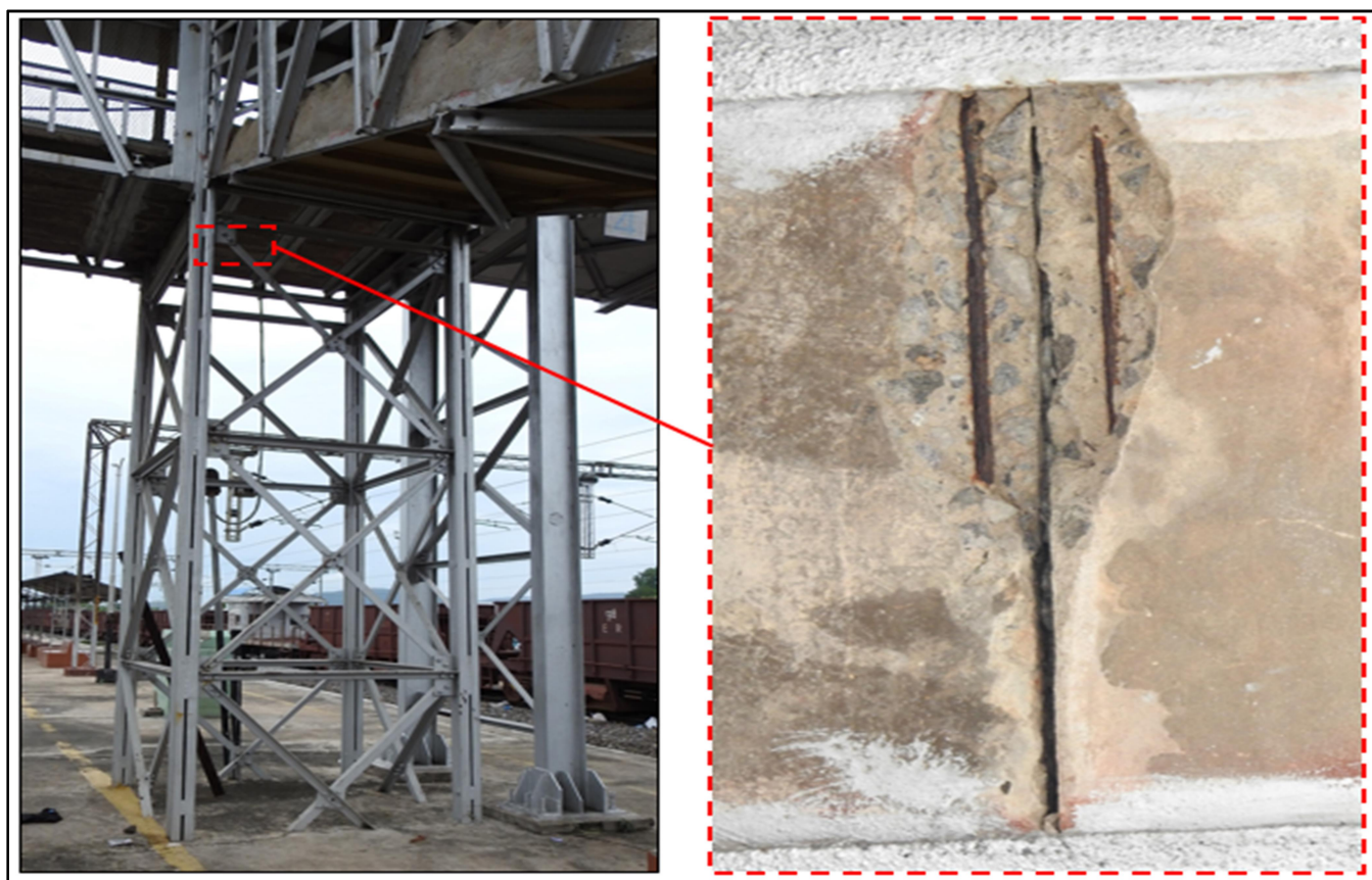
c) Exposed reinforcement on bottom of slab panels (Staircase 3 - Main landing)
