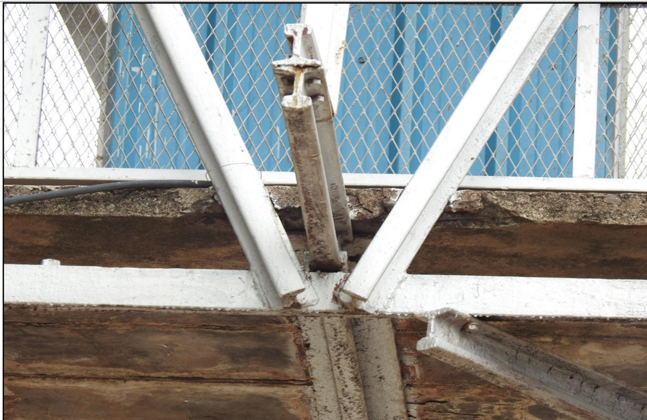
g) Rusting observed at Floor beam and bottom chord
