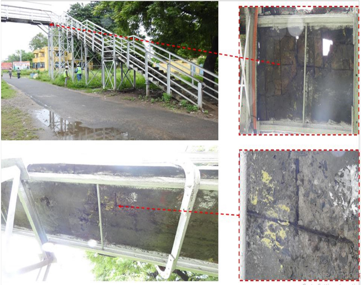
a) Reinforcement exposed & broken slab panels
