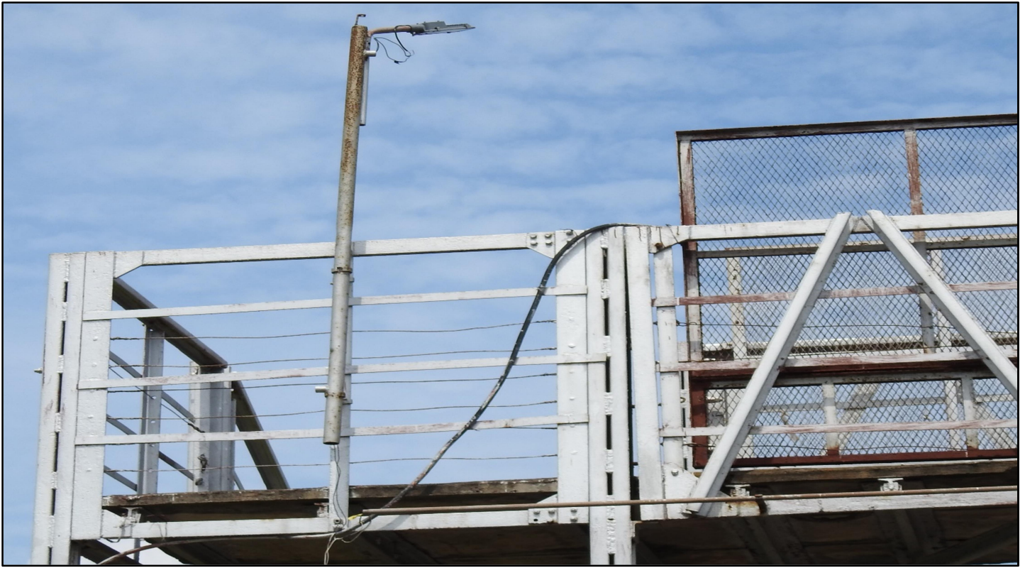
Fig 1: Cables, Electric post and protective screen
