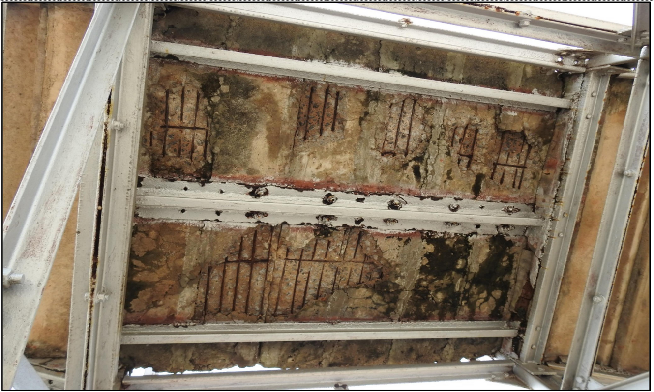
e) Severe Spalling, Reinforcement visible in staircase 2 (Mid landing)
