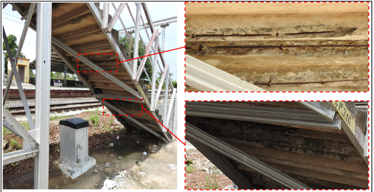
d) Reinforcement exposed slab panels on bottom of staircase-2
