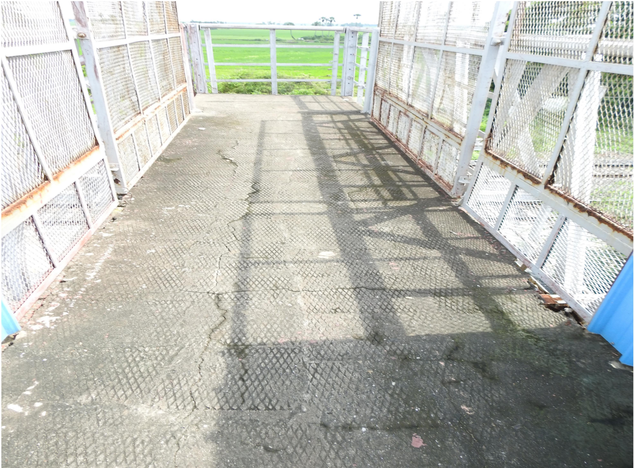
Fig 8: path way, Protective screen
