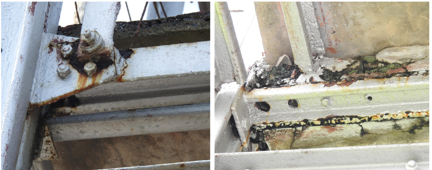
Fig 7: Corrosion is also observed at steel concrete joint gusset plate
