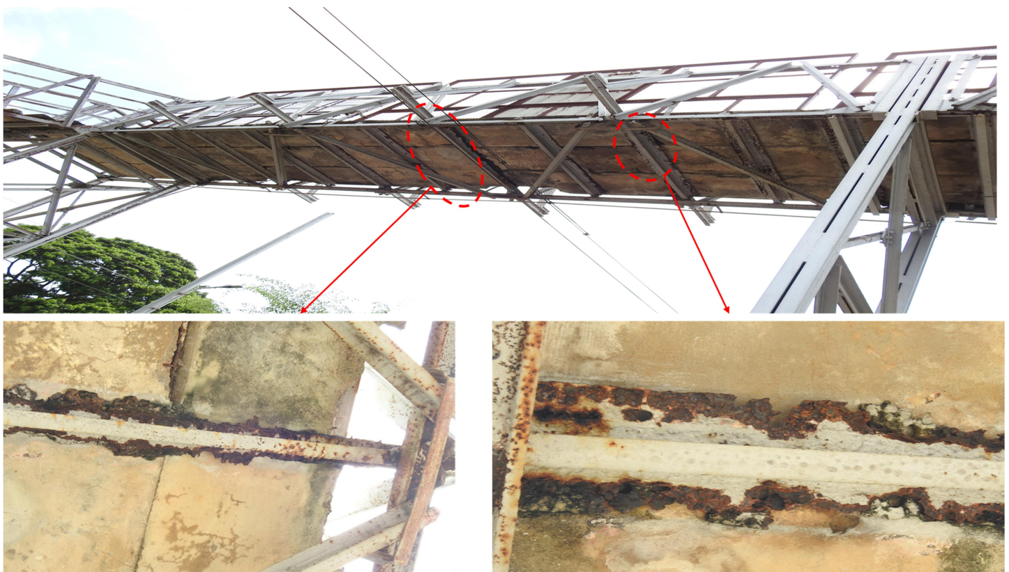
b) Corrosion of Floor beams is observed in 2 nd span
