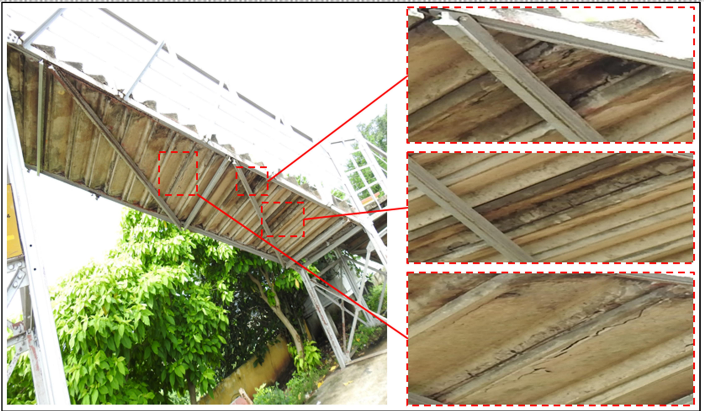
c) Reinforcement exposed slab panels on bottom of staircase-1
