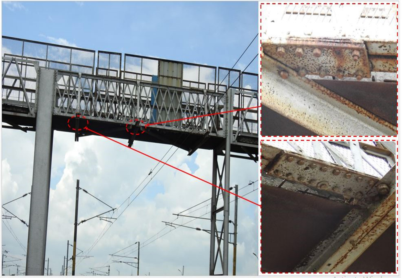
b) Rusting And corrosion At Span-2
