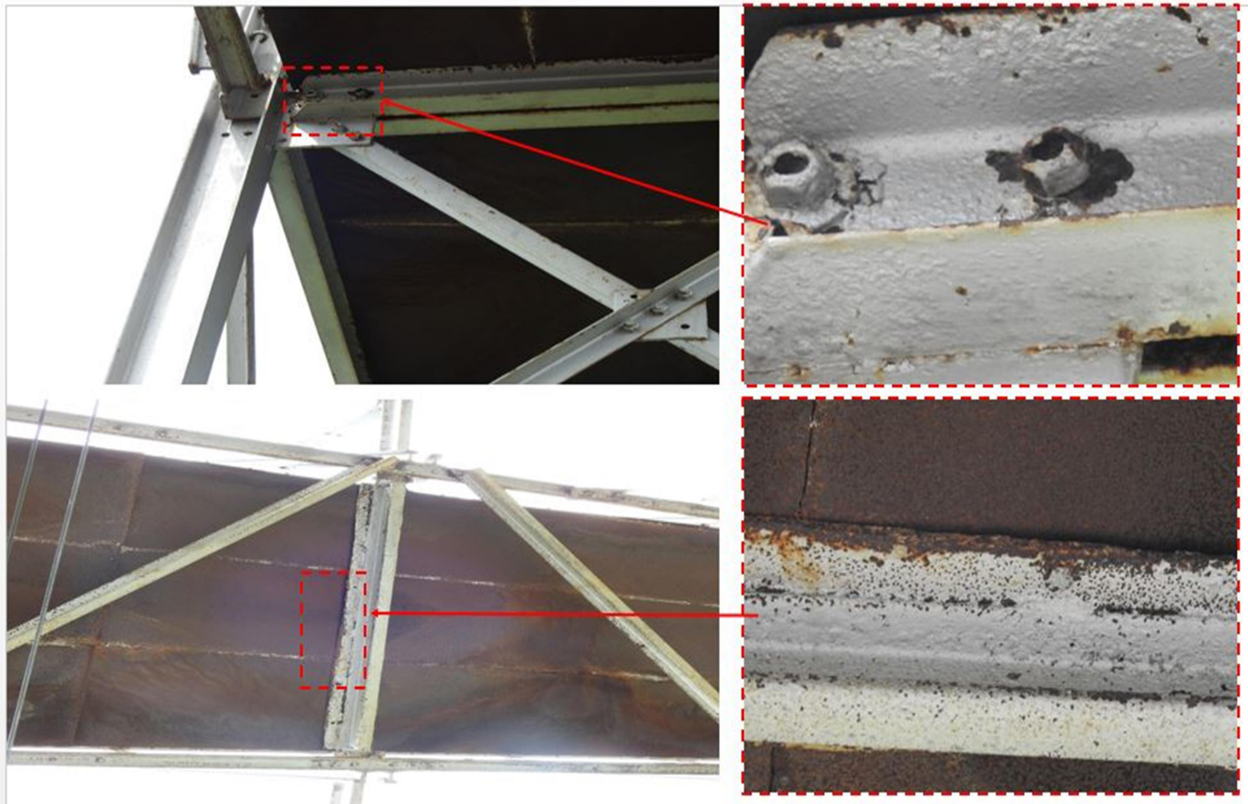
f) Corrosion at connections and Floor Beam
