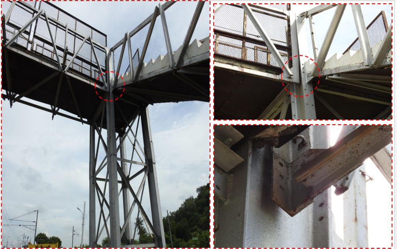
3 Bolts missing and gap of 2" formed in connection between Truss and Trestle-2
