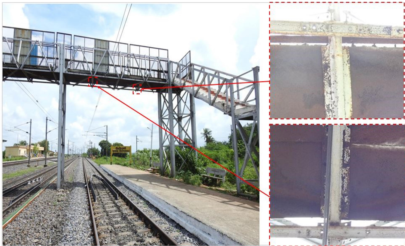
a) Rusting and Corrosion At Span-1
