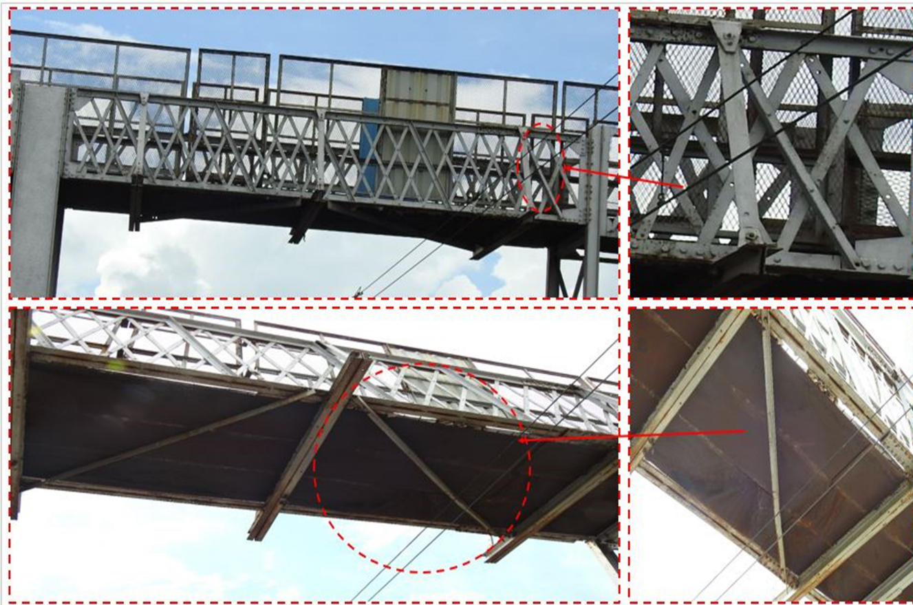
Deformation in Diagonal members and Bottom bracing
