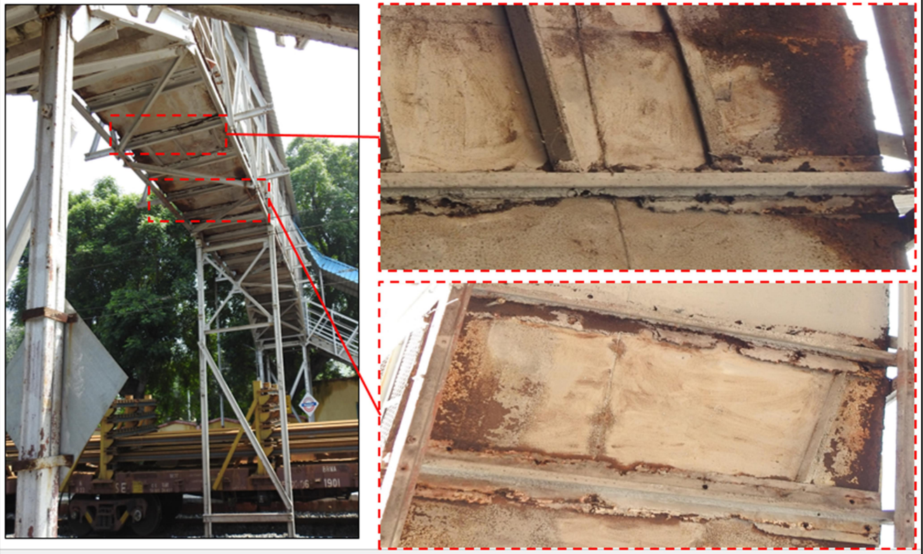
a) Corrosion observed at floor beams on Span-2
