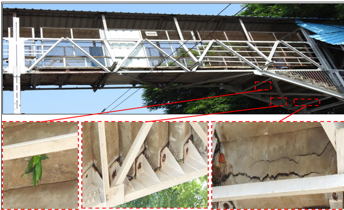
b) Vegetation, corrosion at cleat angles and cracks observed at staircase Span 1
