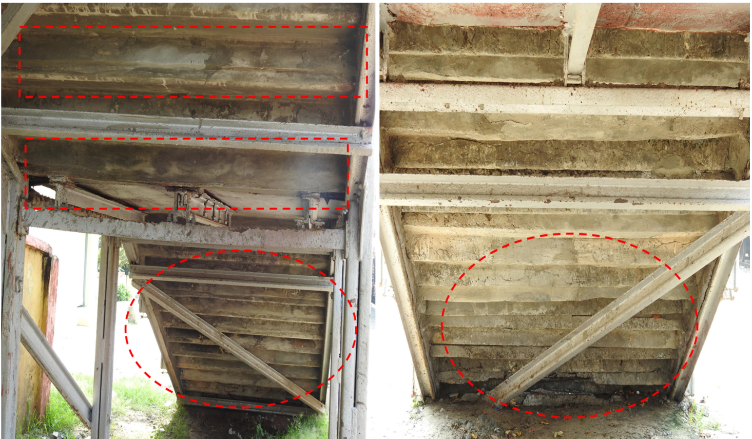
Fig 5: Patch work is observed at PF- 2 stair case steps
