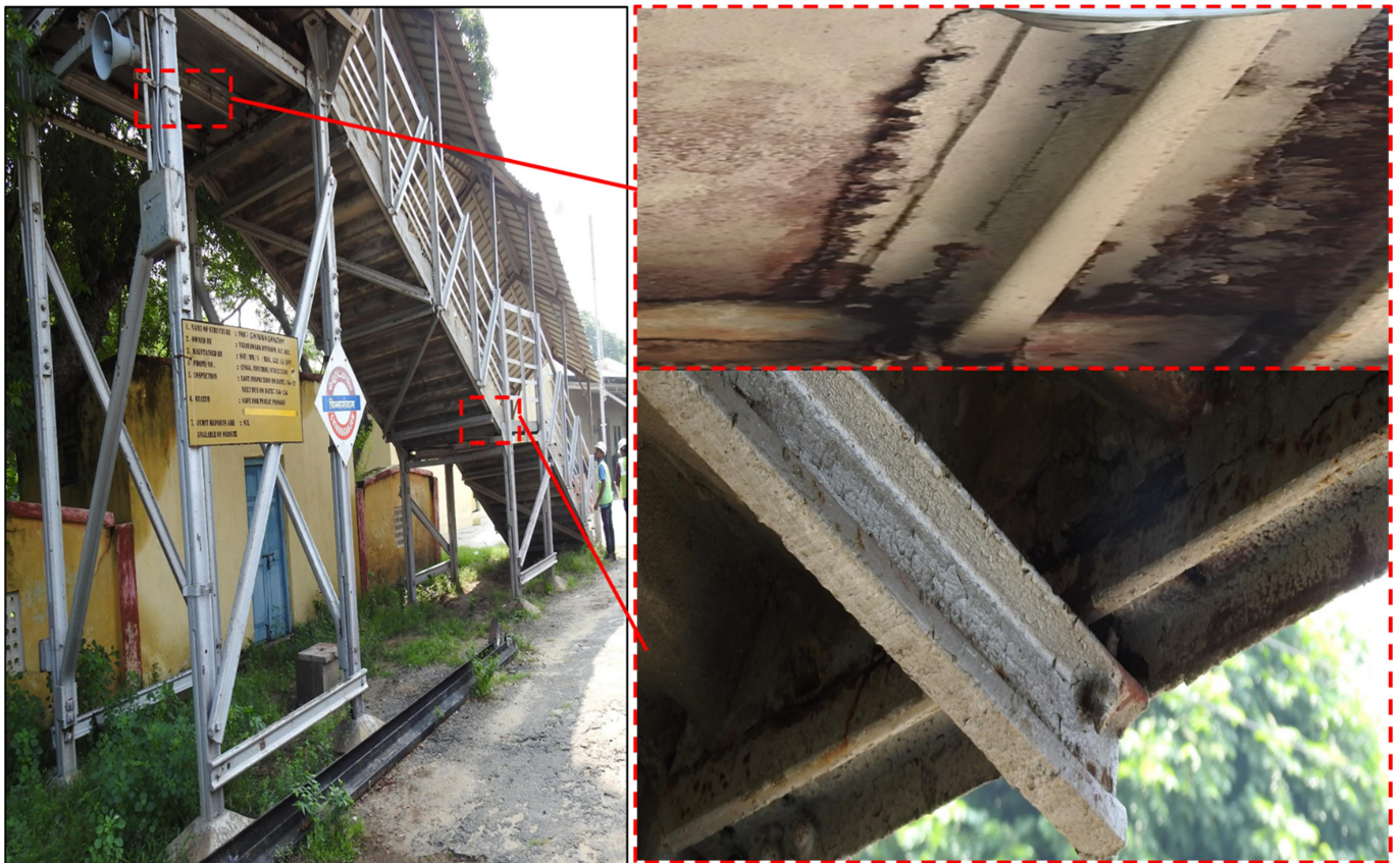
b) Corrosion observed at floor beams in landing and Stringer beams in Staircase 1
