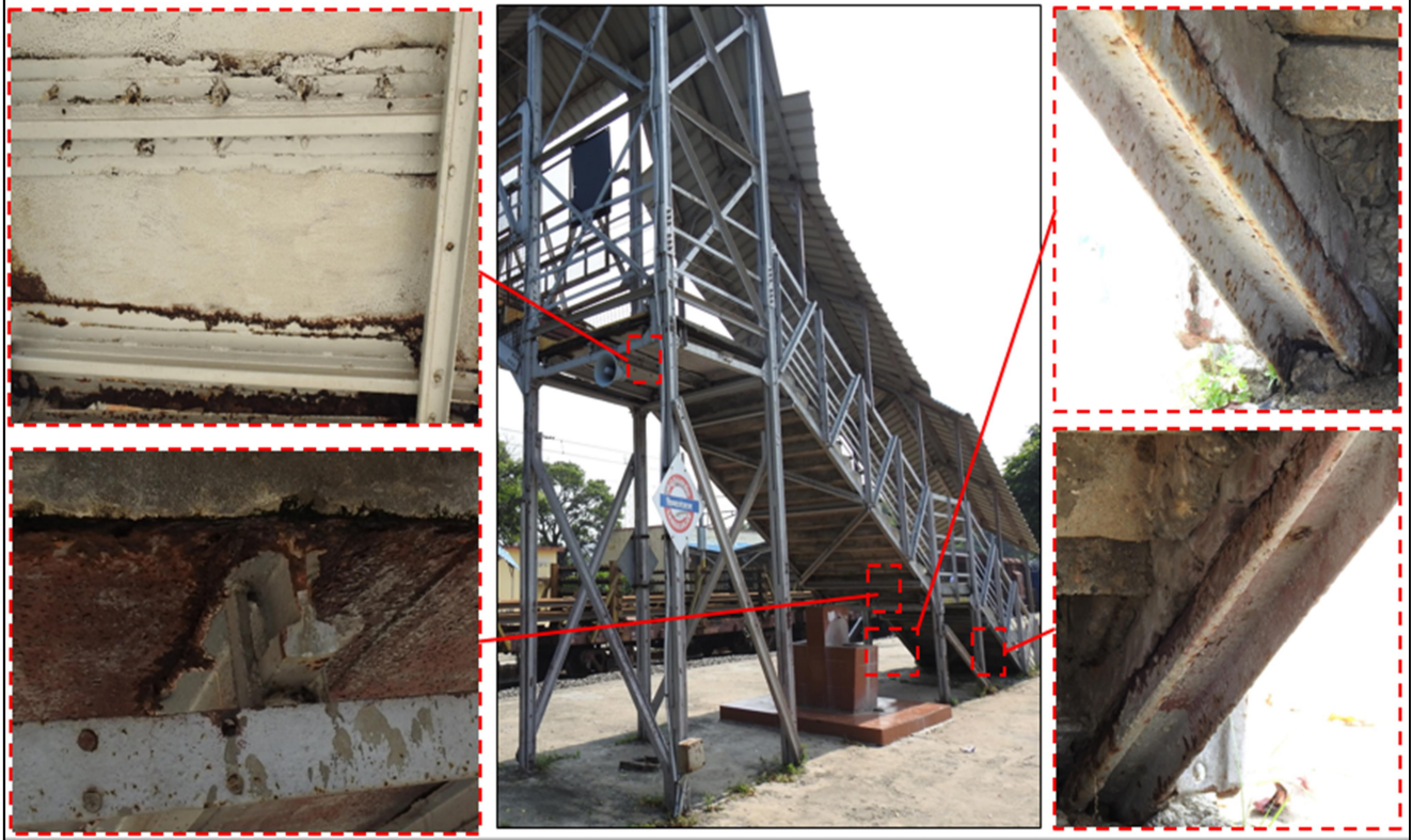
c) Corrosion observed at floor beams in landing and Stringer beams in Staircase 2
