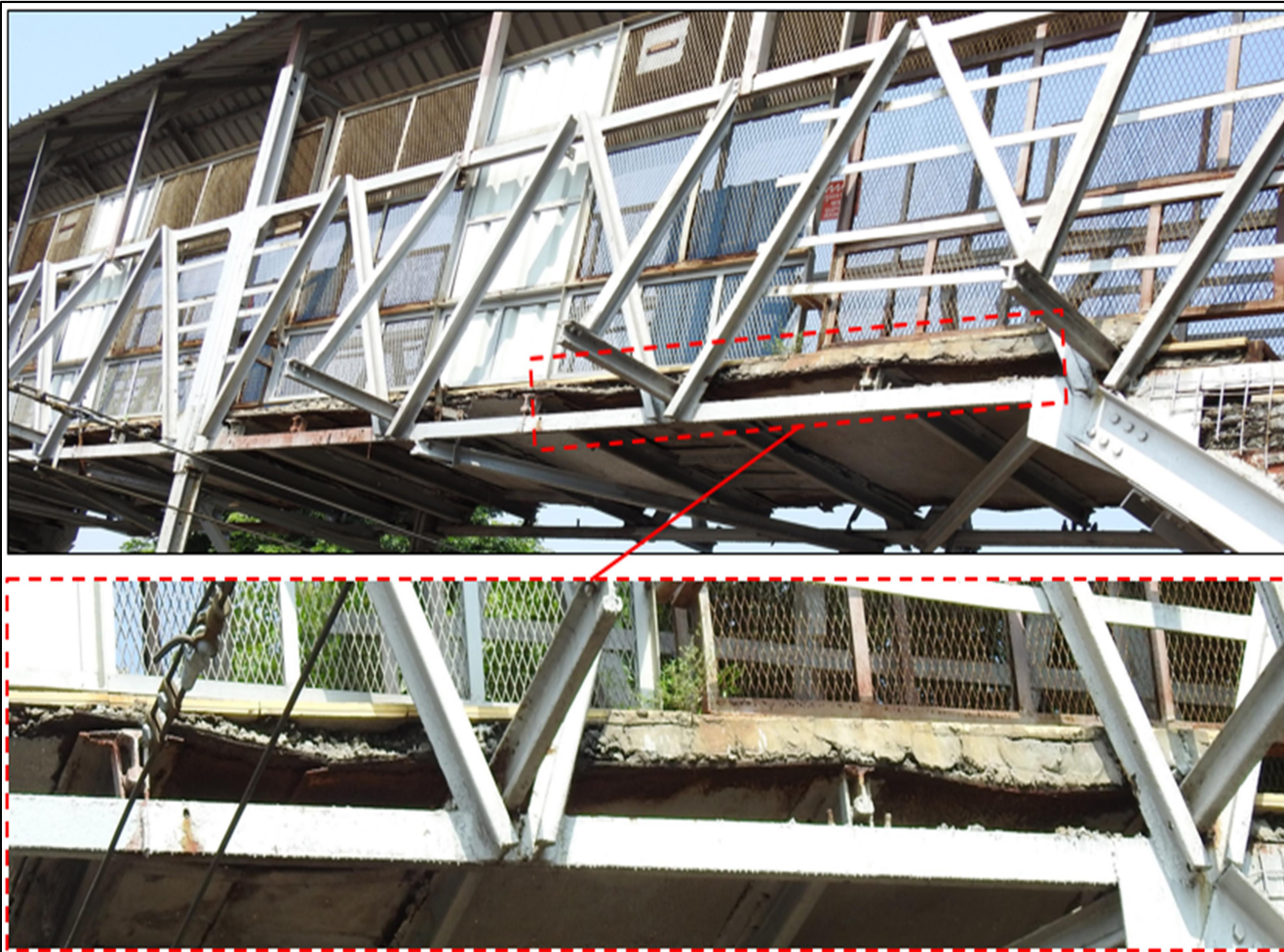
d) Deformation at slab panels on Span-1
