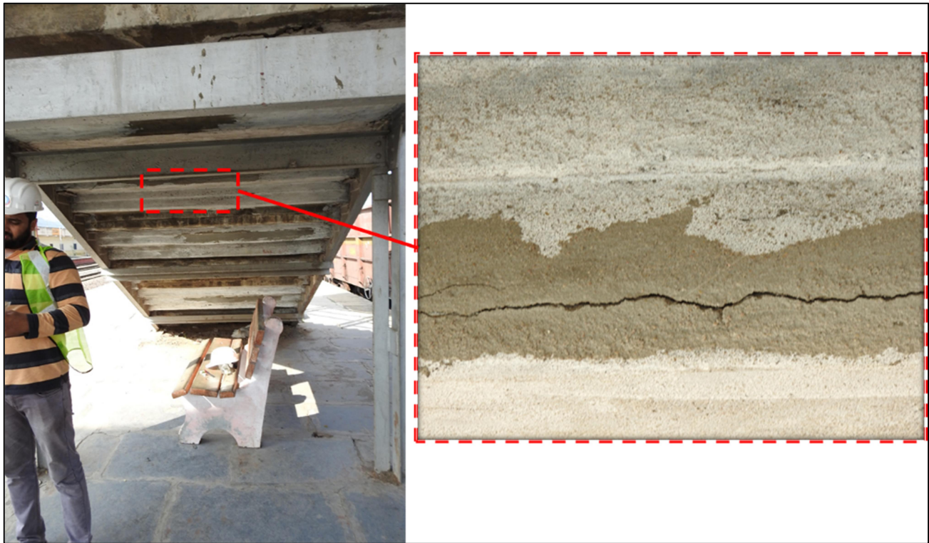
l) Cracks observed in staircase slab panels in staircase-3
