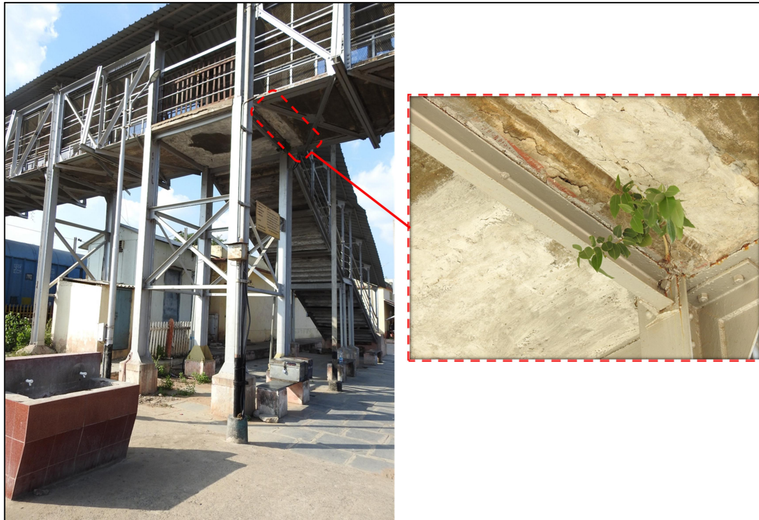
Fig 6: Cracks in slab and vegetation in staircase -2 of FOB
