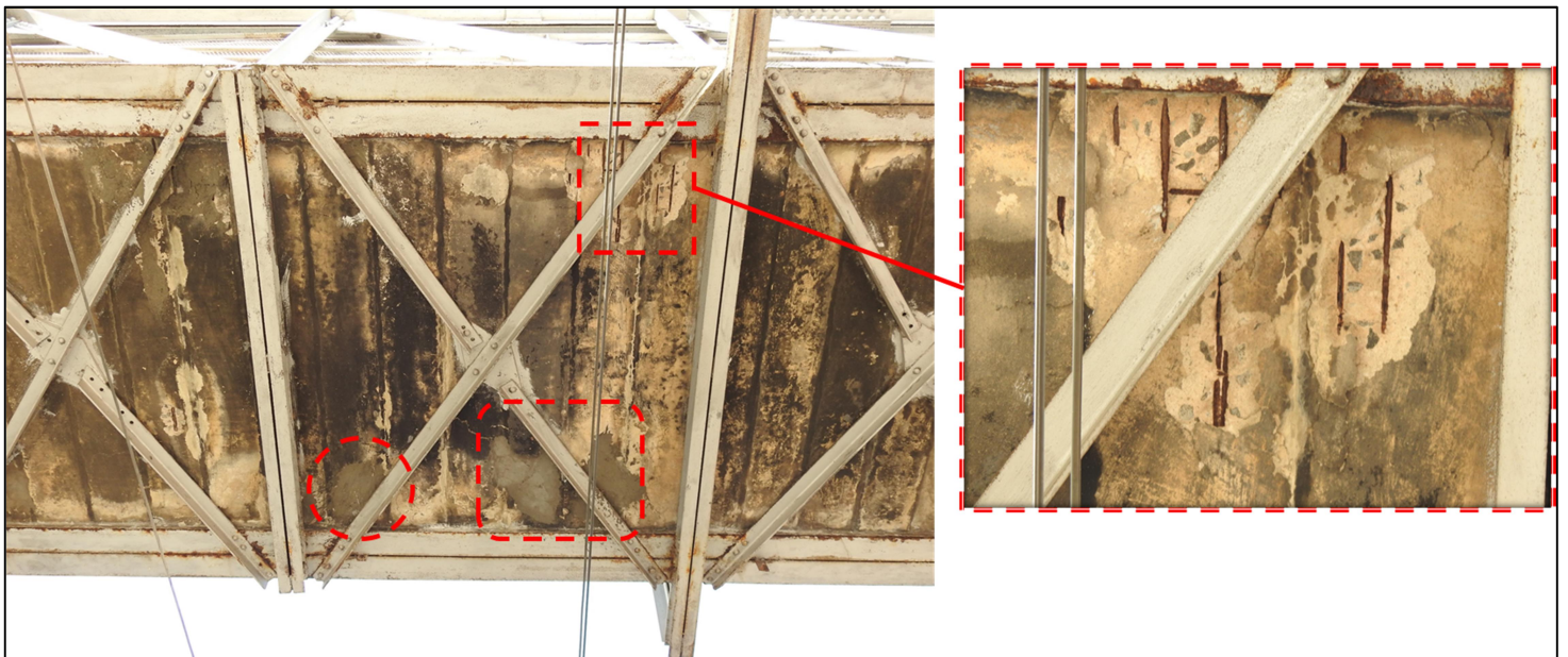
b) Reinforcement exposed slab and patch work 3 rd span of FOB
