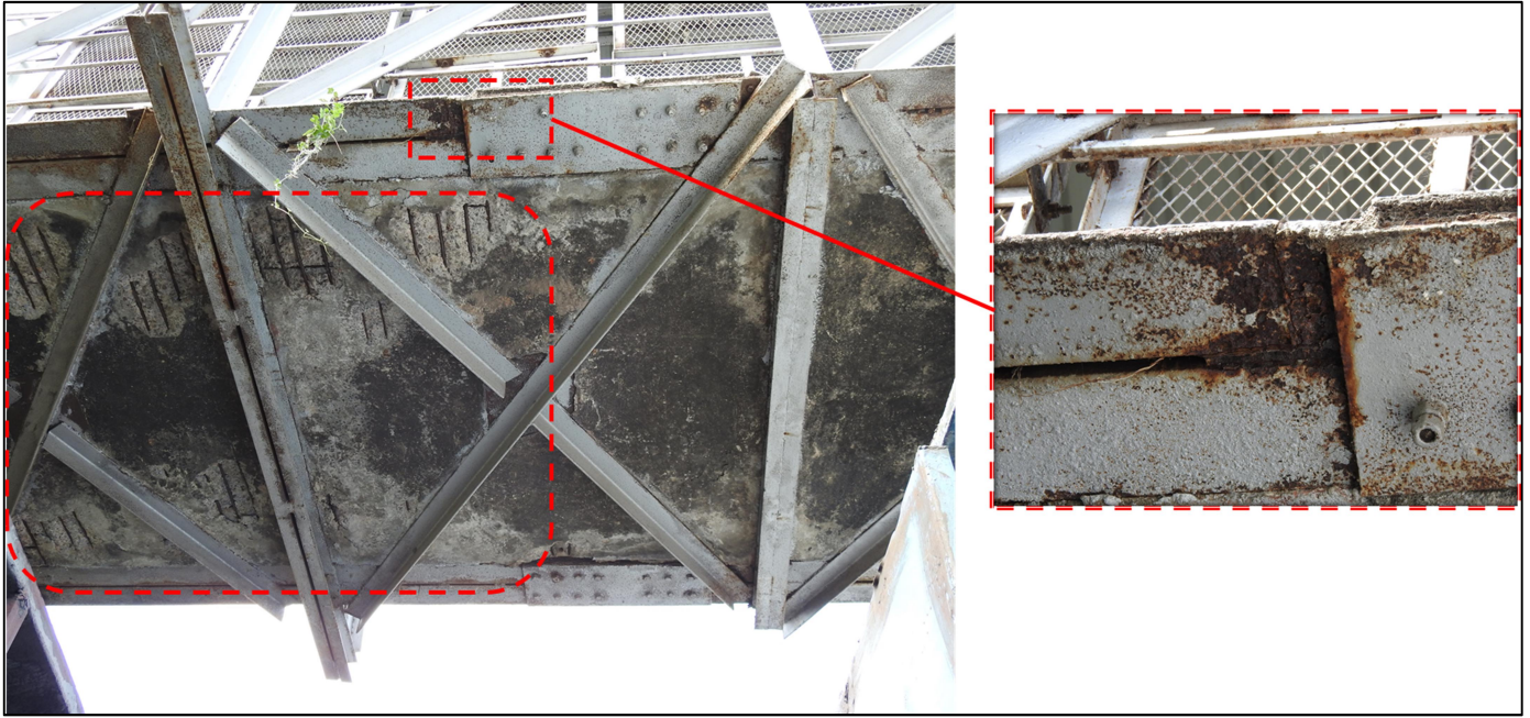
c) Reinforcement exposed slab and corrosion in 1 st span of FOB
