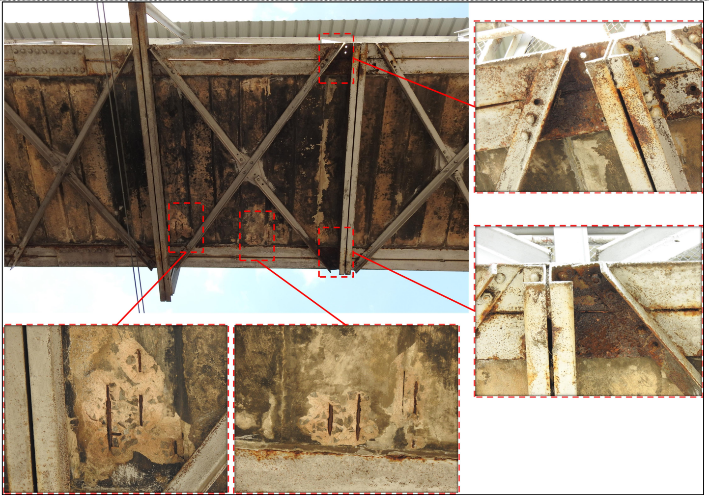
a) Reinforcement exposed slab and corrosion in 3 rd span of FOB
