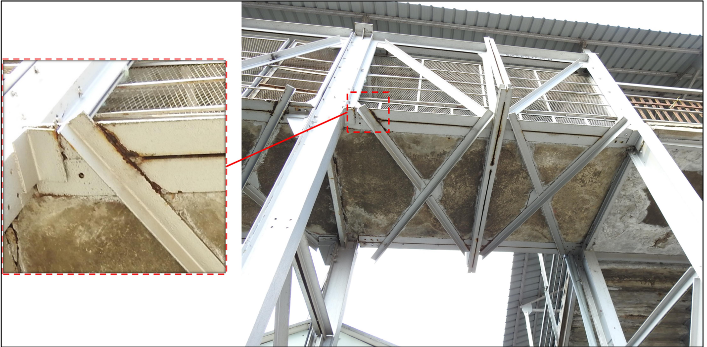
i) Corrosion of gusset plate connected bottom bracing in 2 nd span of FOB
