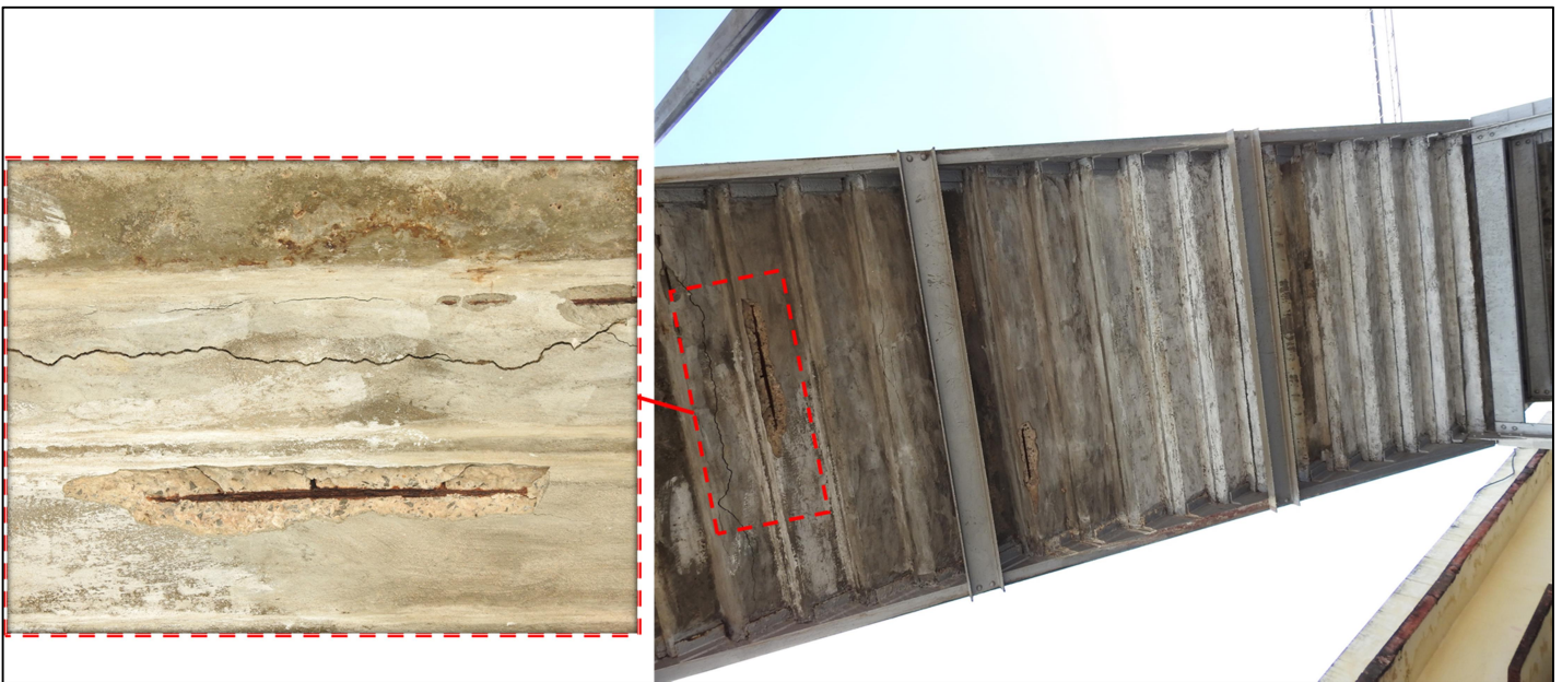
j) Cracks and reinforcement exposed in staircase slab panels in staircase -2
