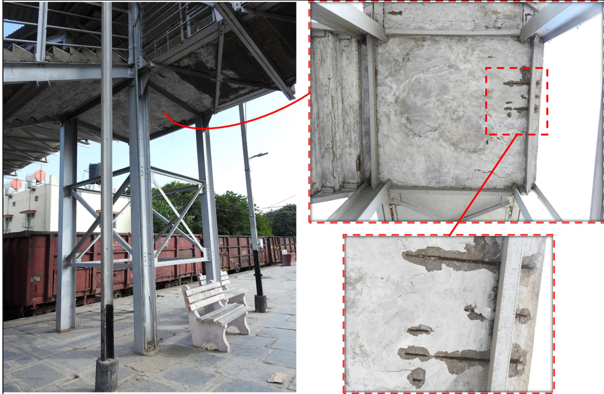
g) Reinforcement exposed slab in landing in 3 rd span of FOB
