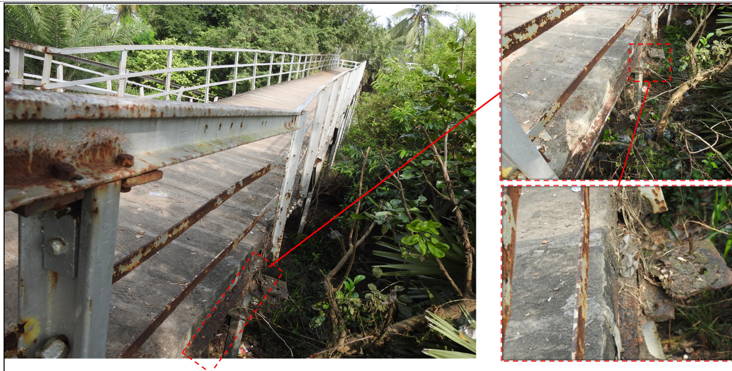
g) Corrosion of ramp landing beam
