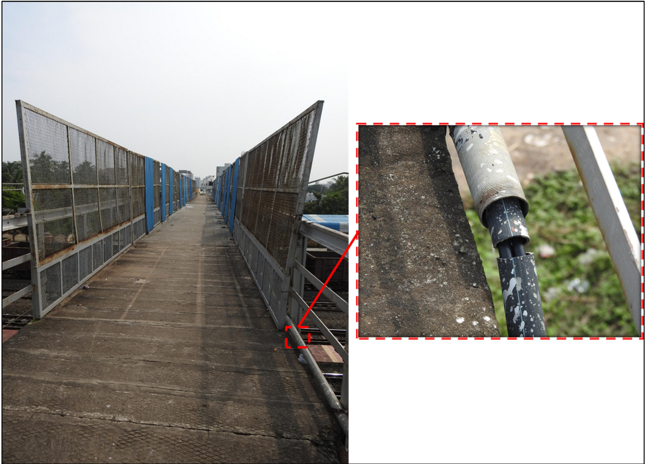
Fig 2: FOB pathway, protective screen and cables on floor of pathway
