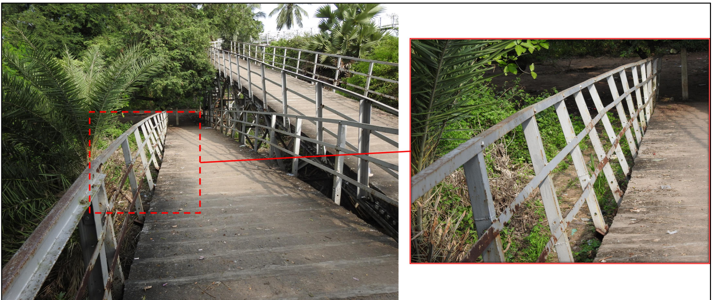
Fig 6: Damaged ramp railing
