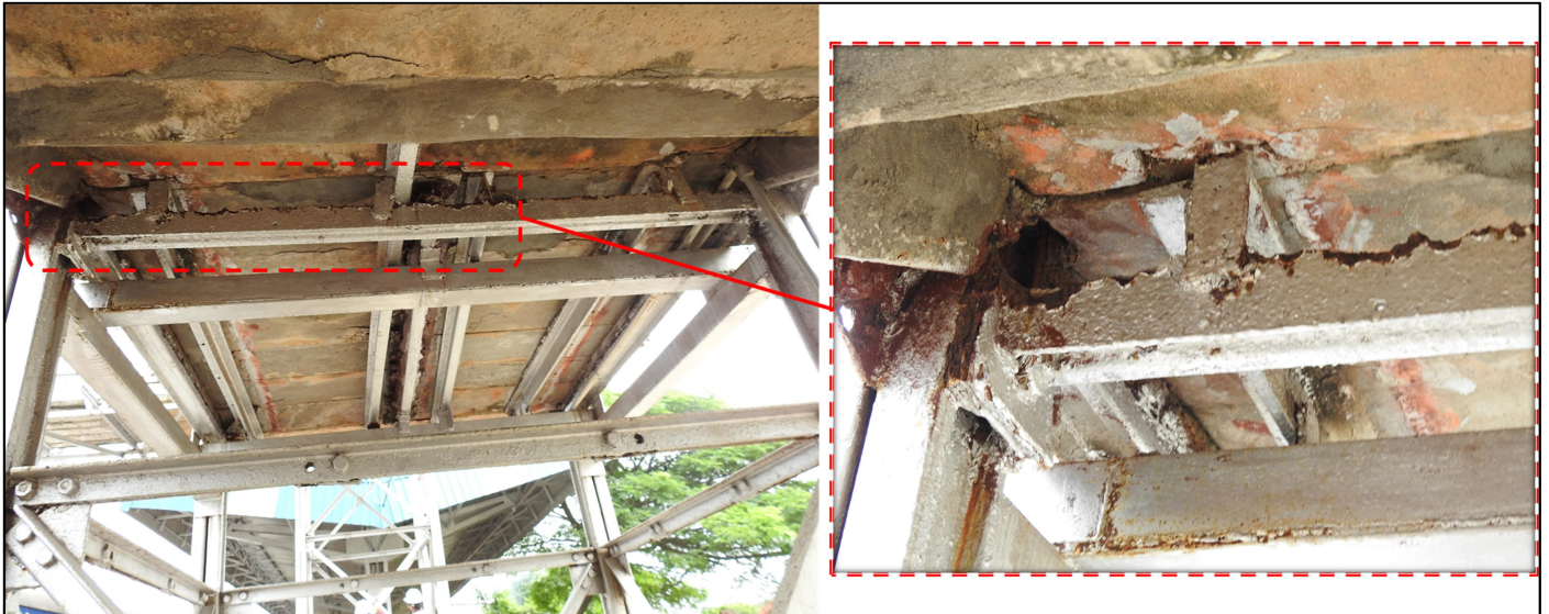
(c) Corroded angle section in staircase -1
