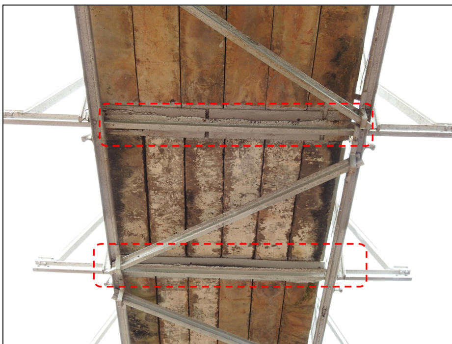
Corrosion of Floor beam coated with silver oxide paint
