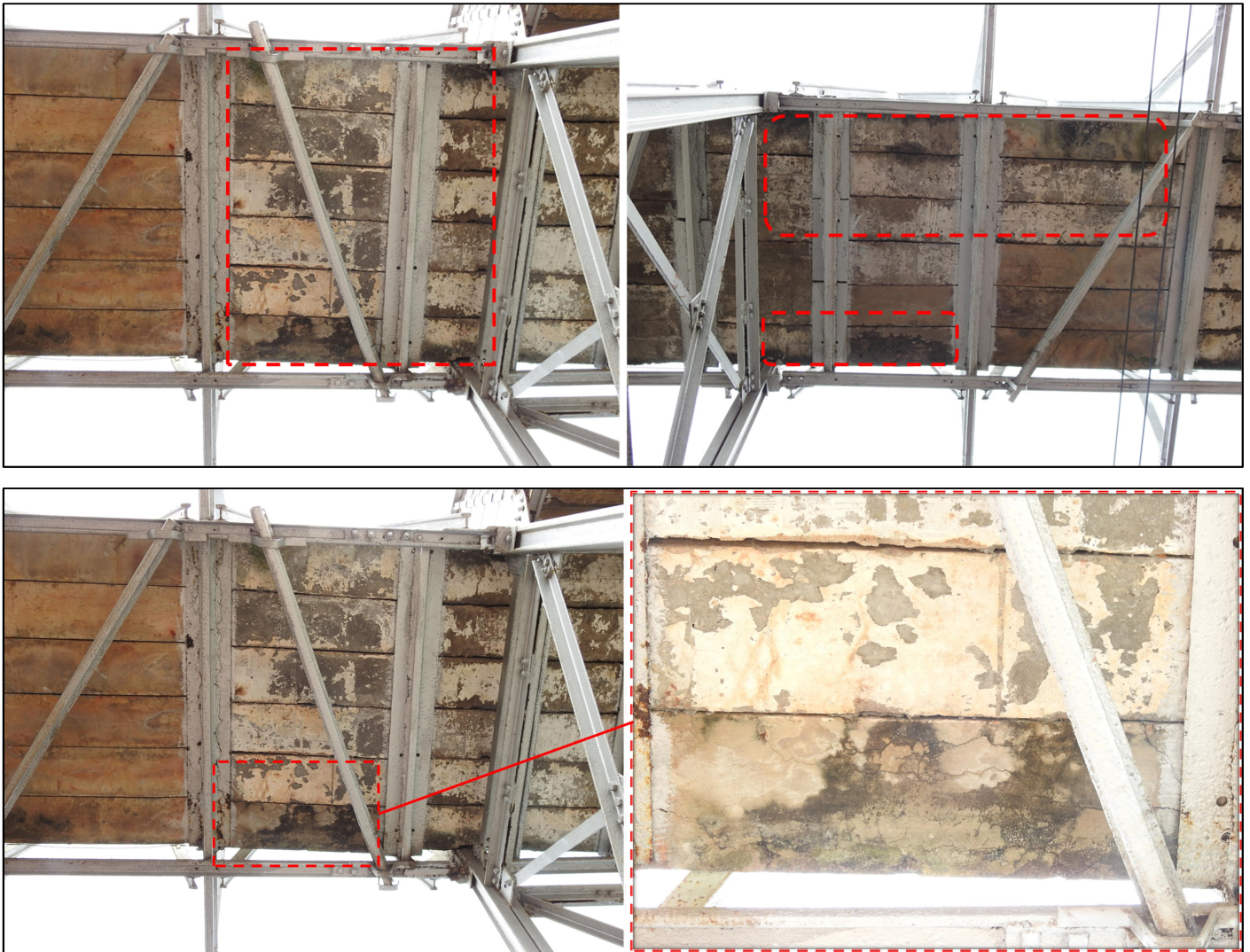
(a) Leaching and cracks in slab panels
