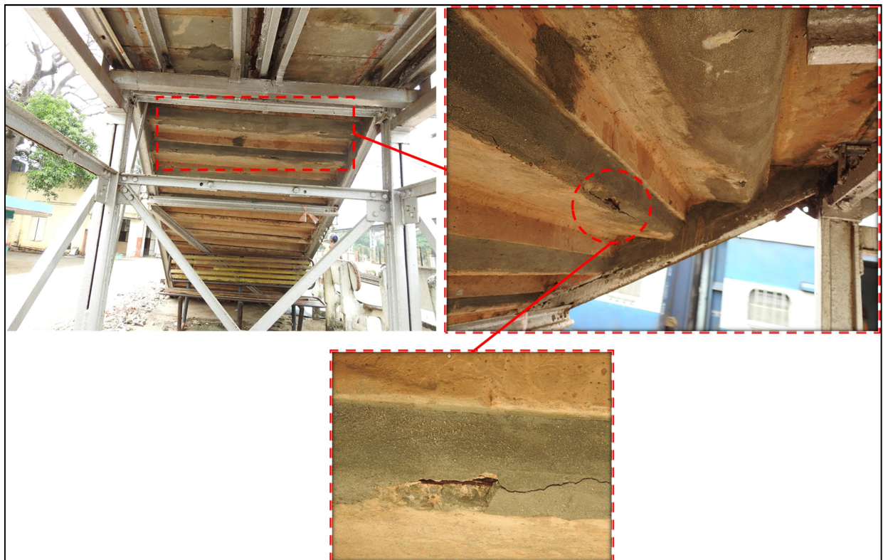
Fig 7: Patch work and reinforcement exposed in staircase -1
