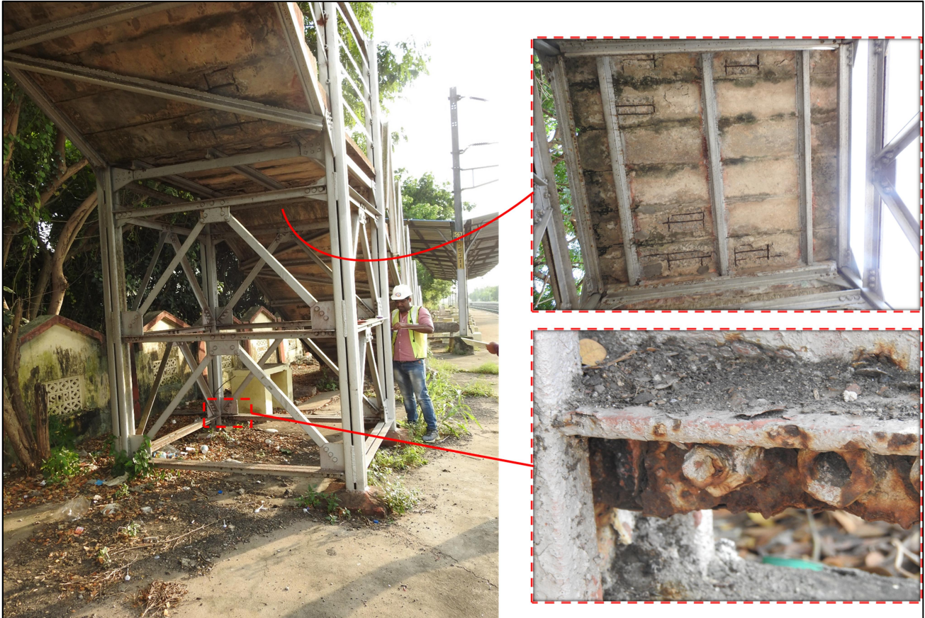
a) Exposed reinforcement and spalling in staircase-2 landing
