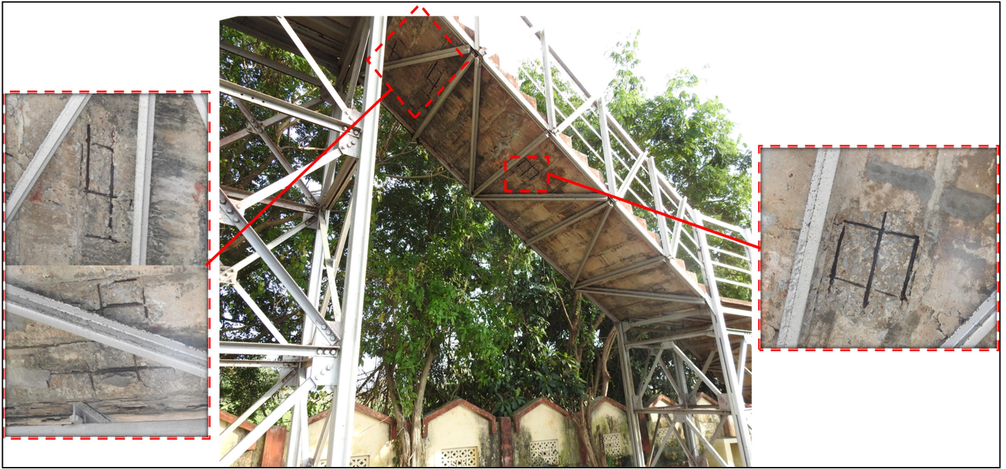
c) Exposed Reinforcement in staircase
