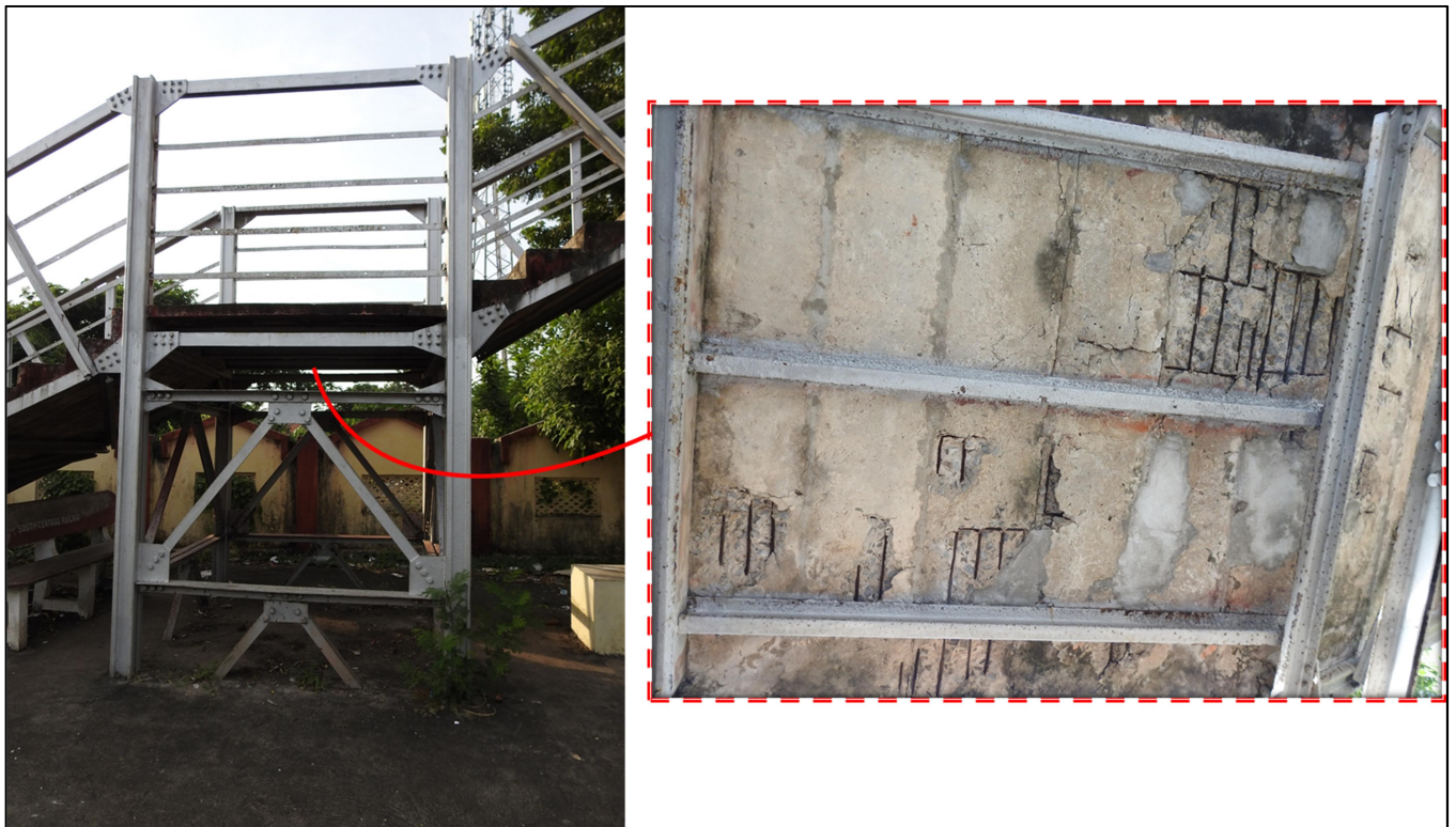
b) Exposed reinforcement and spalling in staircase-1 landing
