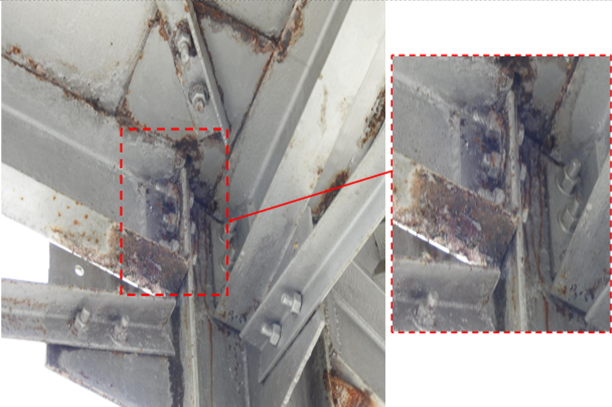
a) Corrosion observed at Stringer beam joint of Span-1
