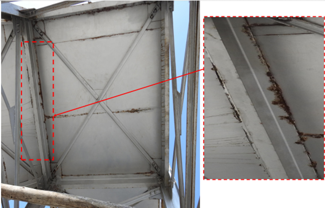
c) Rusting observed at landing of Staircase-1
