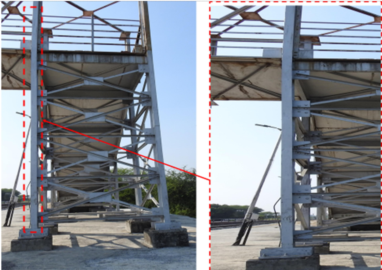
b) Deformation observed at Trestle 2
