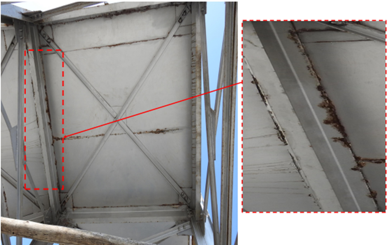
b) Corrosion observed at Main landing of floor beam in Span-1
