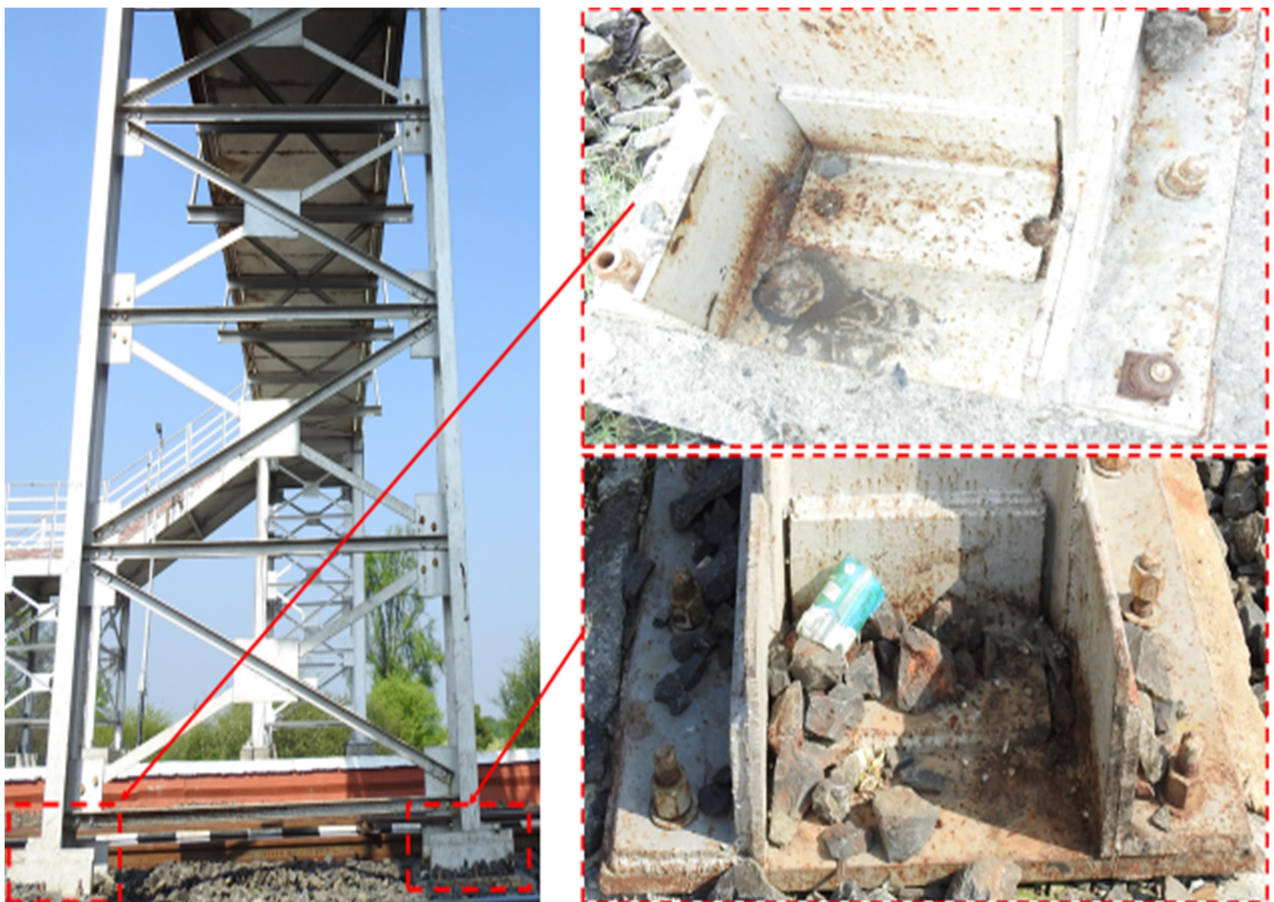
d) Rusting observed at base plate of stanchion
