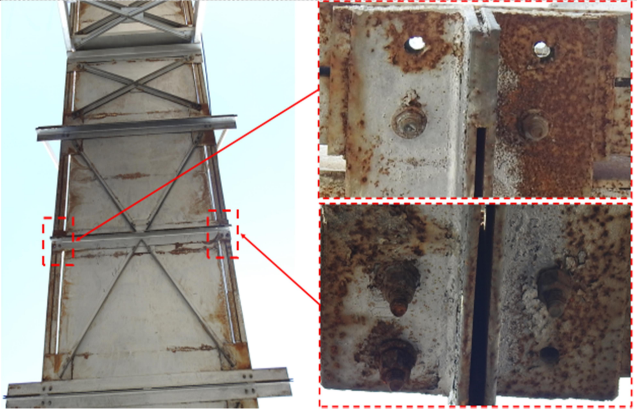
a) Missing bolts are observed at floor beam of Span-1
