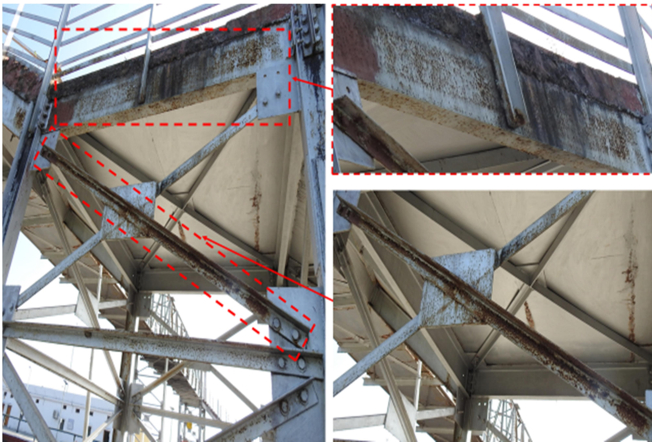
h) Rusting observed at stringer beam and landing in trestle-2
