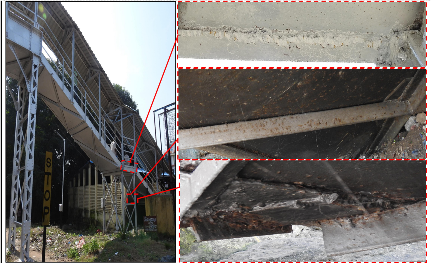
b) Corrosion observed at Staircase 2 Stringer beam and Rusting of cross bracing
