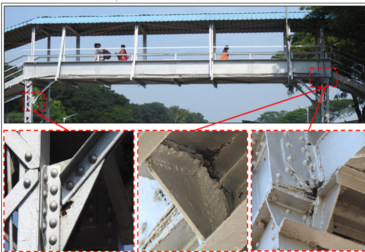
b) Corrosion observed at cleat angle connecting Stanchion and Stair and Gusset plates Joints
