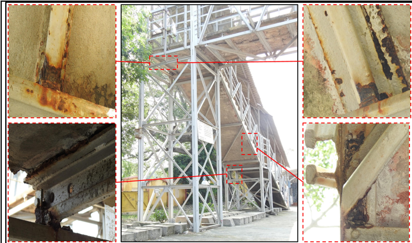
a) Corrosion observed at floor beams on staircase-1 Main landing and mid landing slab bottom
