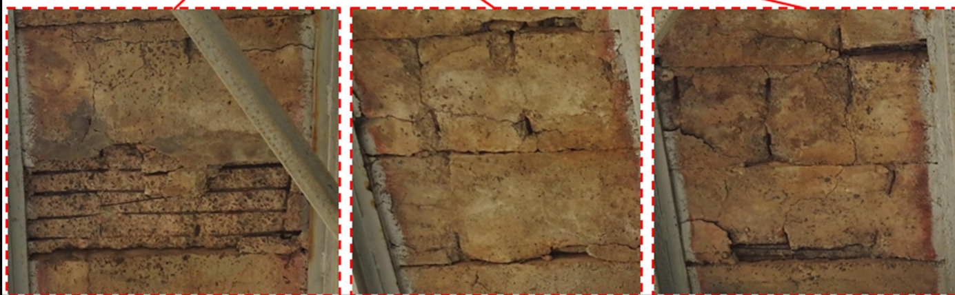
c) Reinforcement exposed and cracks observed on Span 1 slab bottom
