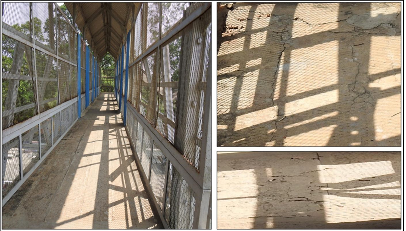
Fig 9: Cracks on top of Pathway Slab panels
