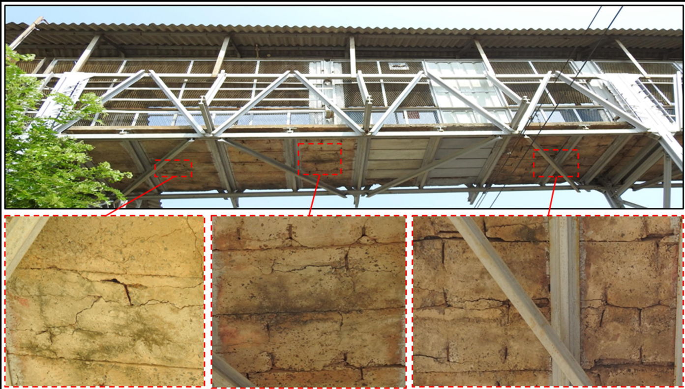
d) Reinforcement exposed , cracks and leaching observed on Span 2 slab bottom
