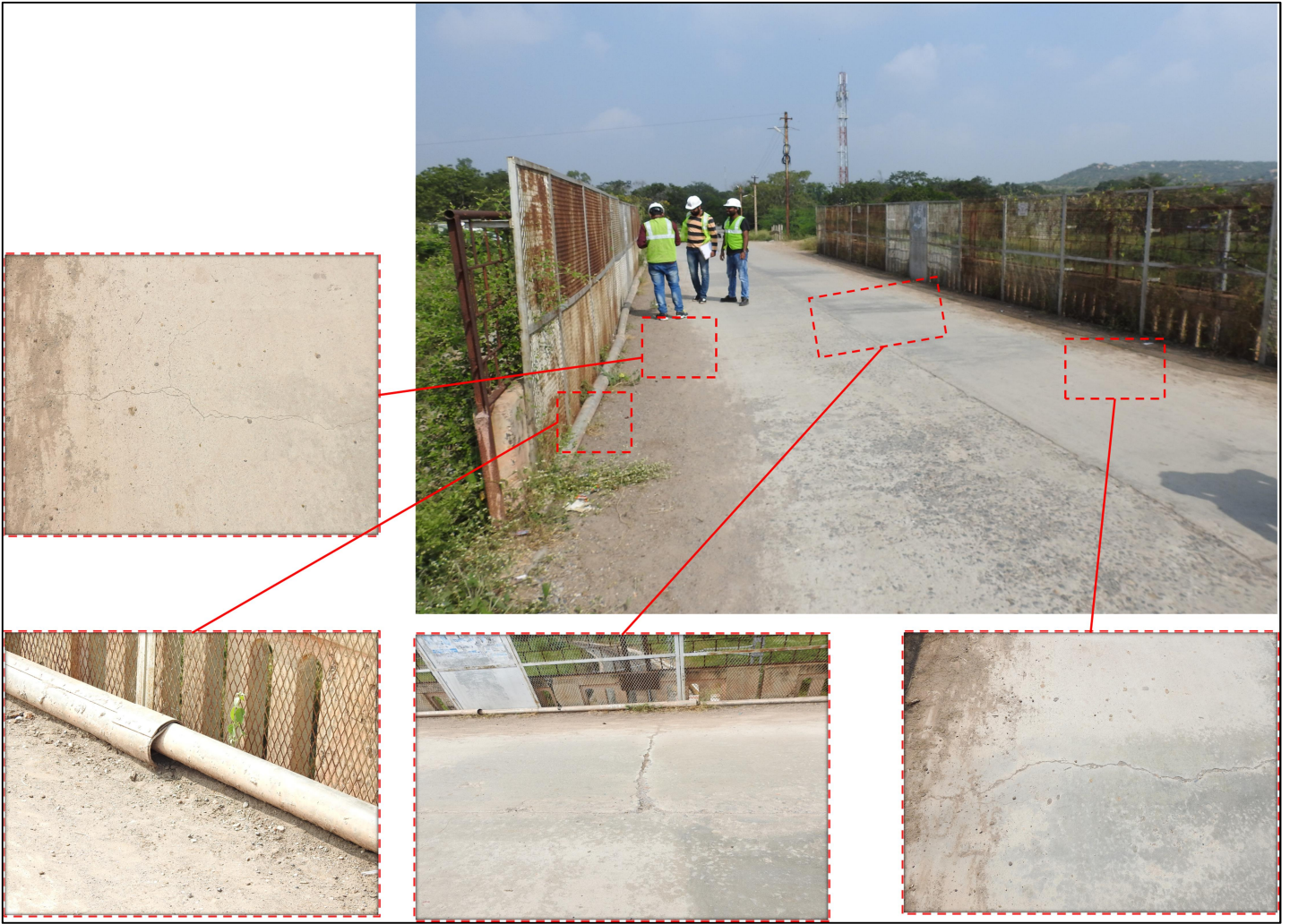
Fig 6: Utility services passing on the Bridge and Wearing Coat condition
