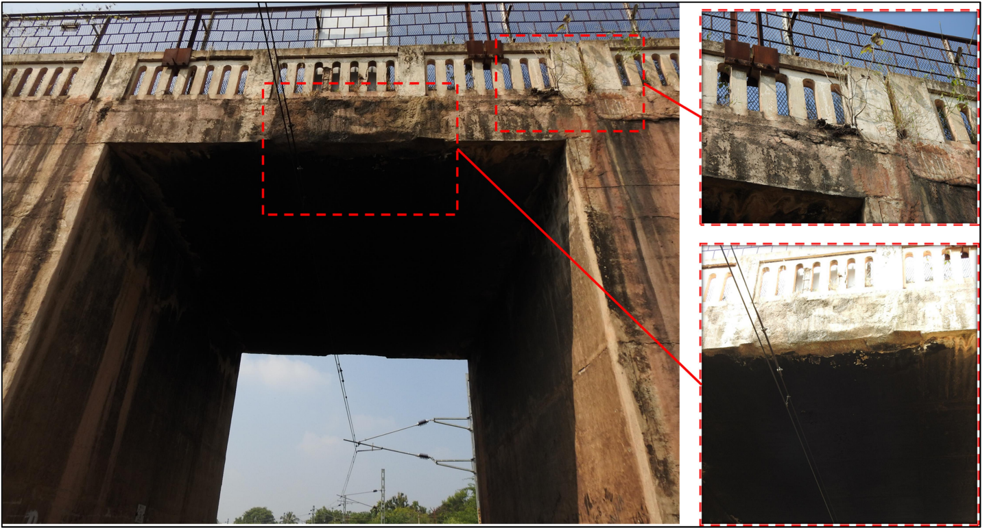
Fig 4: Chipped surface of slab bottom above OHE cable on both sides of ROB and vegetation at railing
