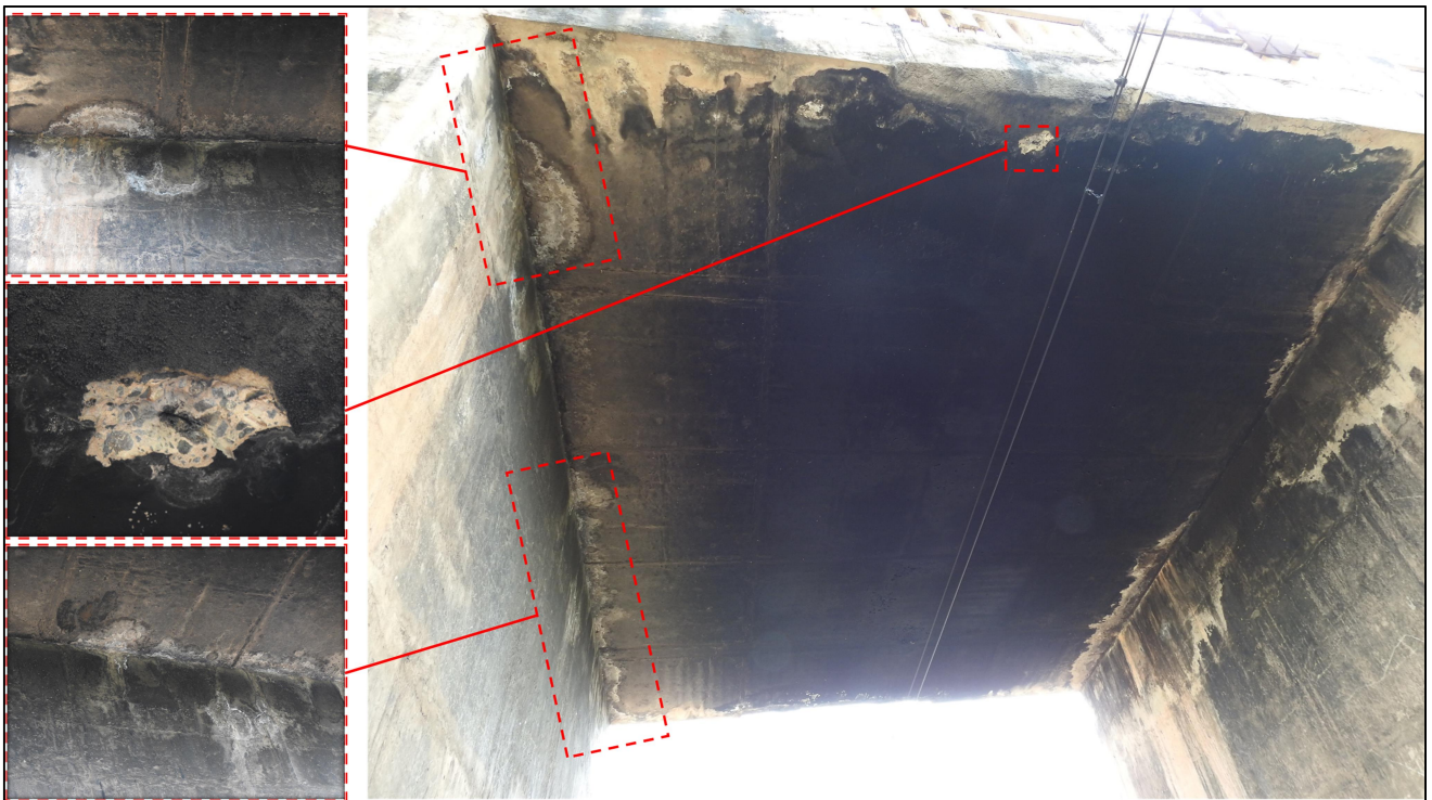
Fig 5(a): Leaching and slight spalling in slab
