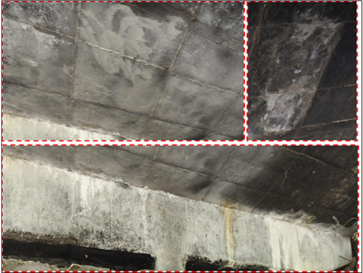
Fig: 11 Leaching observed at slab of Span-1
