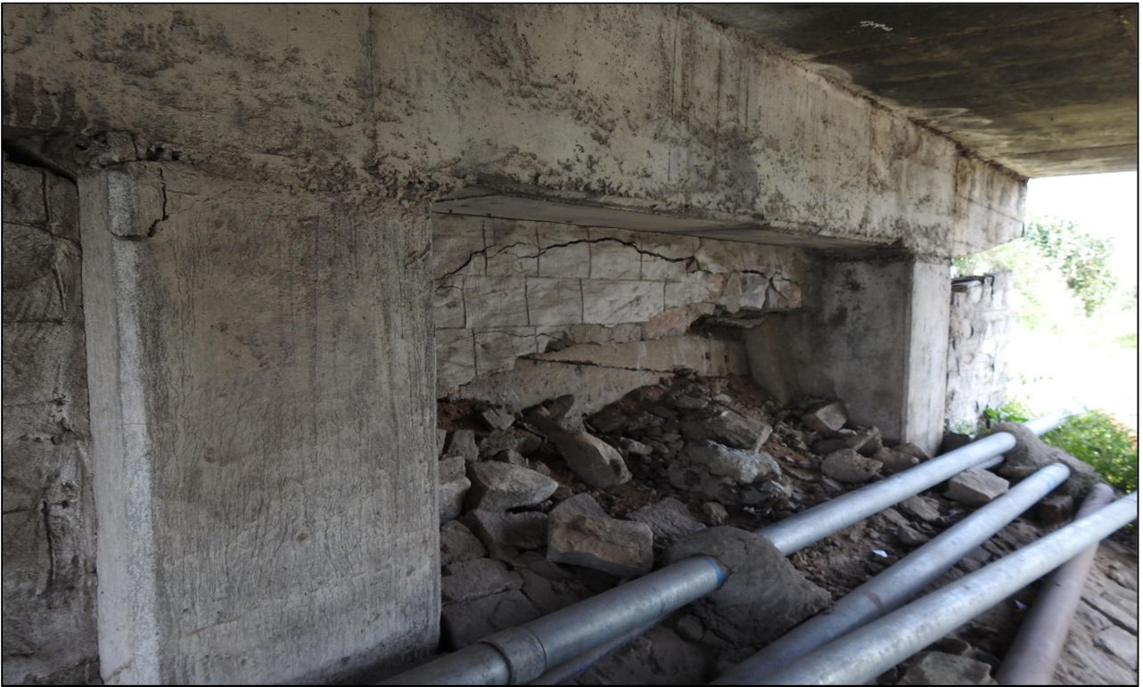
Fig: 18 Retaining wall damaged at Abutment-2
