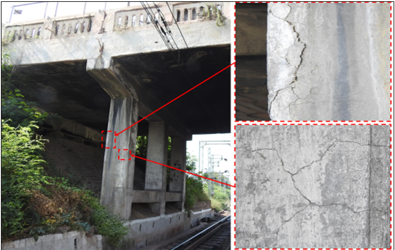
Fig: 8 Spalling and Cracks observed at Pier-4
