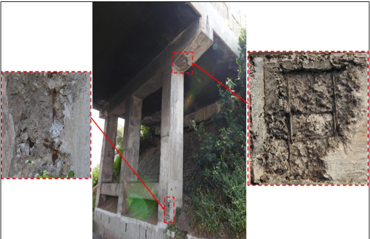
Fig: 5 Reinforcement Exposure observed at Pier-1
