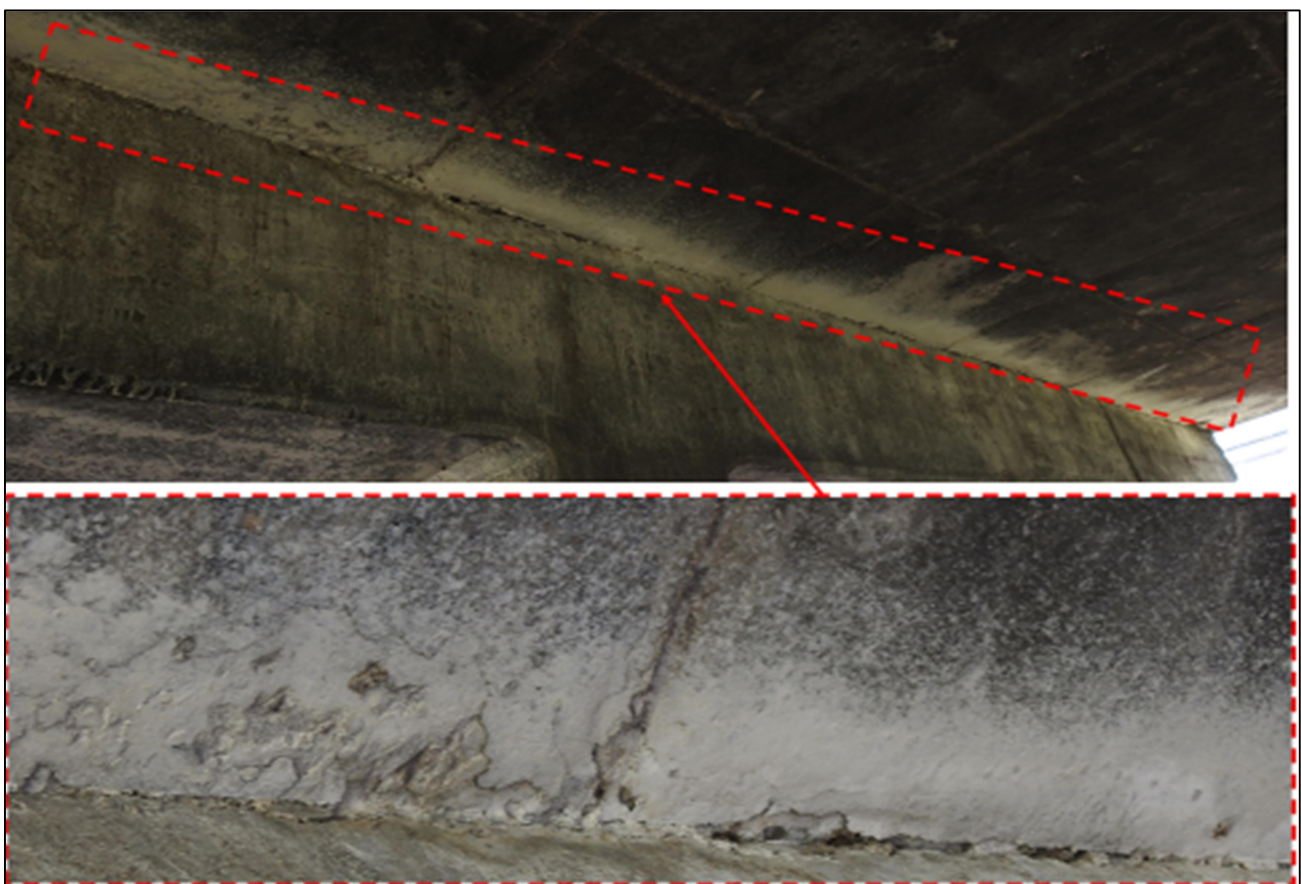
Fig: 15 Leaching observed at slab of Span-5
