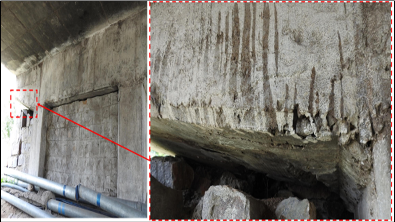
Fig: 4 Deterioration of cantilever portion of bedblock observed at Abutment -2
