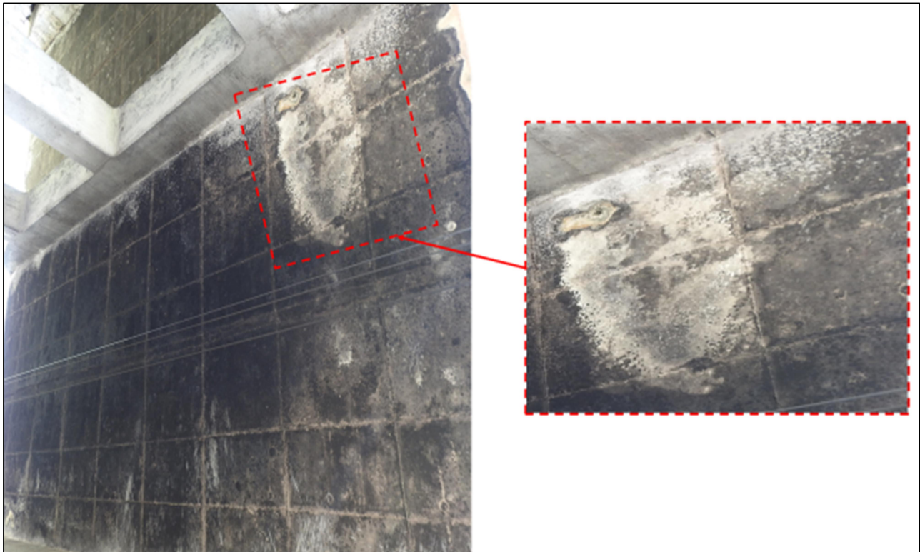
Fig: 14 Leaching observed at slab of Span-4
