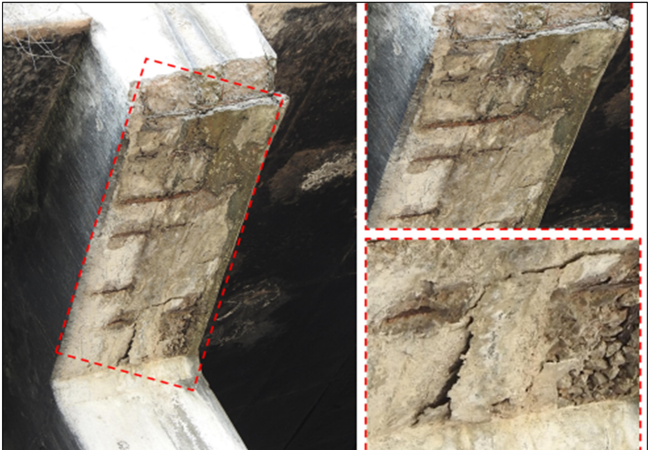
Fig: 9 Reinforcement exposure & Spalling observed at Pier cap-4
