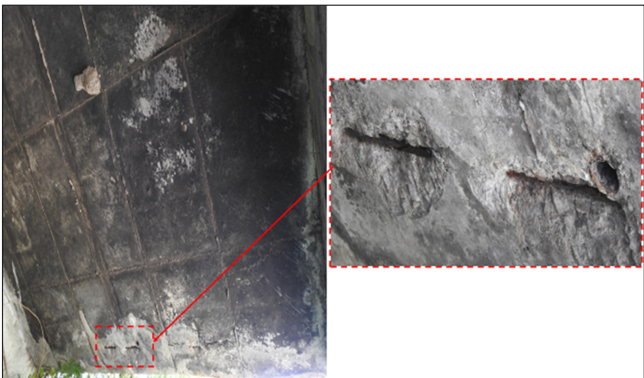
Fig: 10 Reinforcement exposure observed at Slab of Span-1
