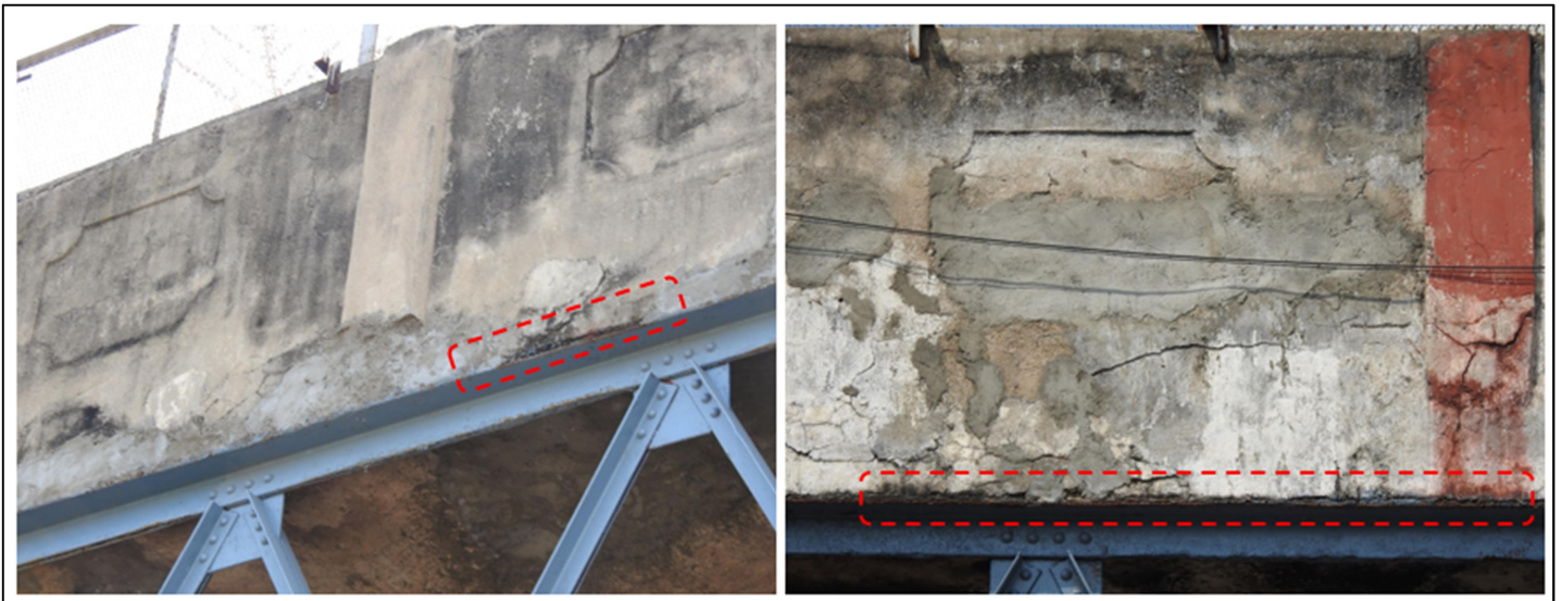
Fig: 11 Corrosion at the steel concrete joints of Exterior Support Truss.
