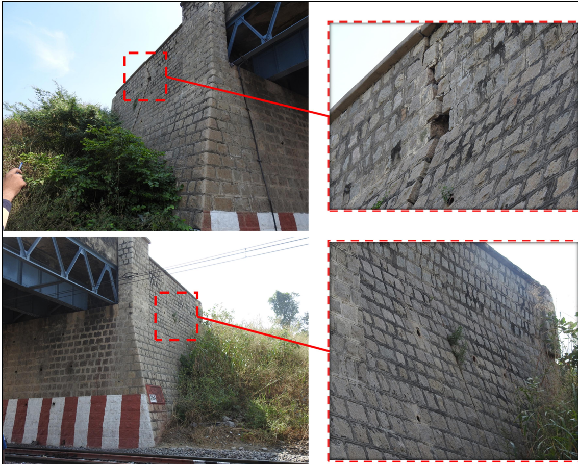
Fig: 10 pointing and vegetation on Abutments on both sides
