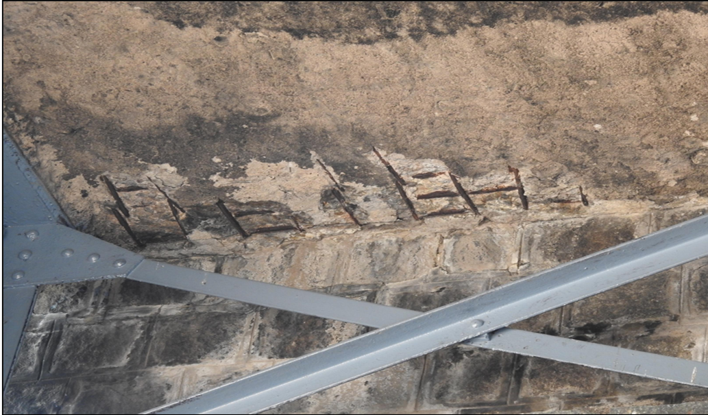
Fig: 8 Leaching and exposed reinforcement in slab
