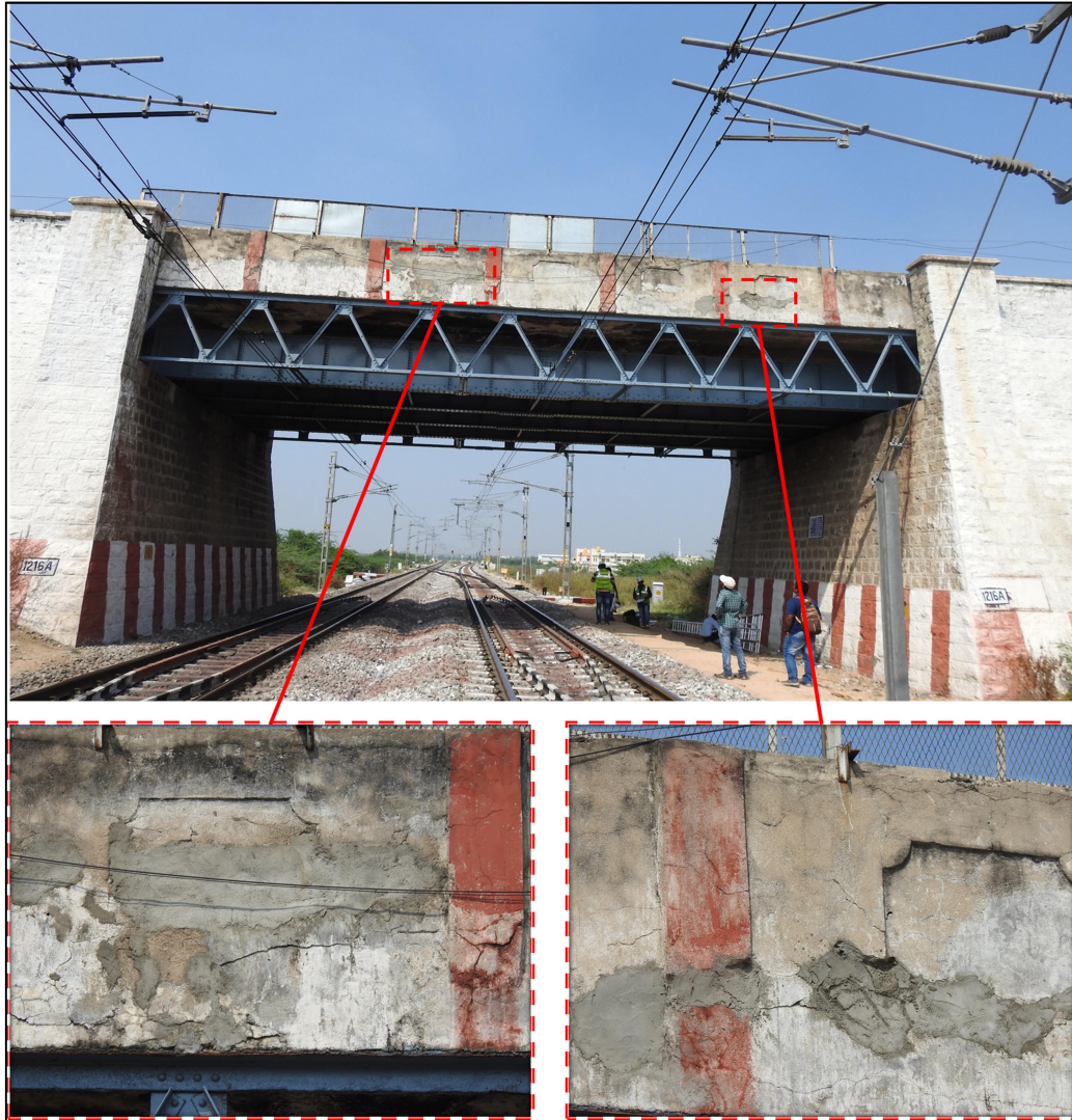
Fig: 7 Patch work observed in Parapet wall
