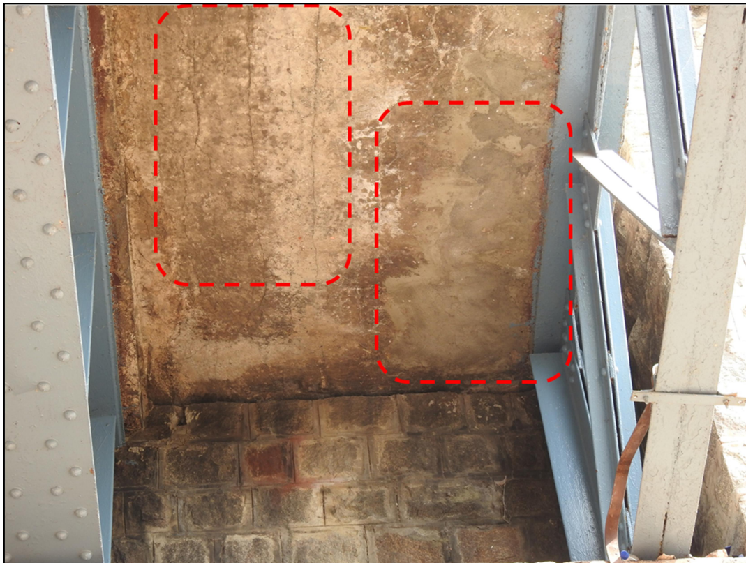
Fig: 9 Cracks and patch work observed in slab.
