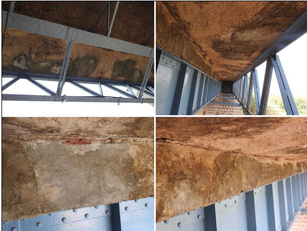
Fig: 6 Patch work observed in Slab
