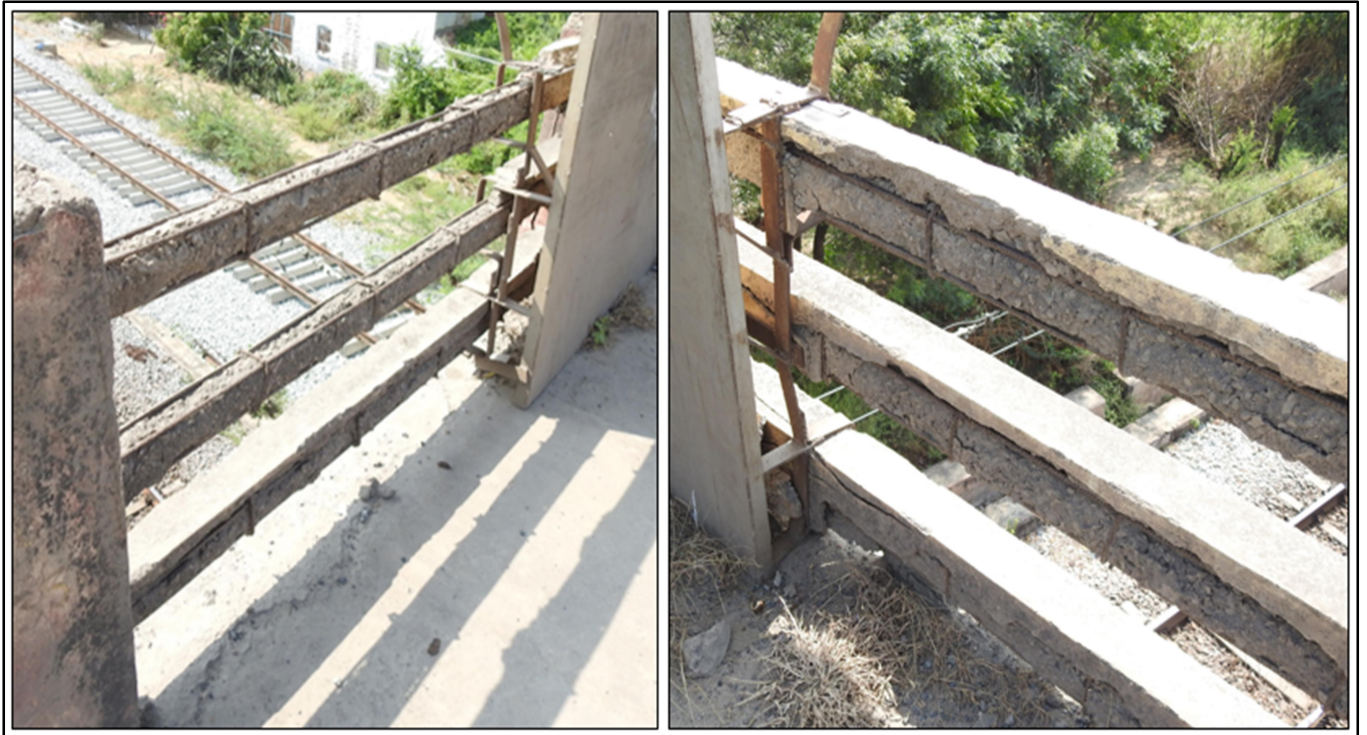
Fig.10: Spalling & Reinforcement exposed on Railings.
