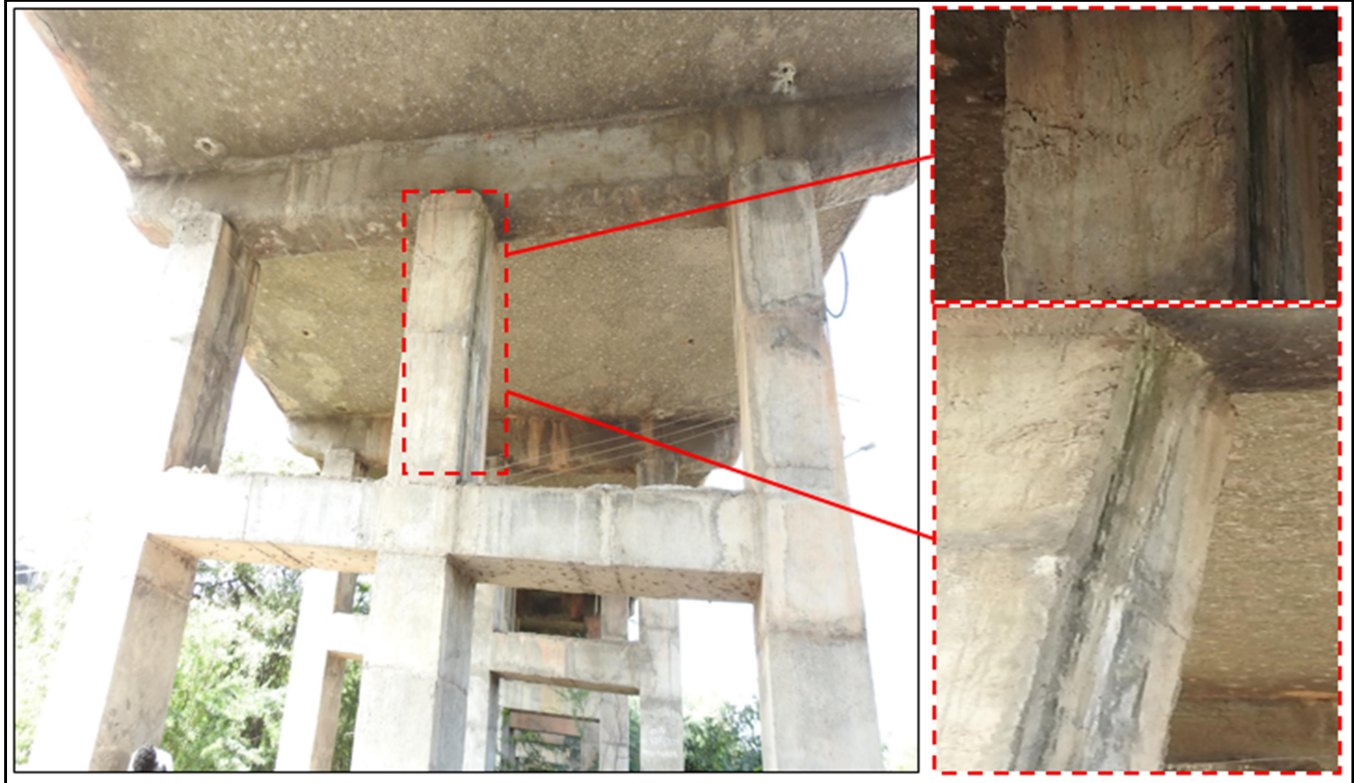
Fig.7: Cracks and leaching is observed at pier-3.
