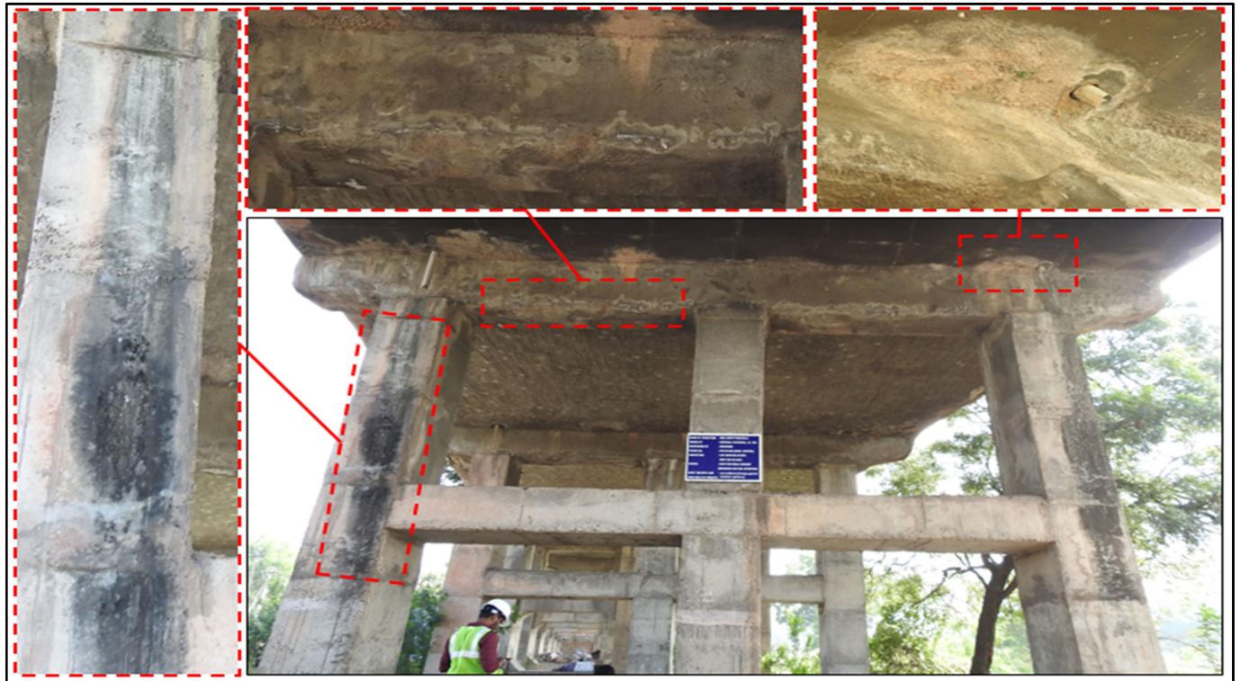
Fig.5: Spalling and leaching observed at columns and cap of pier-1.
