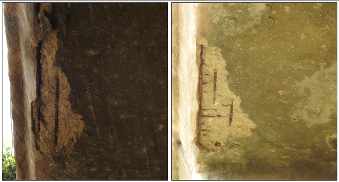
Fig.8: Reinforcement exposed and distresses at other spans of ROB.
