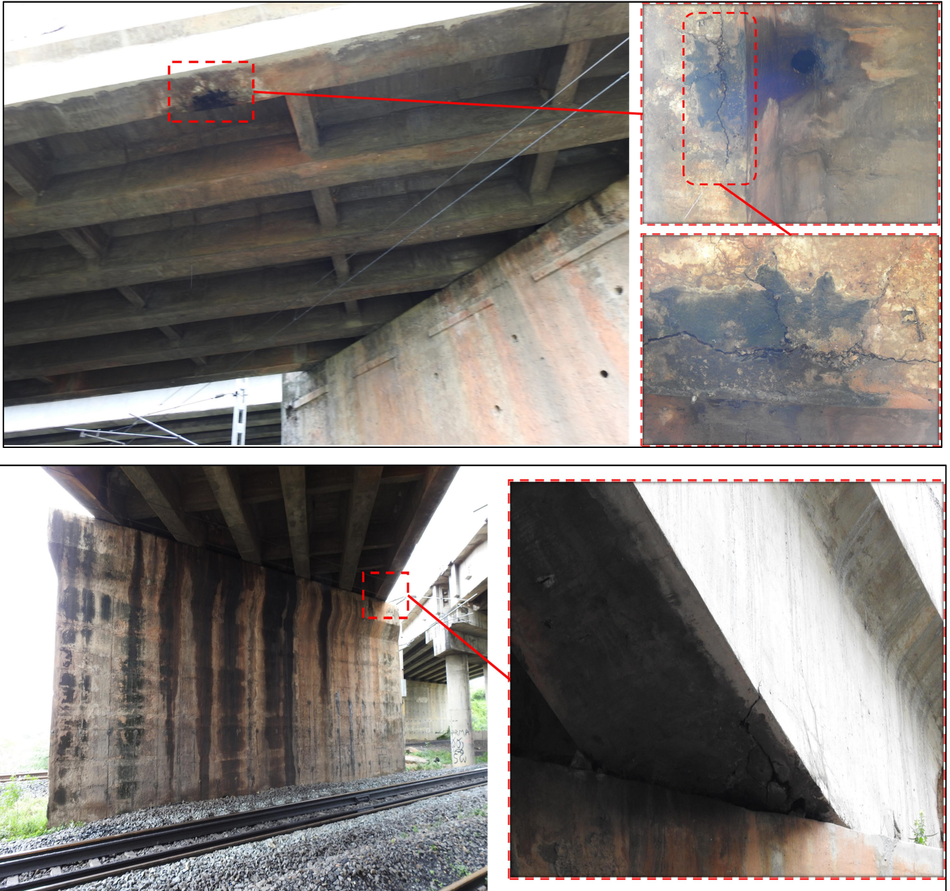
Fig 4: Cracks observed in Exterior girder
