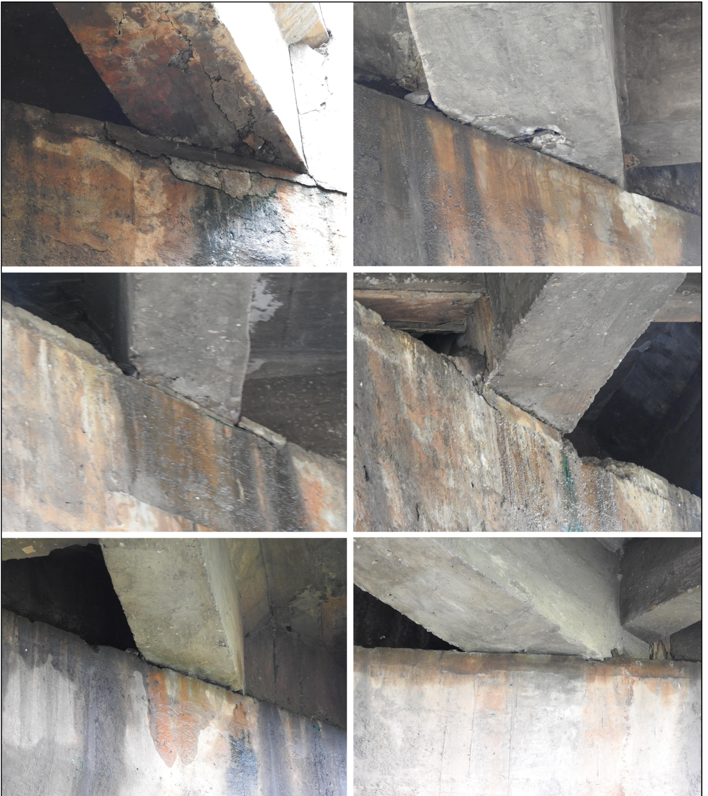
Fig 6: Distresses observed at Bearings
