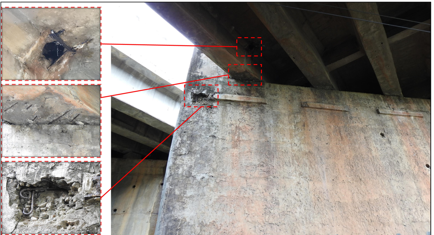
Fig 5(b): Reinforcement exposed in exterior girder, pier and slab at drainage spout
