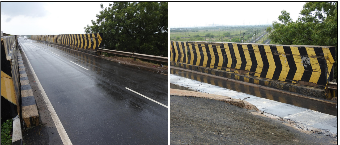
Fig 9: Wearing Coat condition & Accident hitting marks on Crash Barrier.
