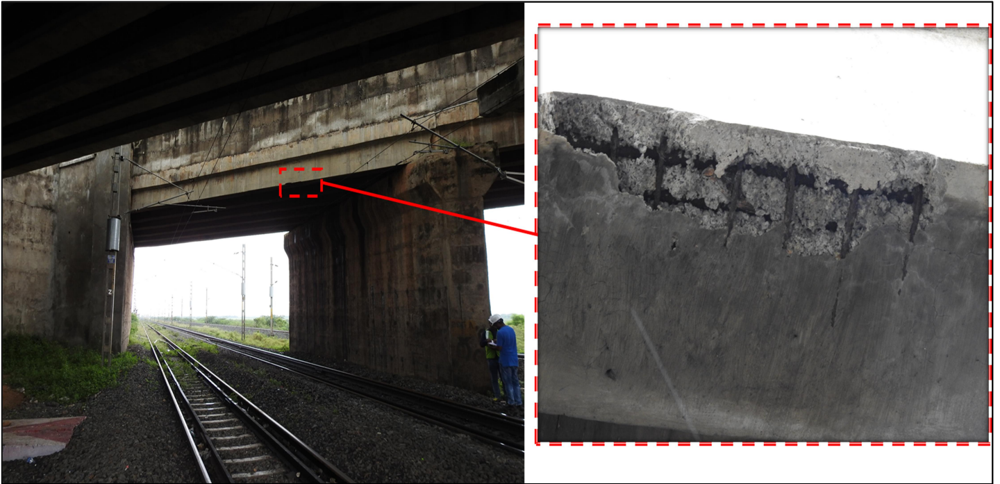
Fig 5(a): Reinforcement exposed in exterior girder
