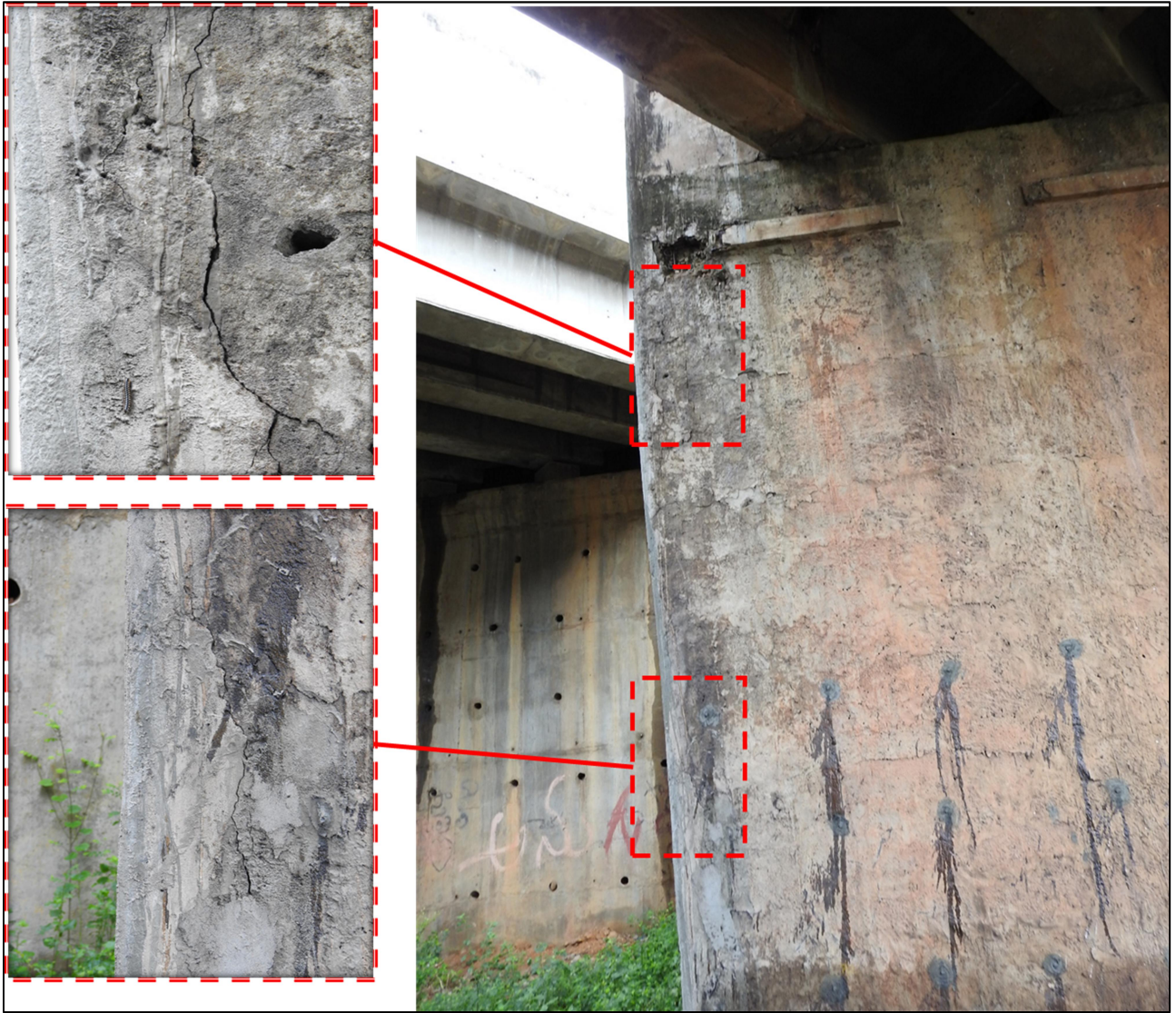
Fig 7: Cracks observed on pier
