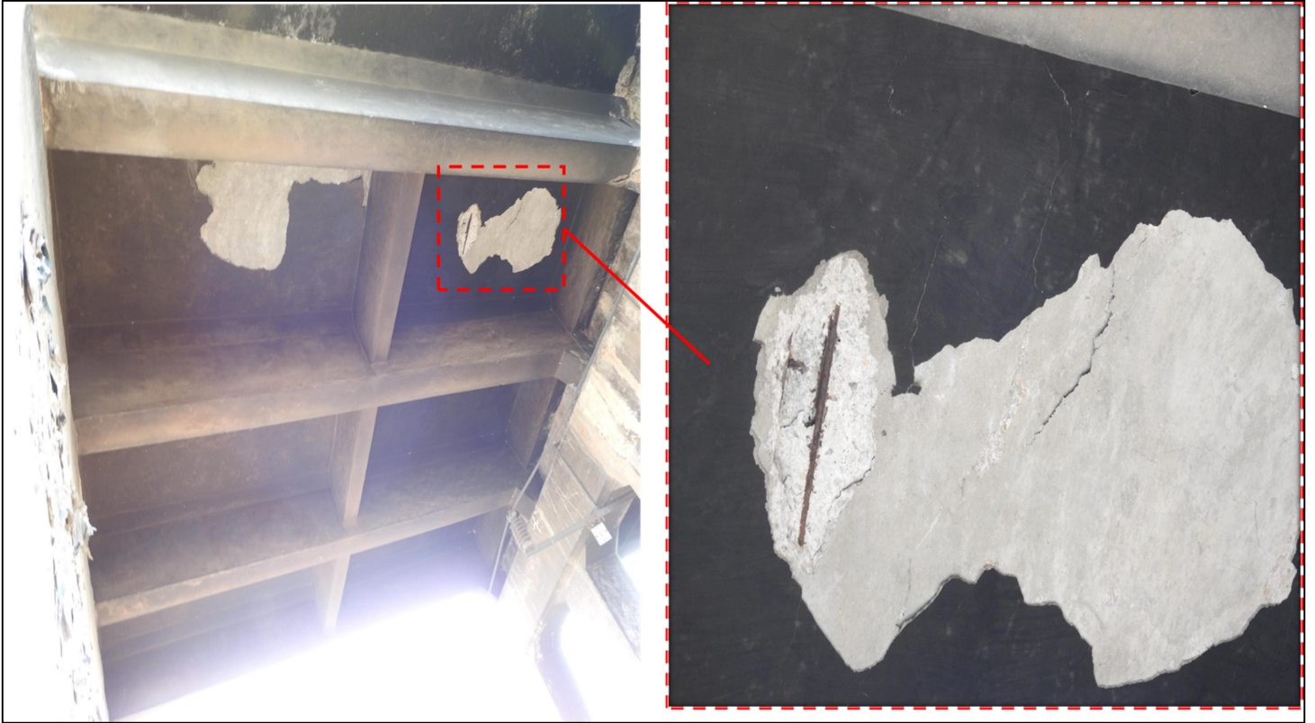
Fig 9: Spalling & Reinforcement exposure at Slab of span-3.
