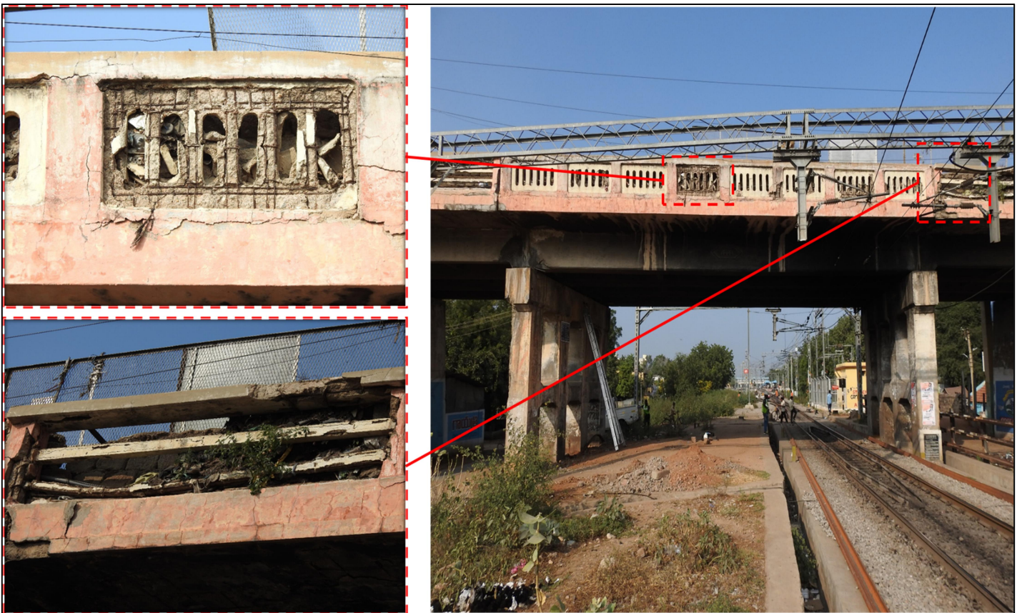
Fig 6: Distressed / Poor condition of Railing
