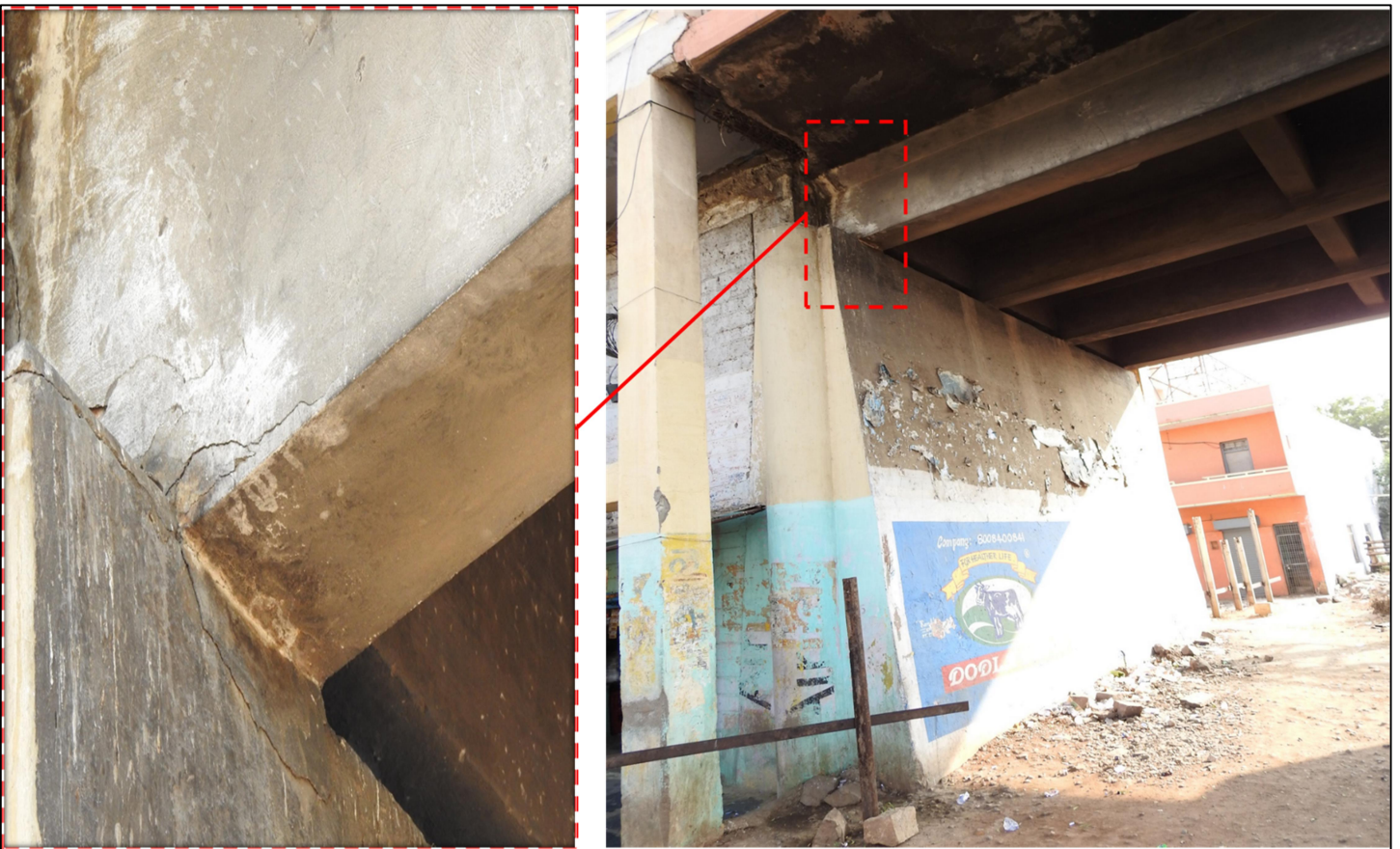
Fig 9: Cracks observed at girder seating location of Span-3.
