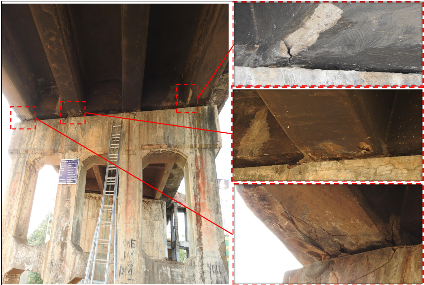
Fig 3: Cracks & Spalling observed in girders
