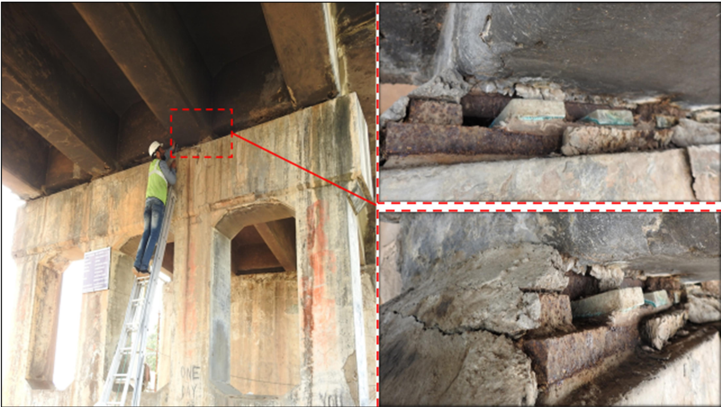
Fig 4: Mortar Patching & Distresses observed at Bearings
