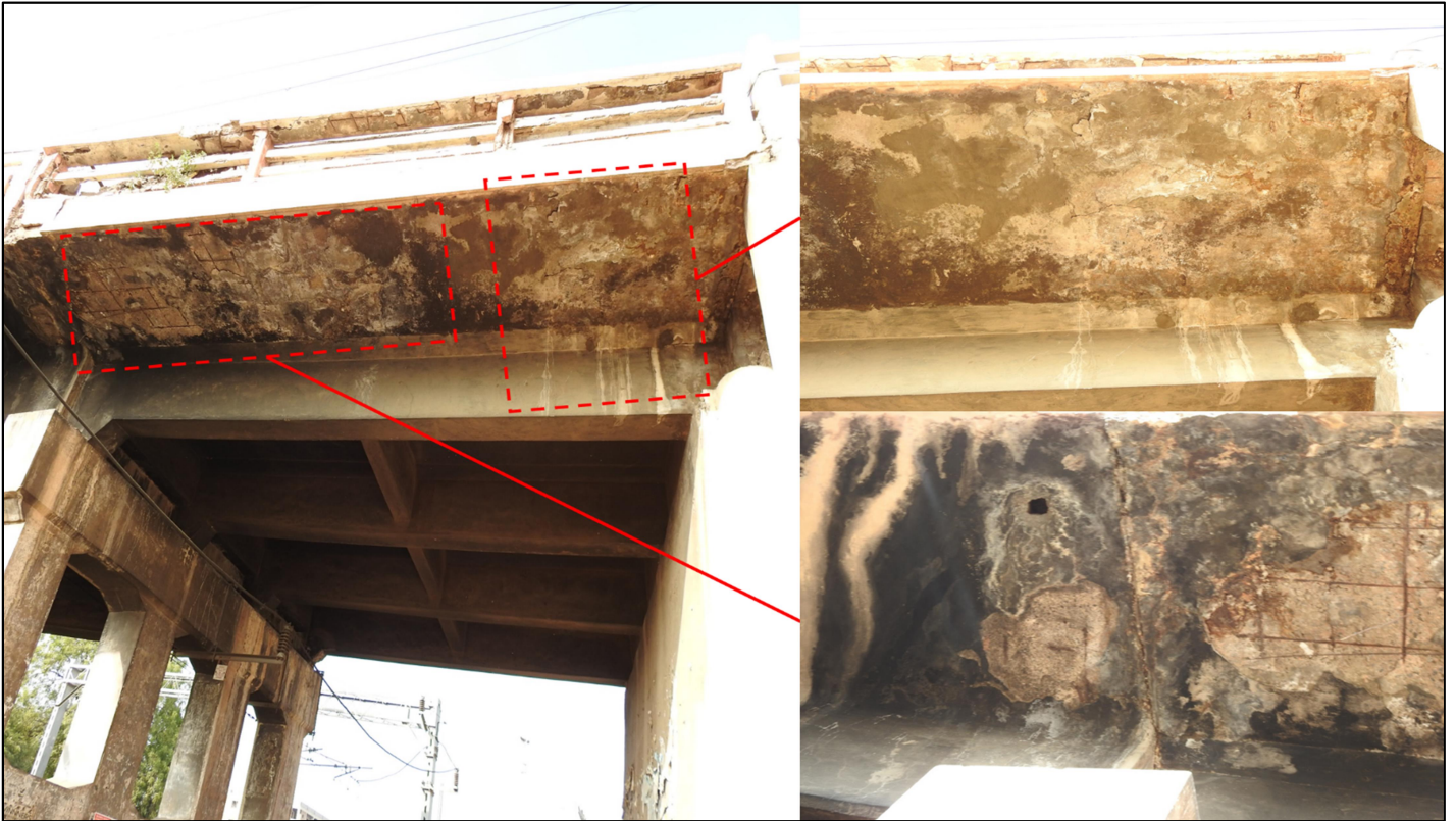
Fig 8: Spalling, Leaching & Reinforcement exposure on slab of Span-1
