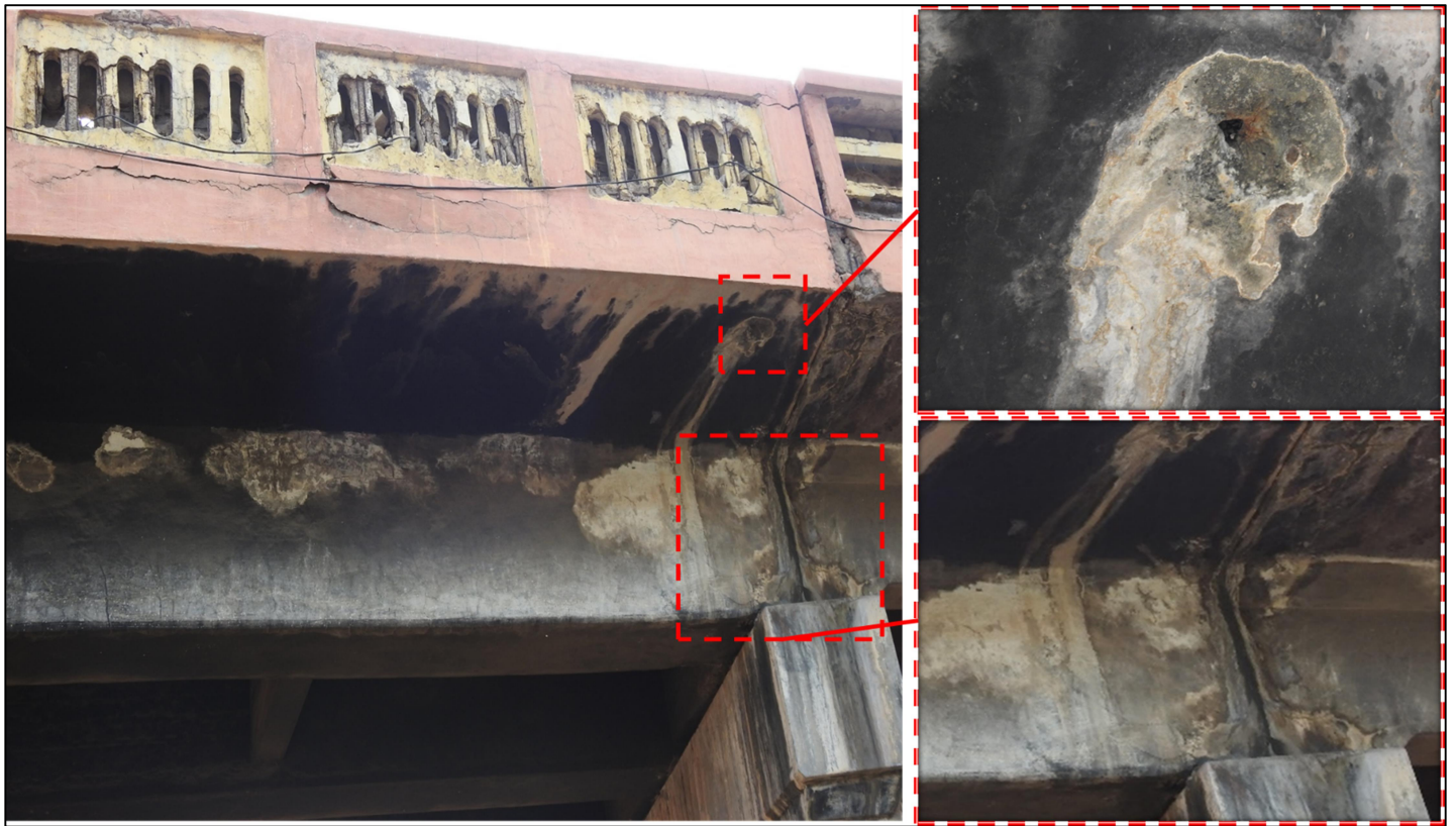
Fig 5(d): Leaching at girder and Slab at drainage spout location
