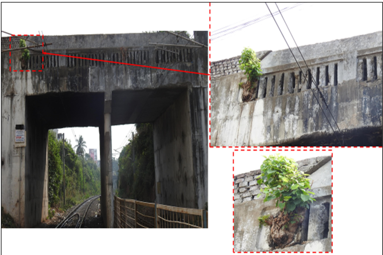
Fig: 8 Vegetation growth observed at Railing of ROB
