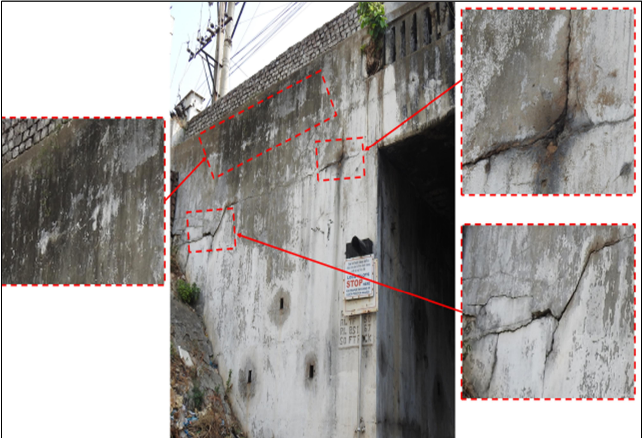
Fig: 7 Spalling, Cracks & Leaching observed at Abutment-1
