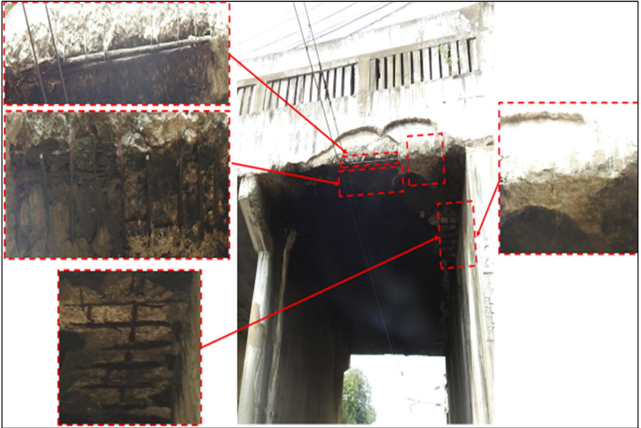
Fig: 4 Reinforcement exposure and Spalling observed at Span-1
