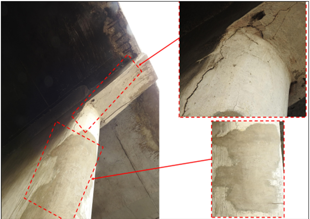
Fig: 5 Cracks & Patch repair work observed at Pier
