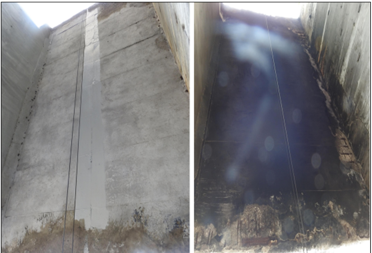
Fig: 3 Bottom view of Slab
