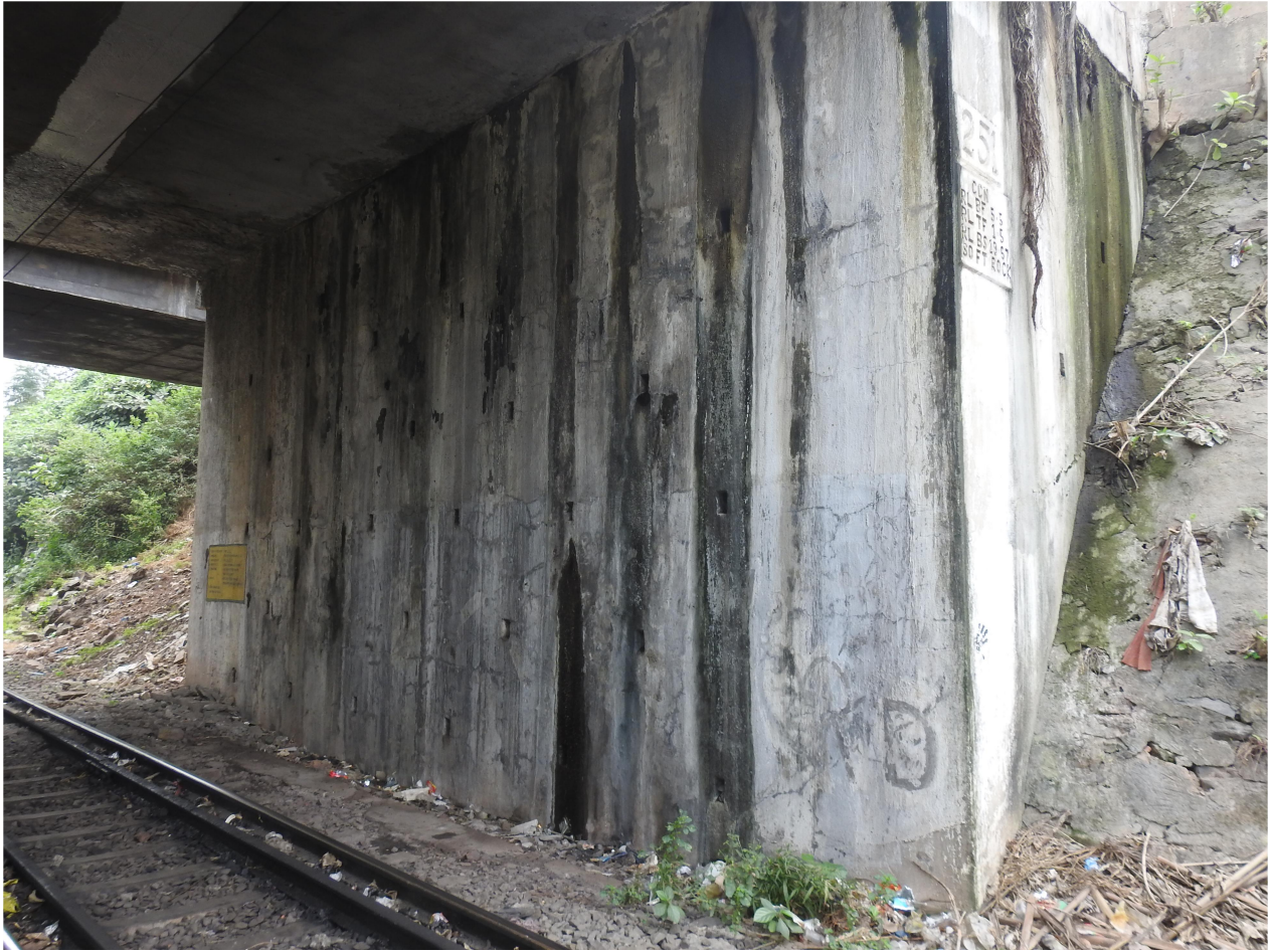
Fig: 4 Water seepage at abutment
