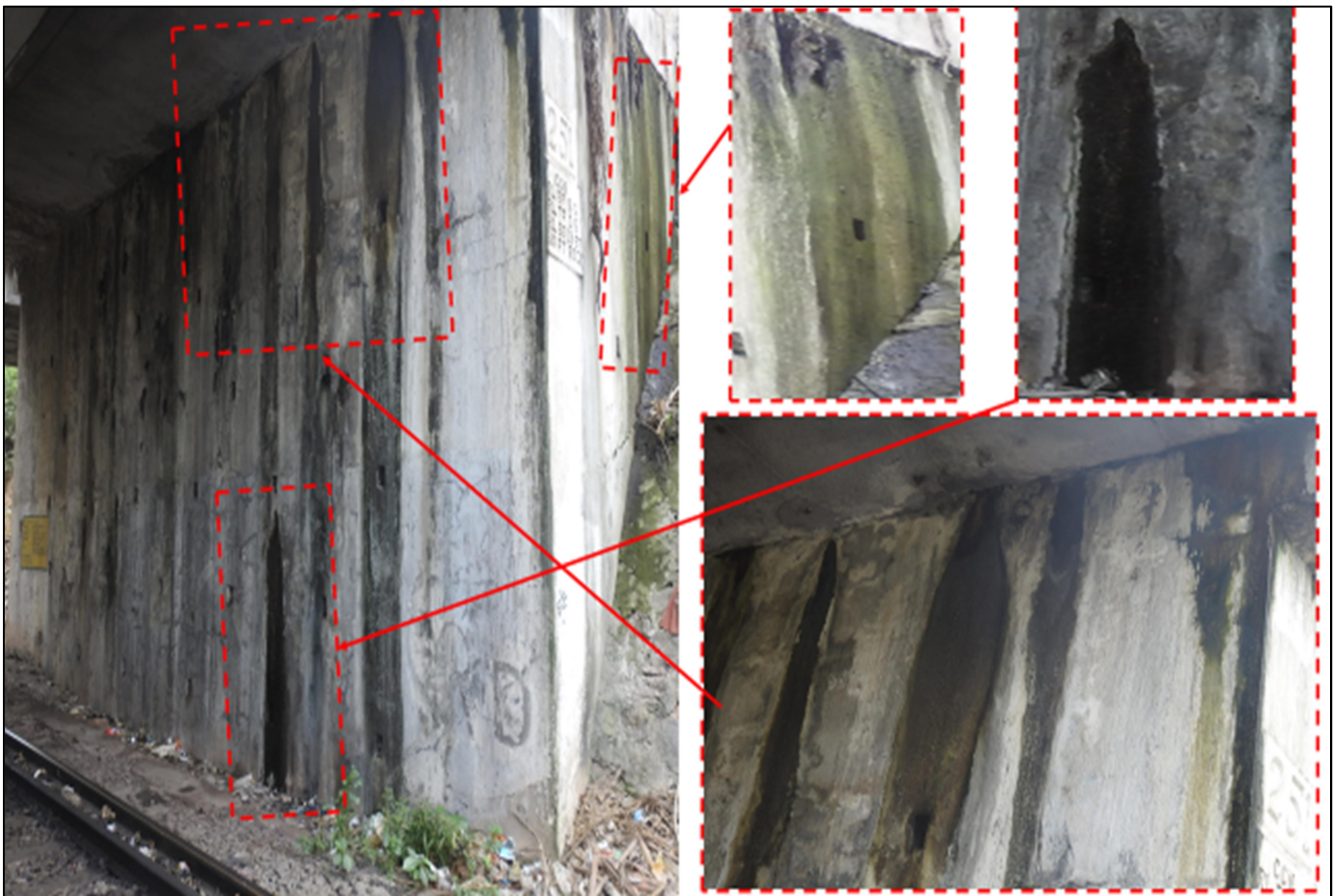
Fig 14: Algae observed on Abutment-2
