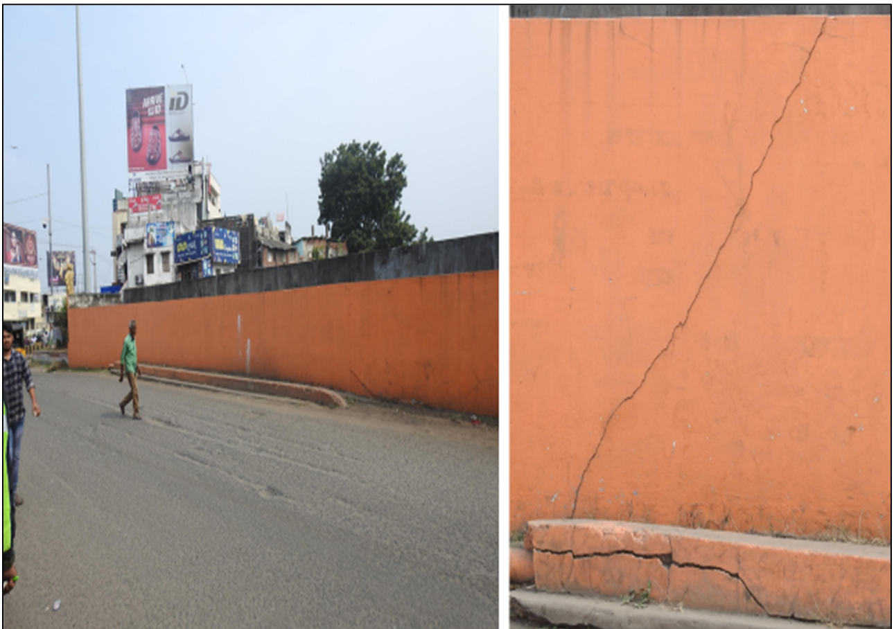
Fig: 3 Cracks observed on parapet wall
