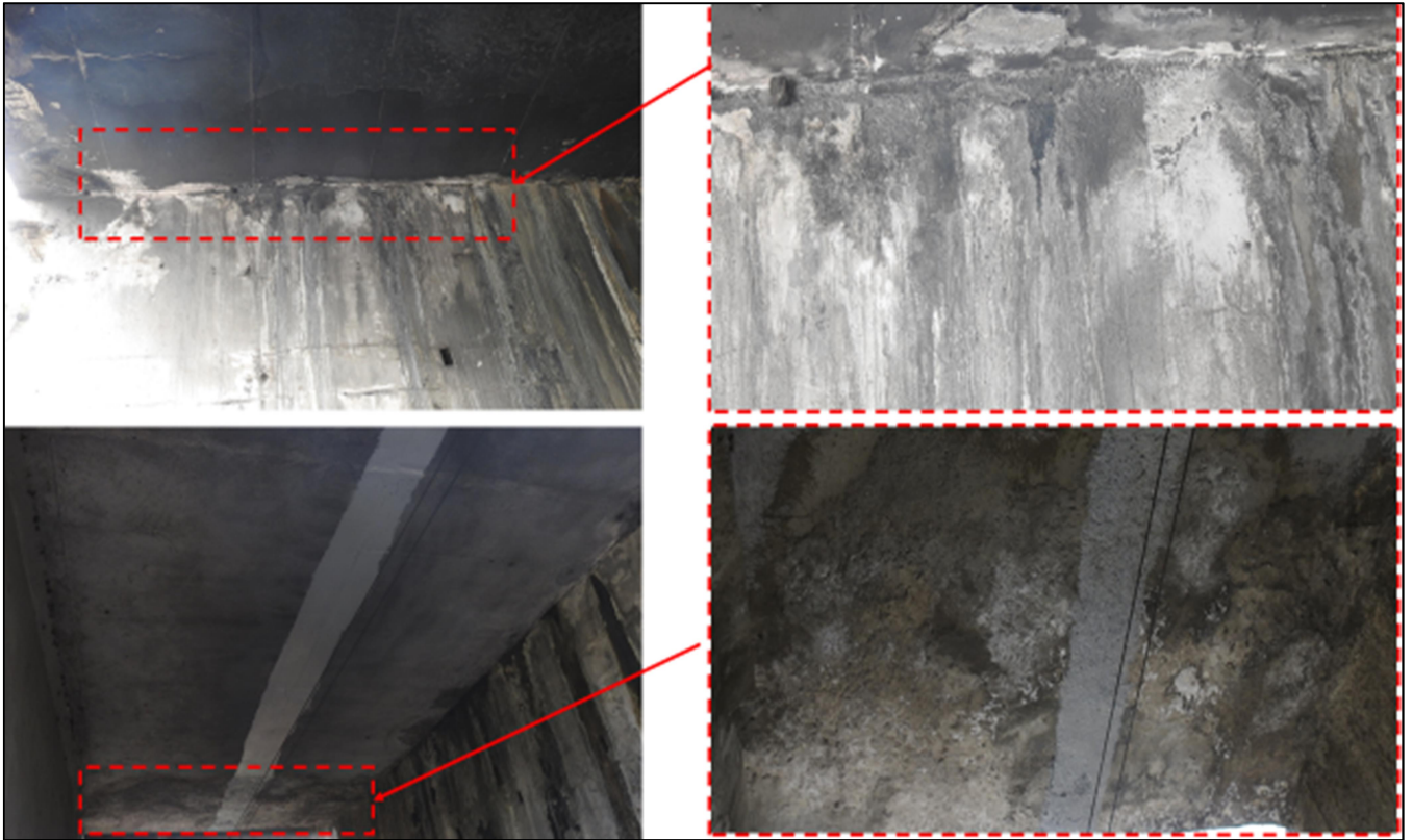
Fig 9: Leaching observed on Slab – 1 & Slab-2
