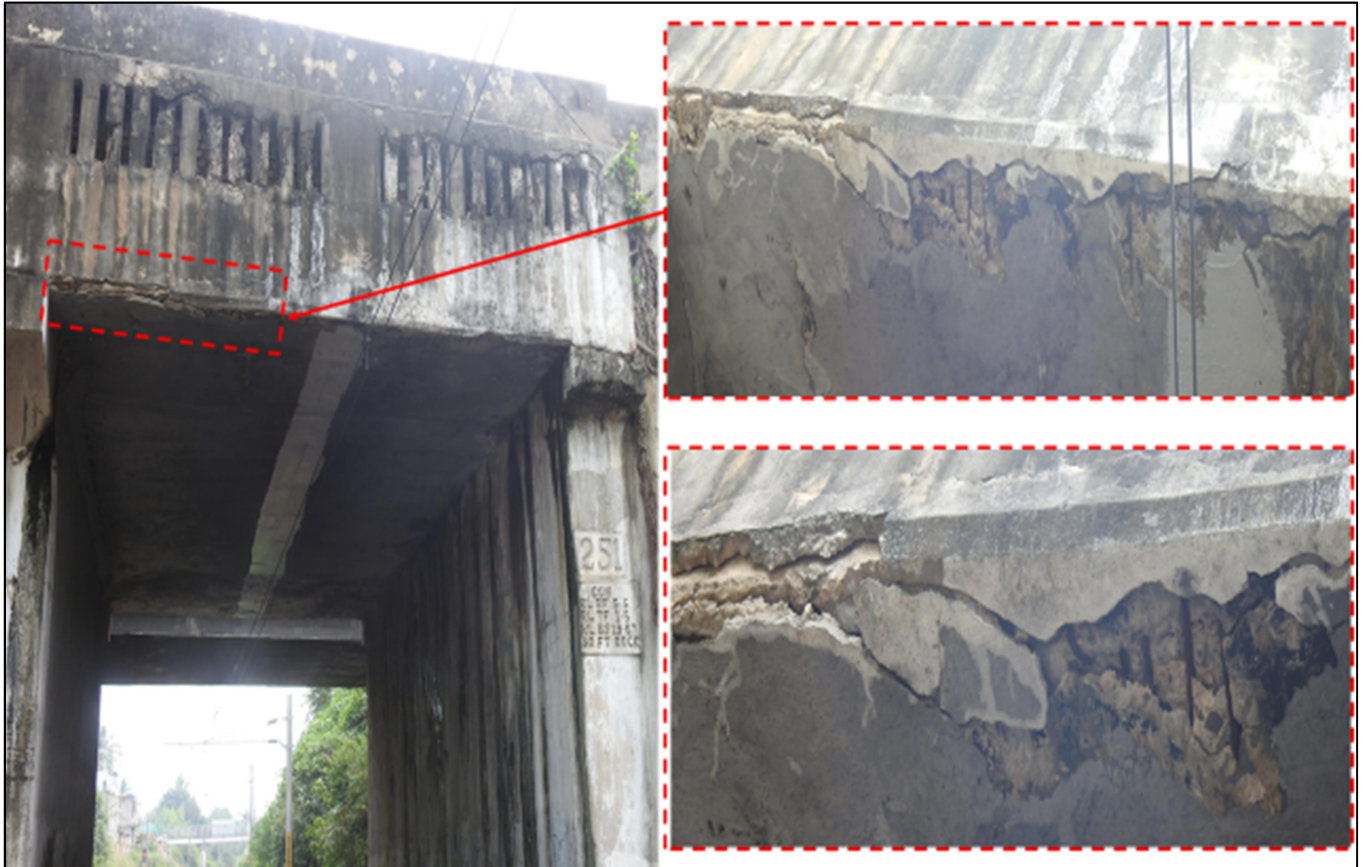
Fig 11: Reinforcement exposure observed at Span-2
