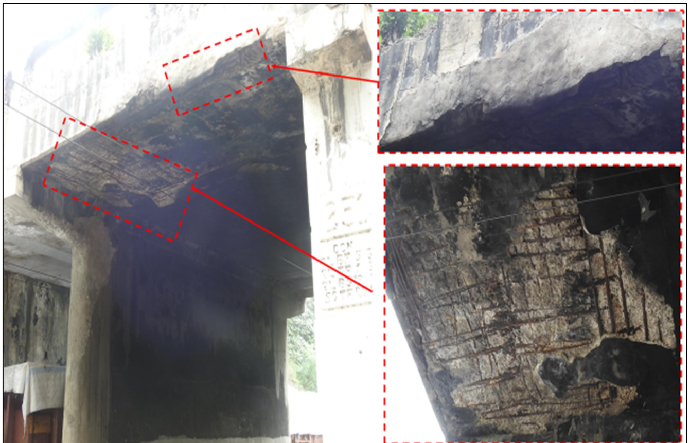
Fig 8: Reinforcement exposure & Spalling observed at Span-1
