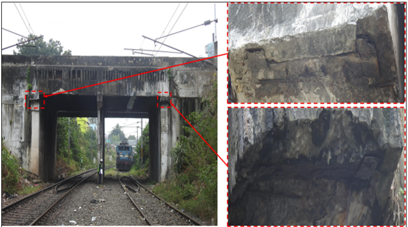
Fig 12: Spalling observed at both Abutment Pier caps
