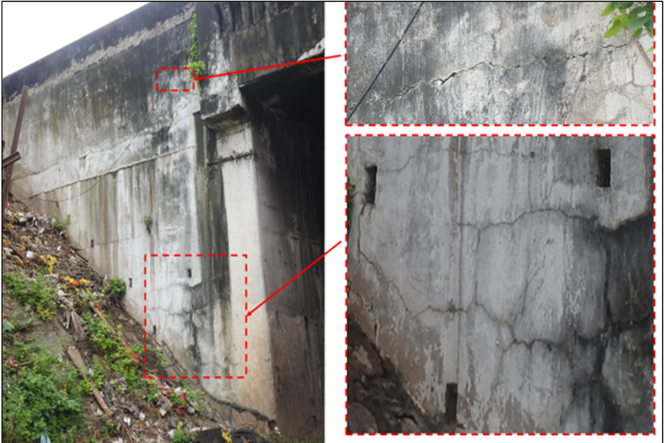
Fig: 5 Cracks observed at Abutment 1
