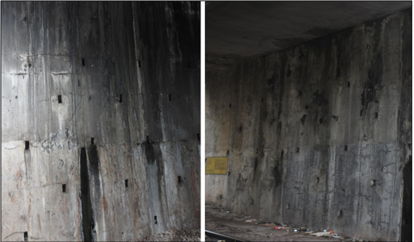
Fig 13: Shrinkage cracks observed on A1 & A2 Abutments
