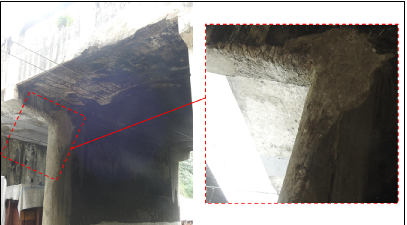
Fig 10: Cracks & Spalling observed at Pier
