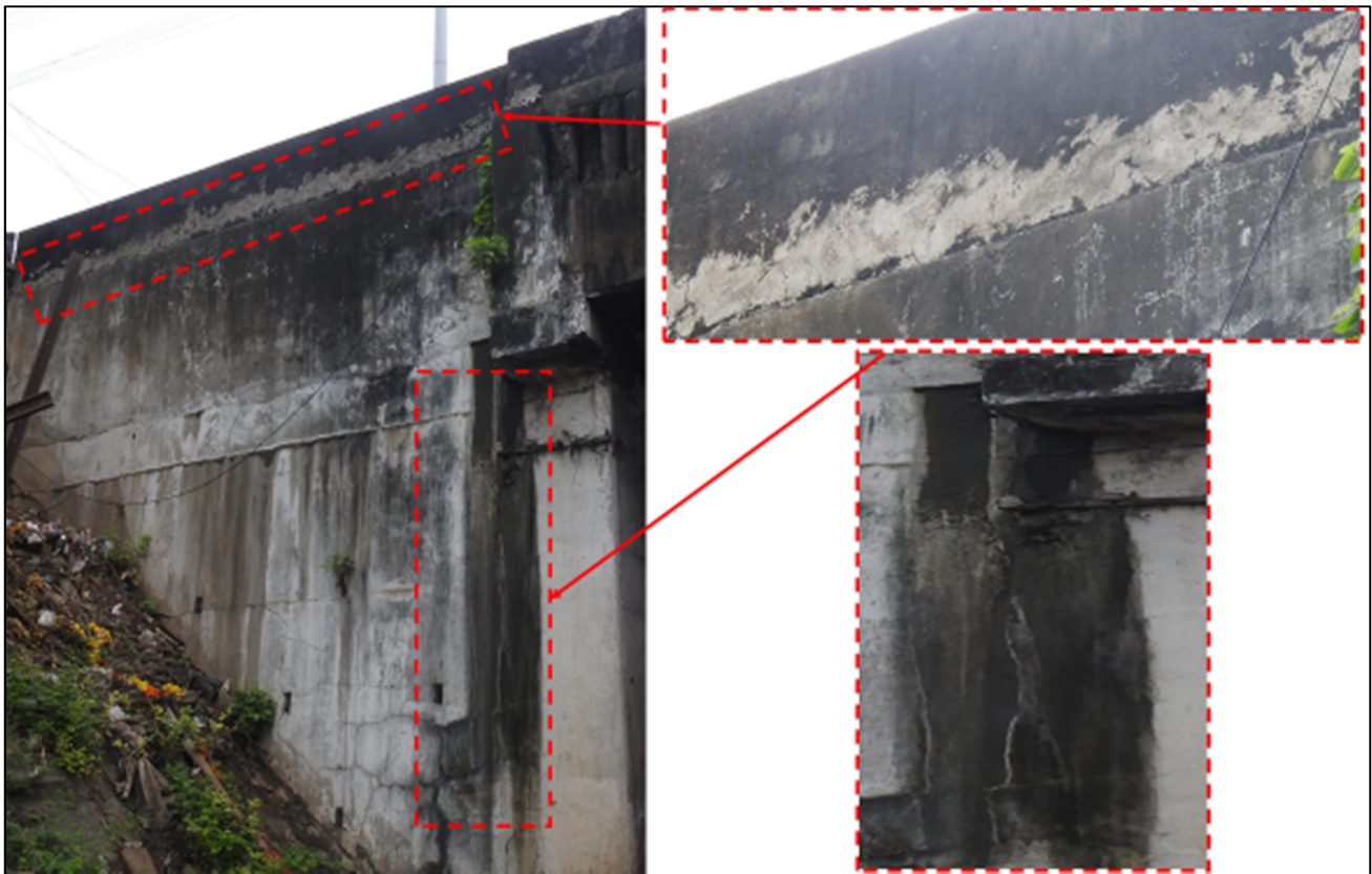
Fig:6 Patch work & Leaching observed at Abutment-1
