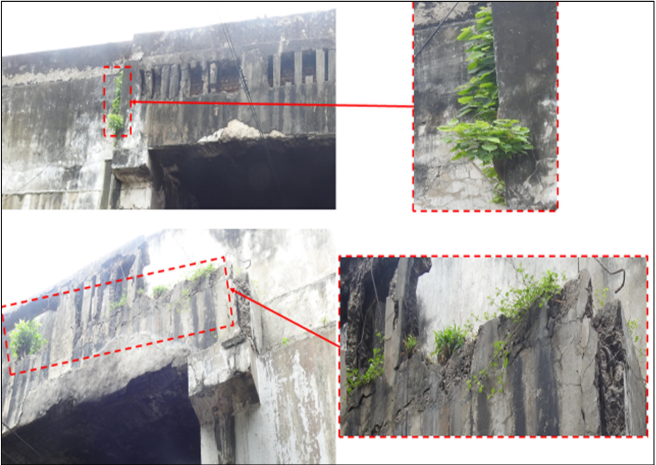
Fig 7: Vegetation growth observed at Abutment-1
