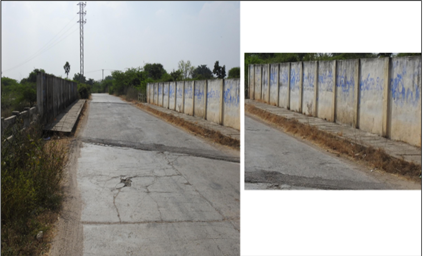
Fig 9: Condition of Road surface & Parapet wall
