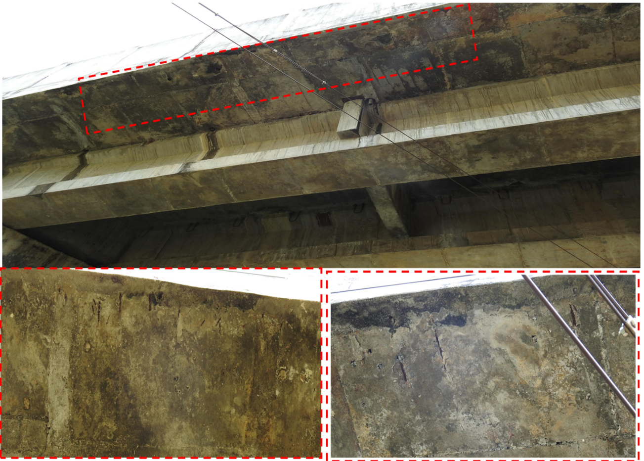
Fig 4: Spalling at overhang portion of slab
