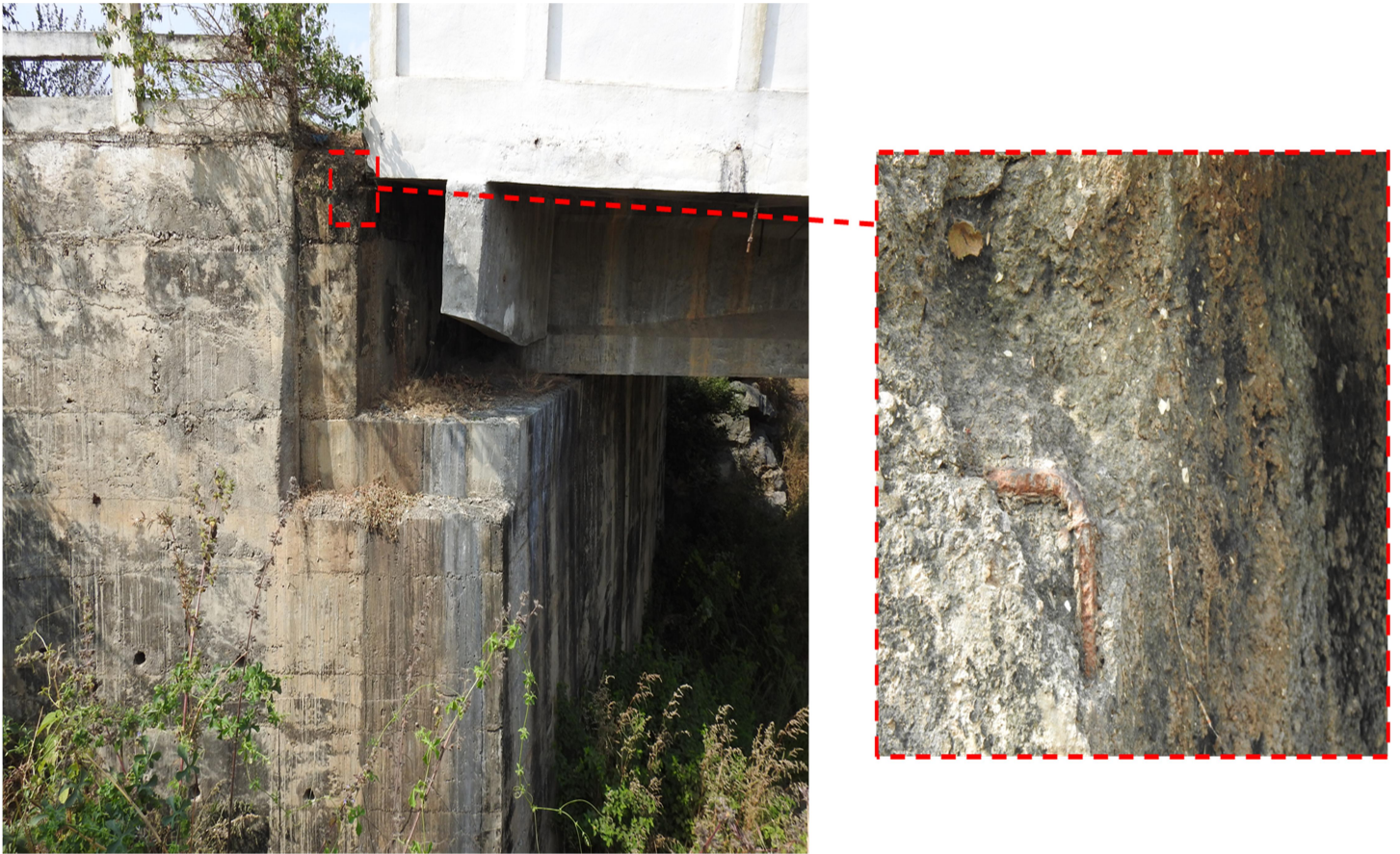
Fig 7: Spalling observed at dirt wall
