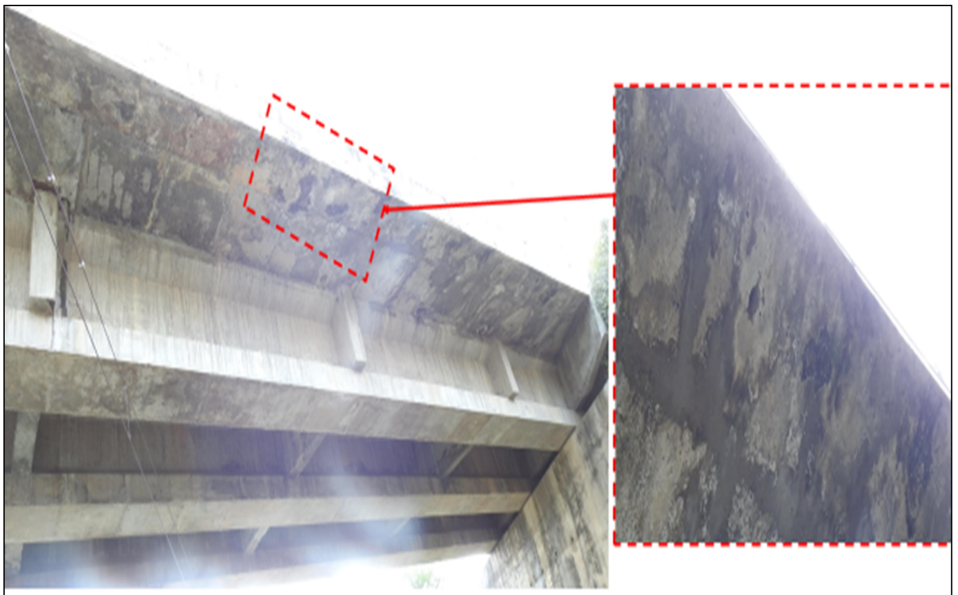
Fig 6: Leaching observed at Slab
