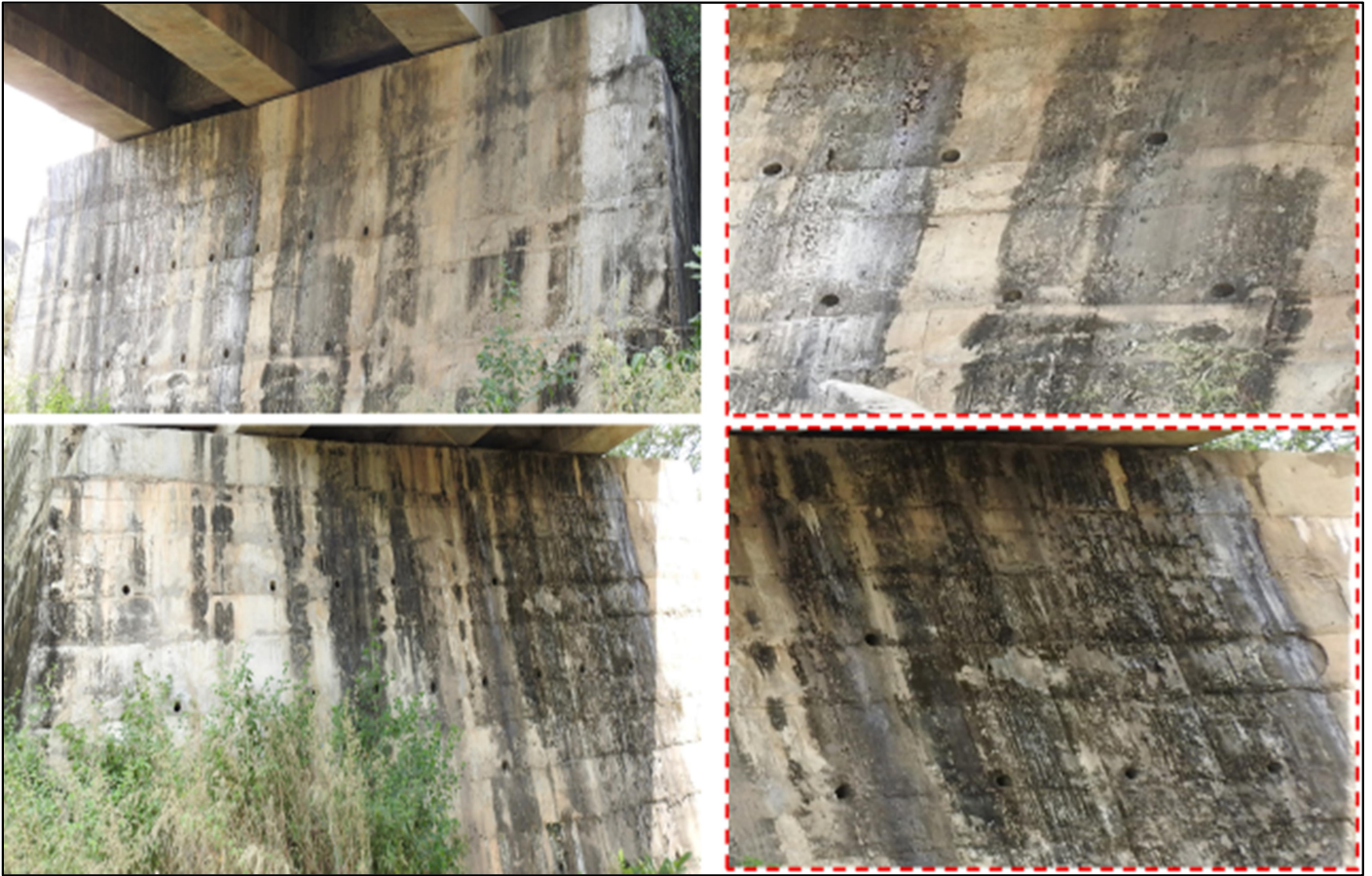
Fig 5: Leaching observed at Abutment -1 & 2
