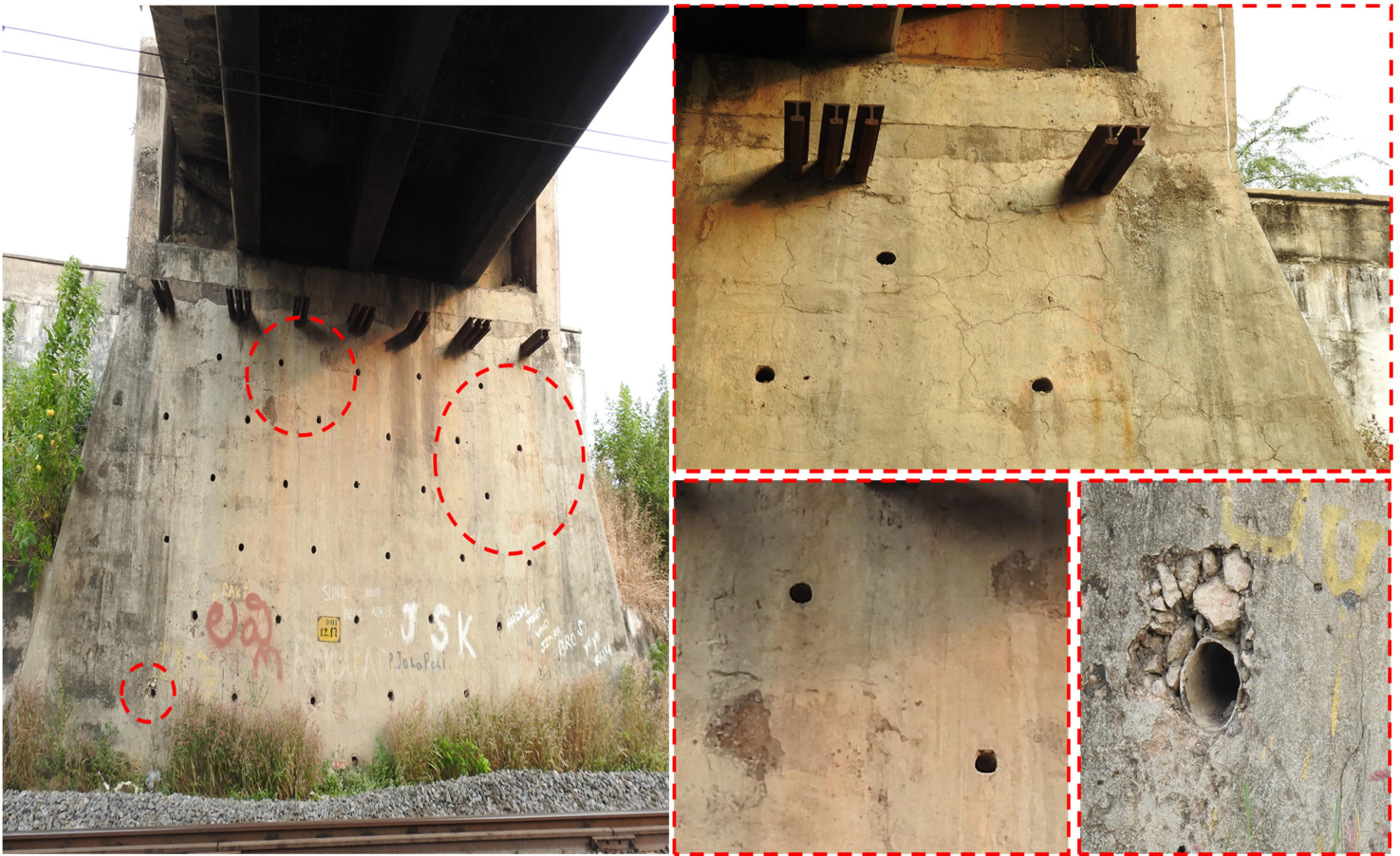
Fig 11: Shrinkage cracks and minor spalling at Abutment 1
