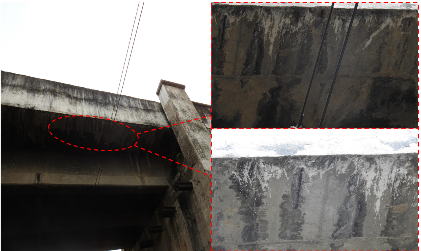
Fig 10: Spalling at Overhang Slab portion
