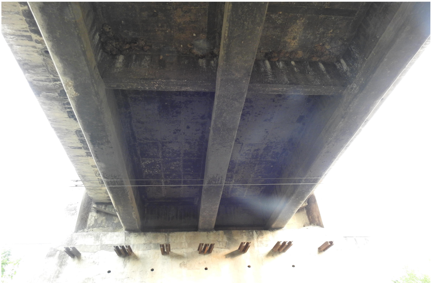
Fig: 3 Bottom view, Leaching observed
