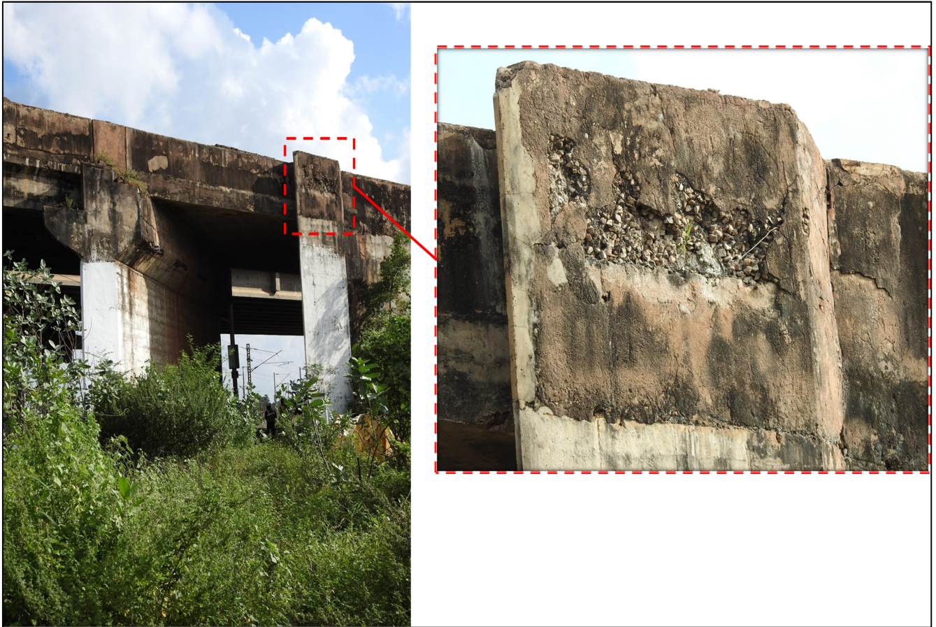
Fig 4: Spalling and reinforcement exposed in abutment
