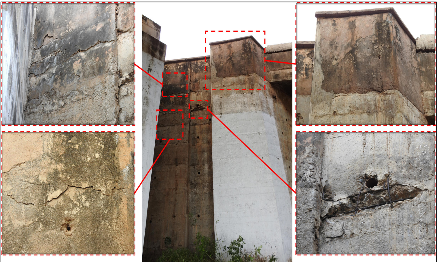
Fig 7: Distresses observed at Retaining Walls & Abutment
