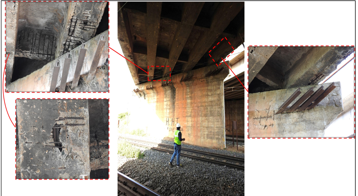
Fig 12: Severe Spalling & Reinforcement exposure at girder ends
