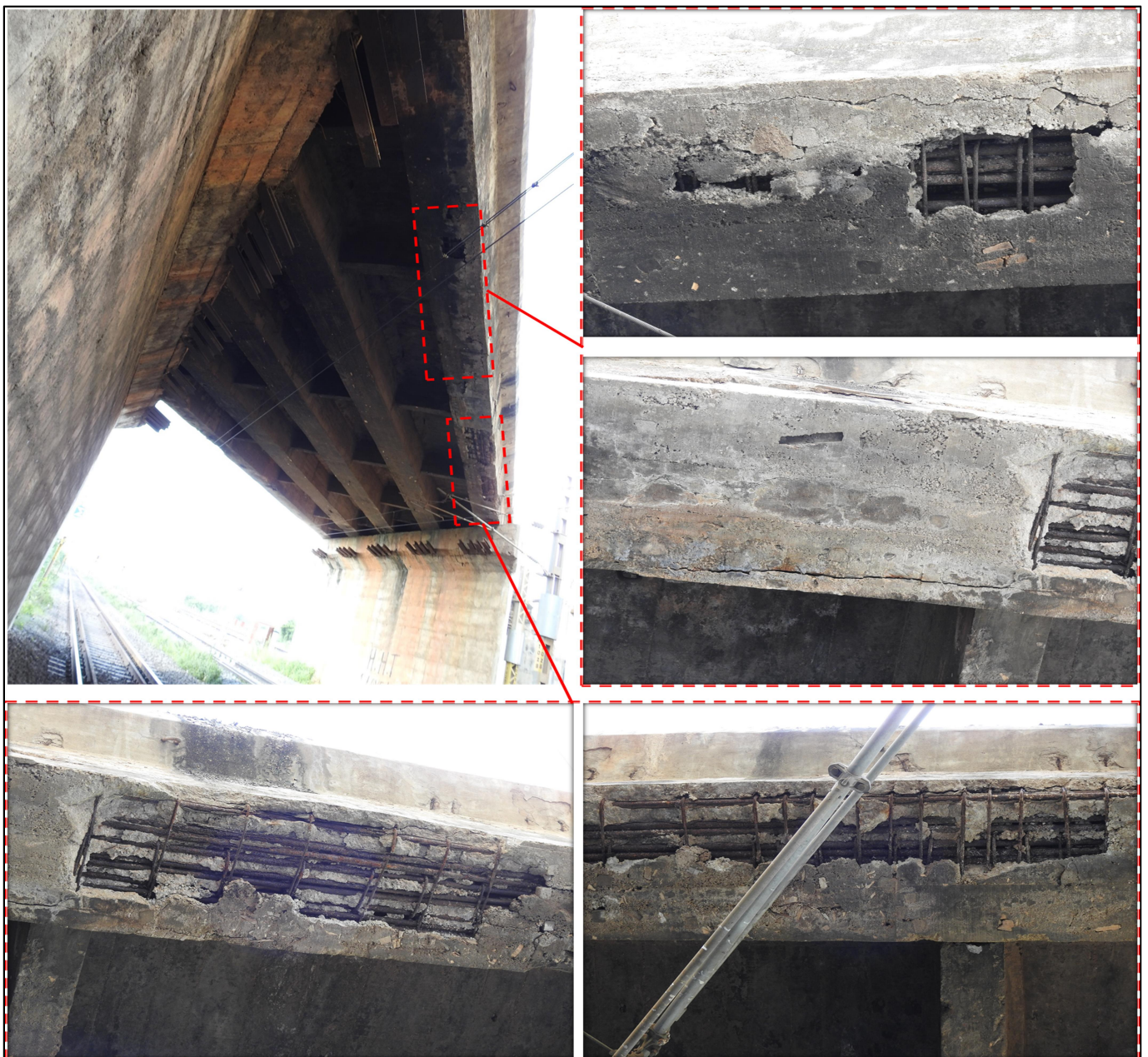
Fig 11: Severe Spalling & Reinforcement exposure at exterior girder of Span-3
