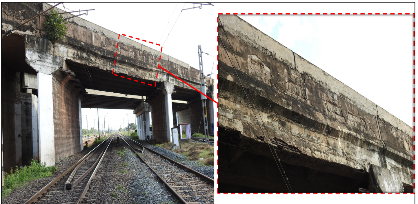
Fig 13: Spalling & Reinforcement exposure at exterior girder & parapet
