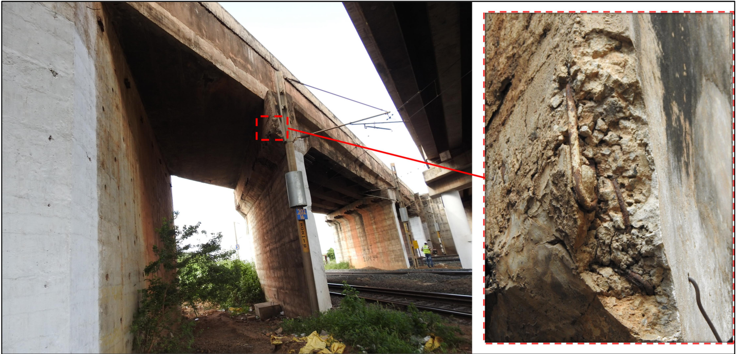
Fig 8: Spalling & Reinforcement exposed at Pier
