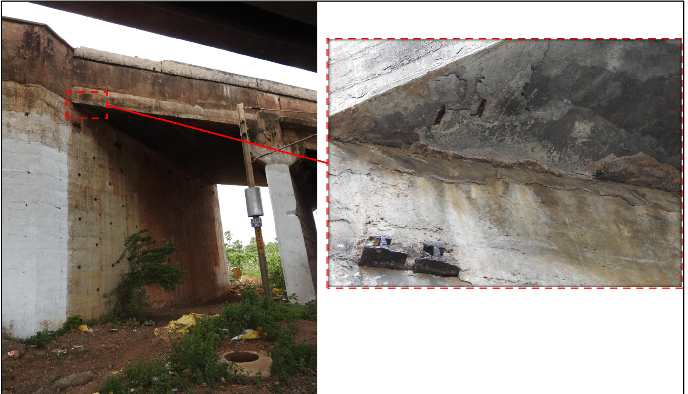
Fig 6: Reinforcement exposure at slab and Corroded Rail sections (Shuttering Support) at Abutment
