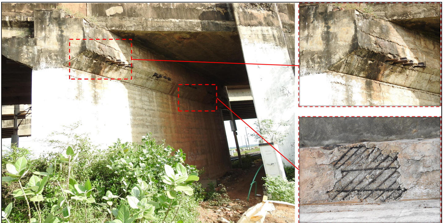
Fig 5 Spalling & Reinforcement exposed at Pier-1
