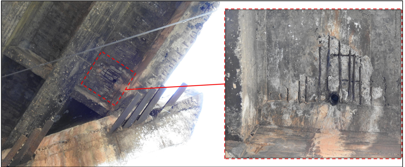
Fig 10: Spalling & Reinforcement exposure in slab at drainage spout location
