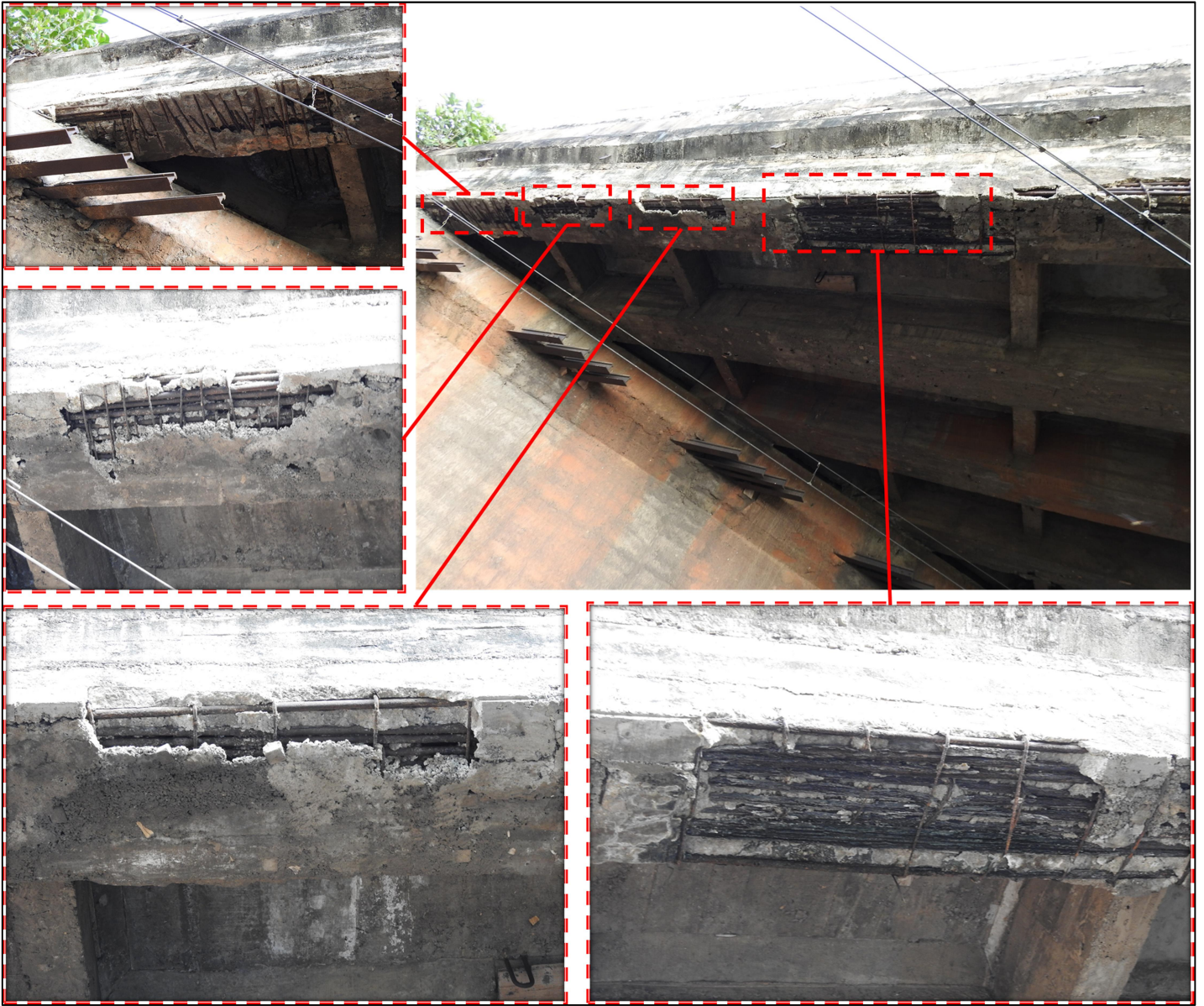
Fig 16: Severe Spalling & Reinforcement exposure at exterior girders
