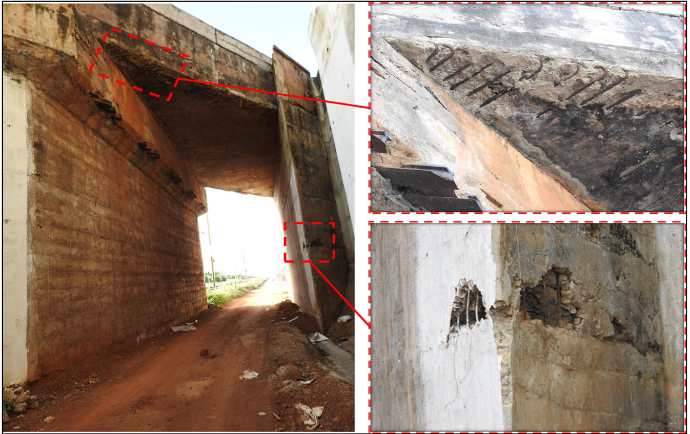
Fig 15: Spalling & Reinforcement exposure at Slab of Span-4 & Abutment
