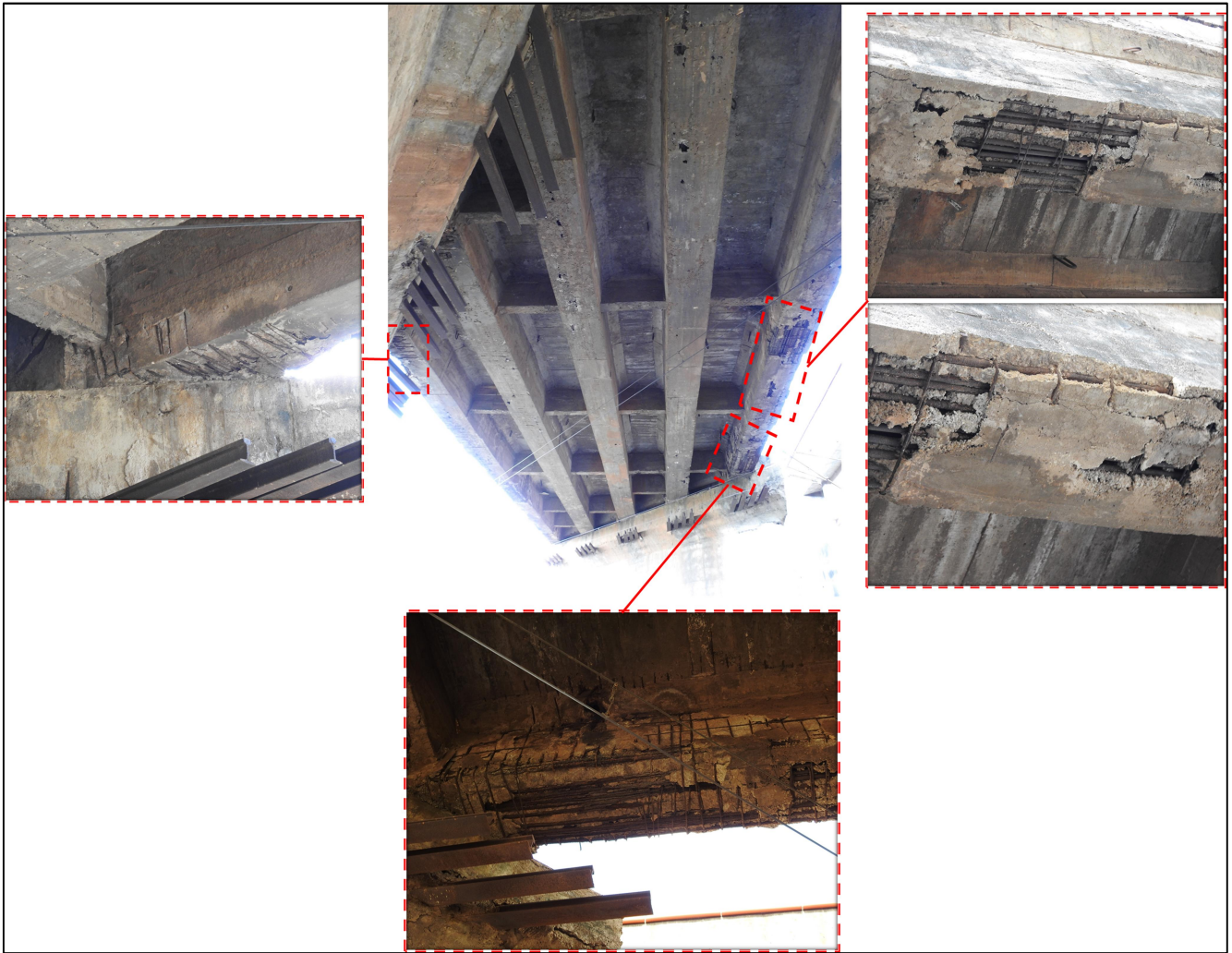
Fig 14: Severe Spalling & Reinforcement exposure at girders
