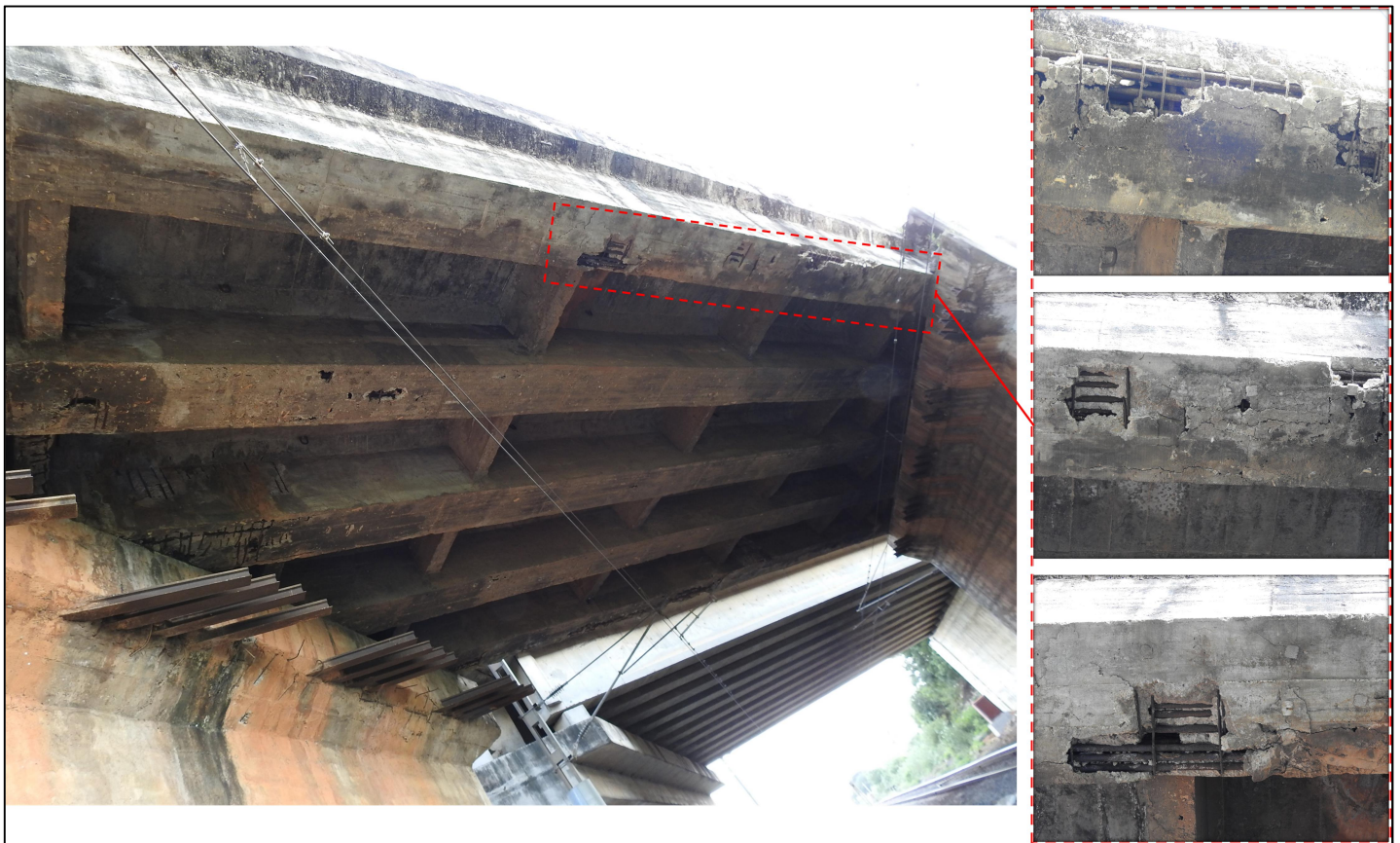
Fig 9: Severe Spalling & Reinforcement exposure at exterior girder of Span-2
