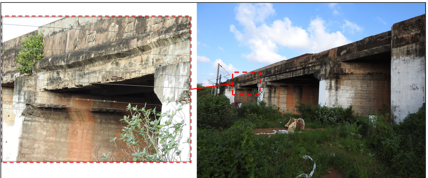
Fig 17: Deflection Observed at Exterior Girder of Span-3
