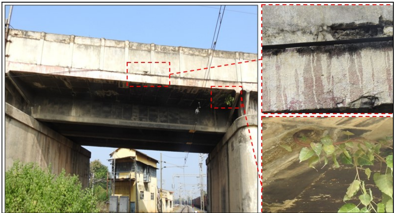
Fig.10 : Spalling and vegetation observed in span 3 .
