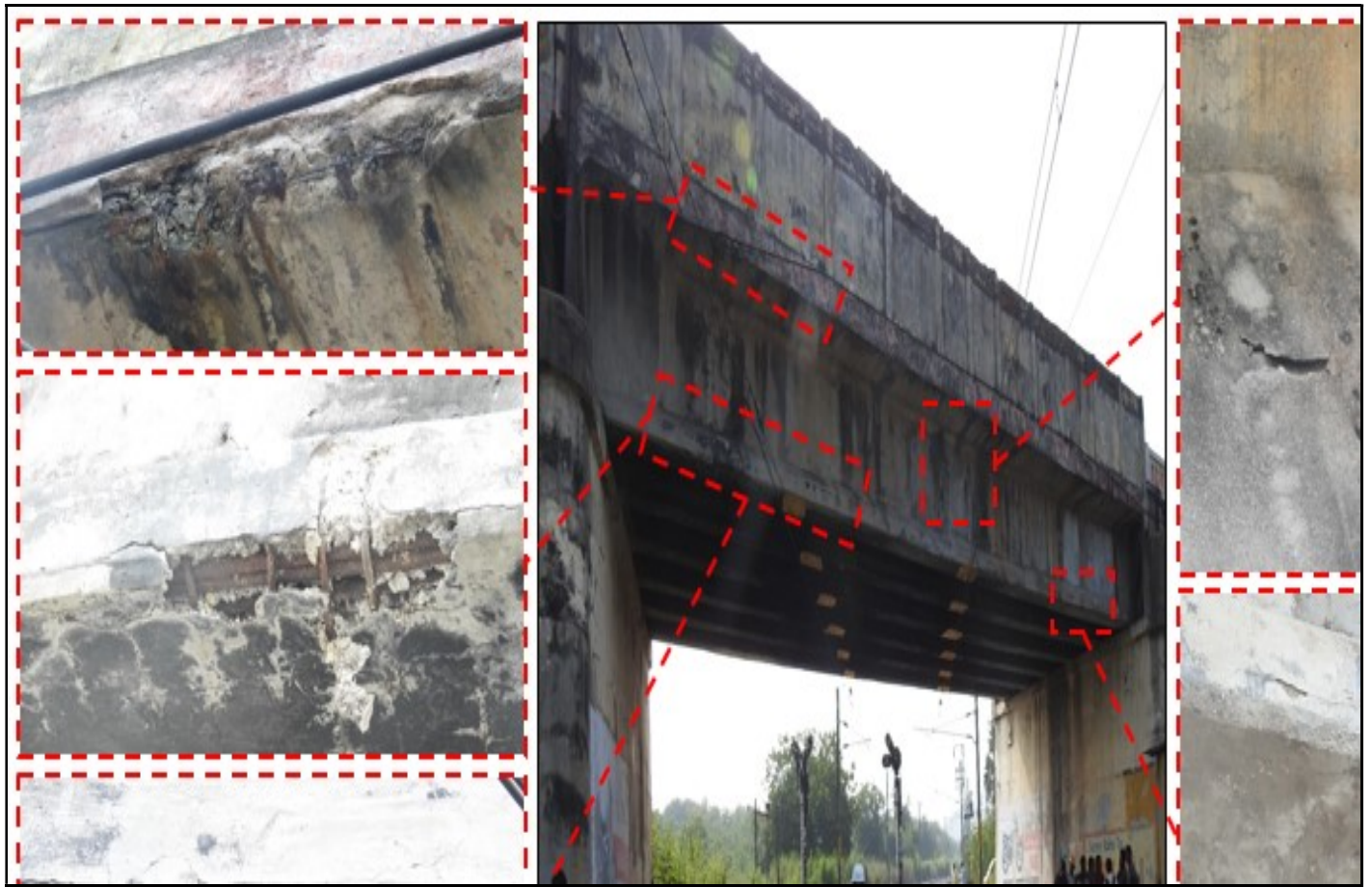
Fig.5 : Patch work, Reinforcement exposed and Structural Cracks at Span-1
