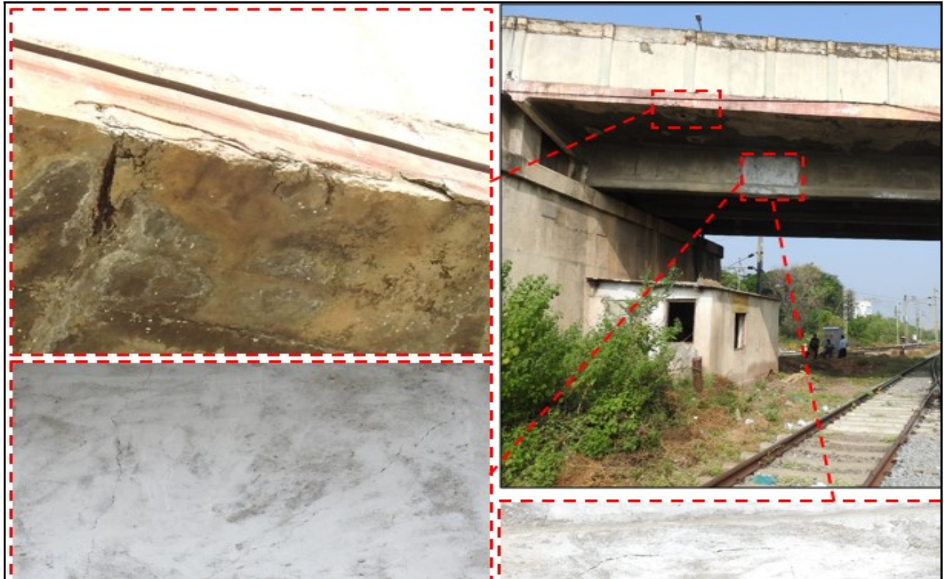
Fig.9 : Cracks, patch work and Spalling is observed at main girder and overhang slab of Span-2.
