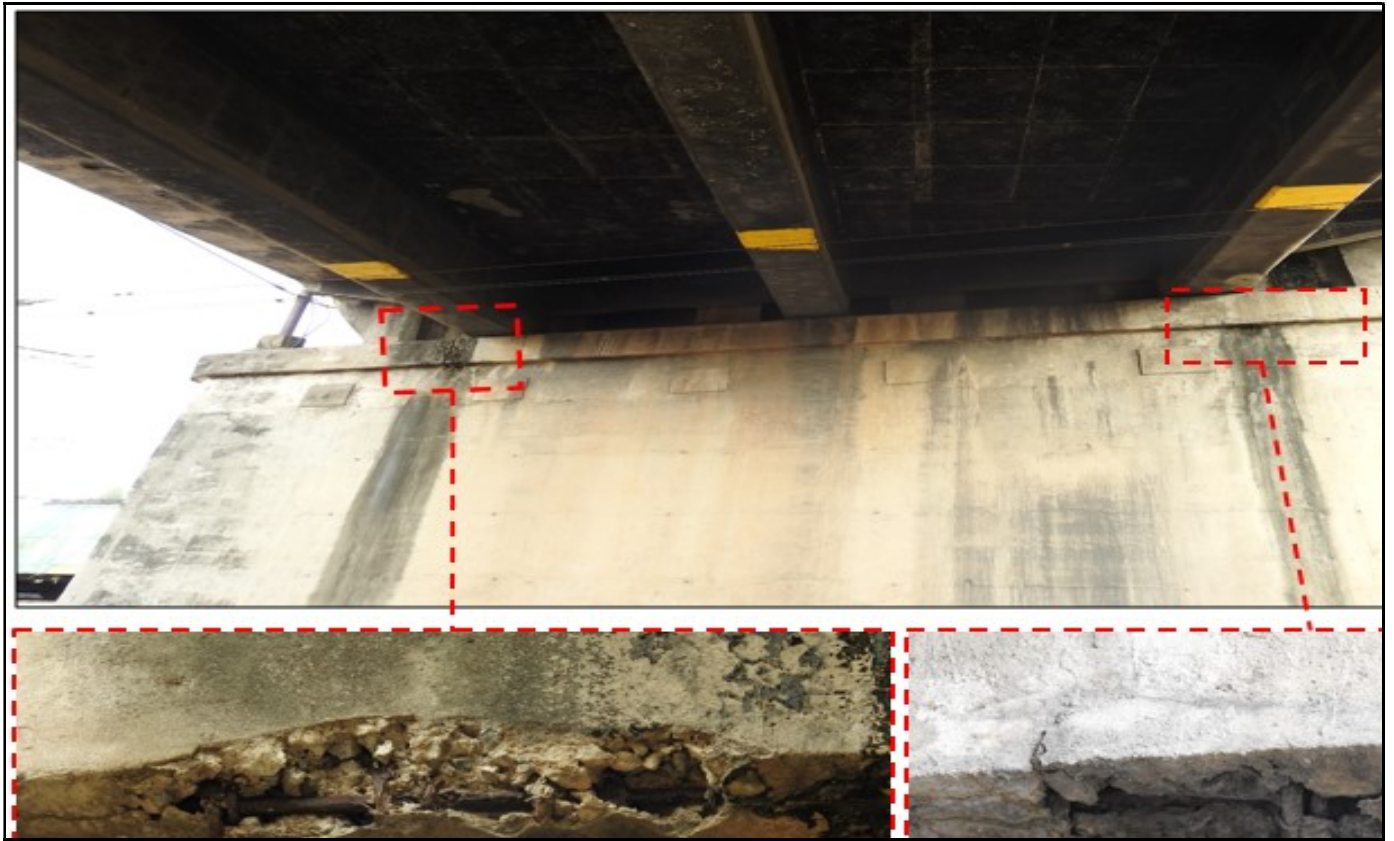
Fig.11 : Reinforcement exposed, spalling and cracks observed at pair-3 .
