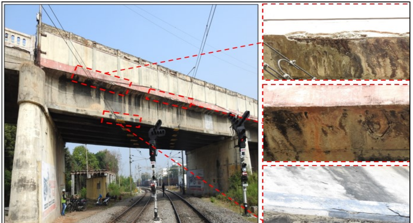
Fig.6 : Spalling, Cracks, leaching and Reinforcement exposed is observed at Main girder of span-1 and overhanging portion of slab.
