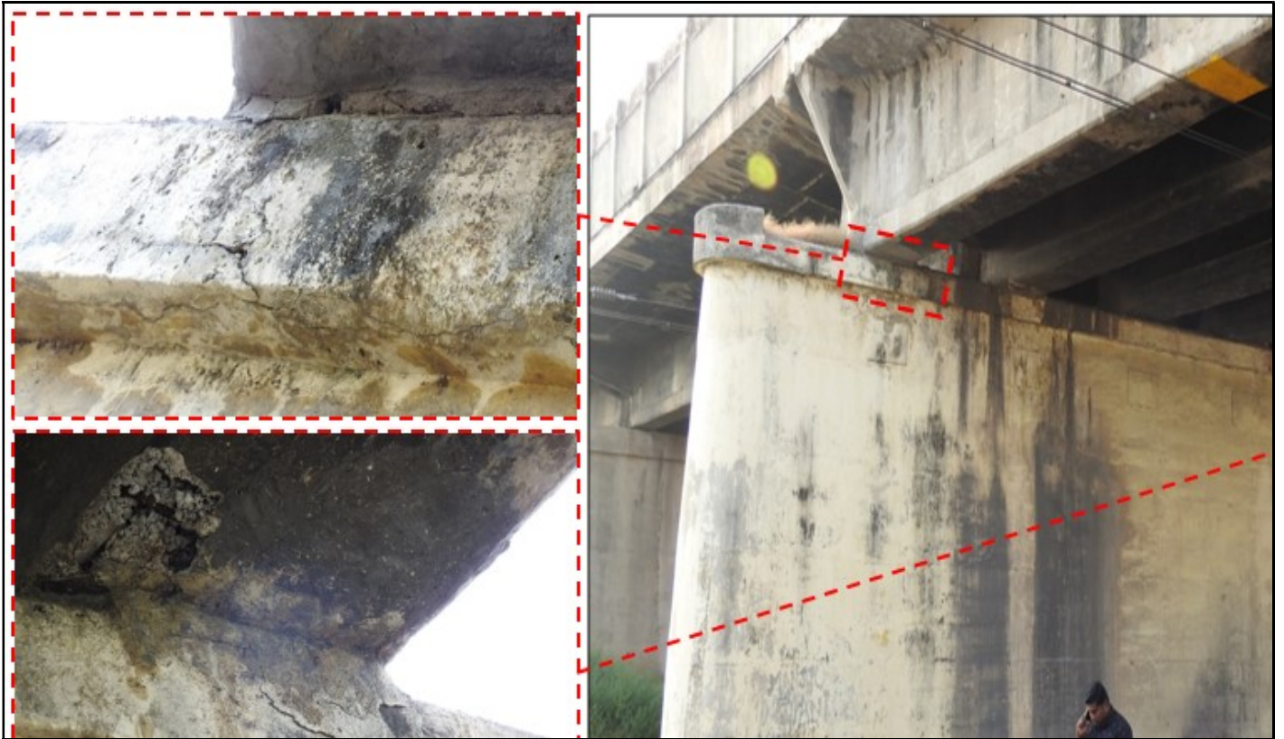
Fig.13 : Spalling , cracks and Reinforcement exposed observed at Pier cap and girder joint of Pier-4 .
