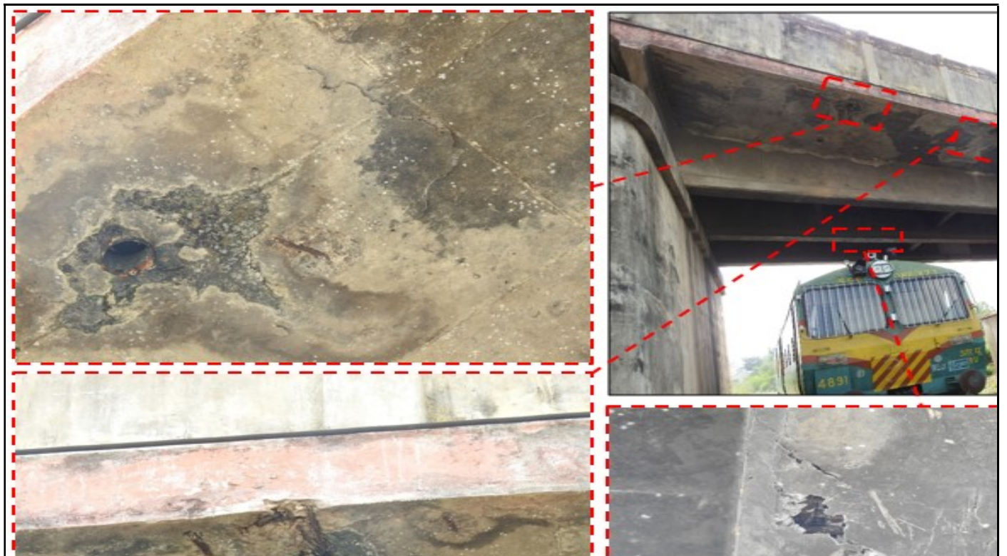
Fig.8 : Reinforcement exposed and Spalling is observed at overhang slab portion and Main girder of Span-2.
