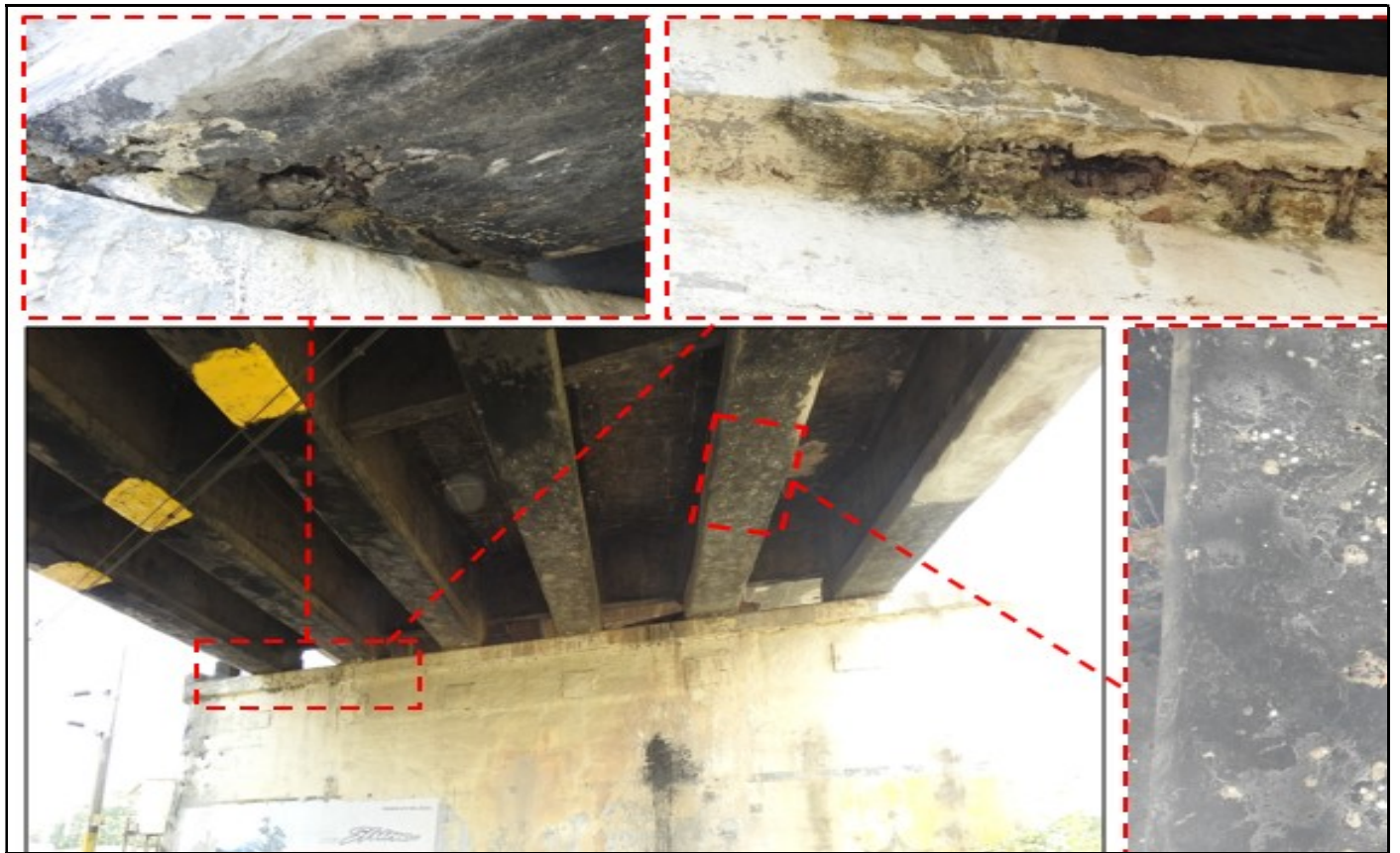
Fig.7 : Reinforcement exposed and Spalling is observed at pier cap and main girder of Span 1.
