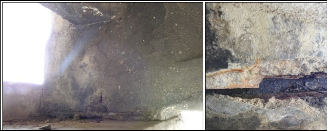
Fig.3 : Metallic plate Bearings corrosion observed at span 1 and 4
