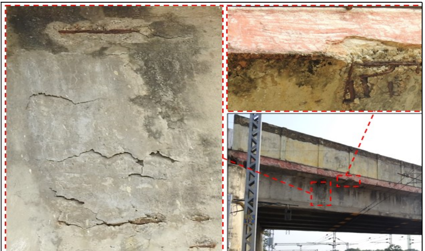
Fig.14 : Spalling and Reinforcement exposed observed at span-4 overhang slab portion .
