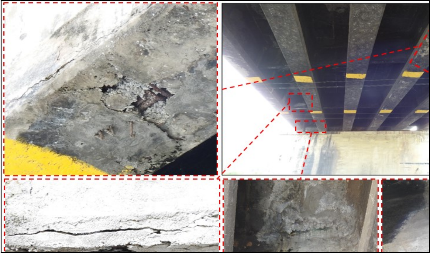
Fig.15 : Reinforcement exposed , Spalling , leaching and patch work observed at main & Secondary girders of span-4 .
