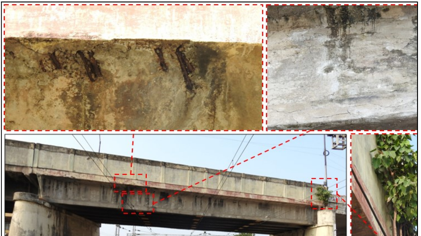
Fig.12 : Reinforced exposed, cracks and vegetation observed at overhang slab portion of span-4 .
