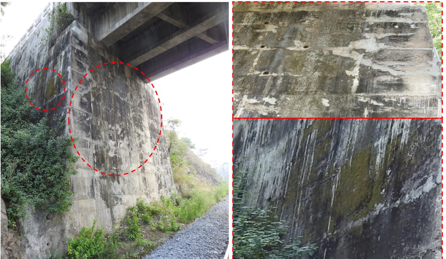
Fig 5: Leaching and algae formation observed at Abutment
