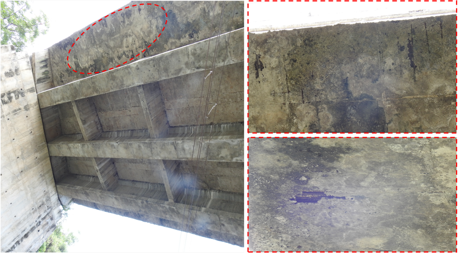
Fig 4: Reinforcement visible at overhang portion of slab
