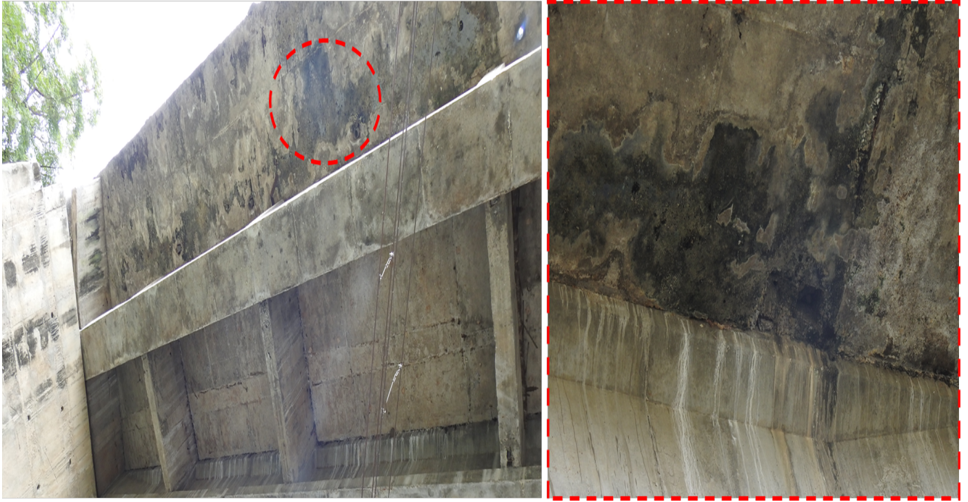
Fig 6: Leaching observed at overhang portion of Slab
