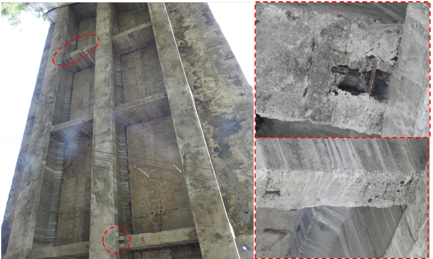
Fig 7: Reinforcement visible at Cross girders
