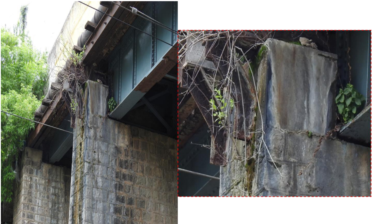
Fig: 3 Vegetation, algae growth, leaching and cracks observed at Piers
