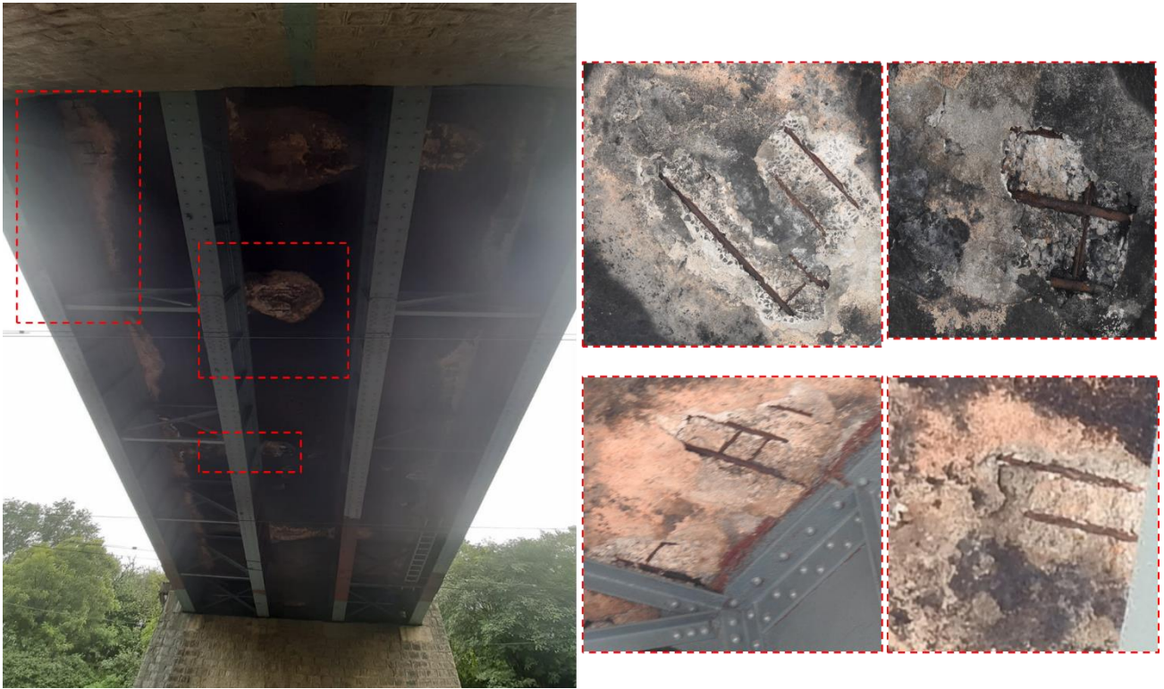
Fig: 4 Exposed reinforcement observed in span 2
