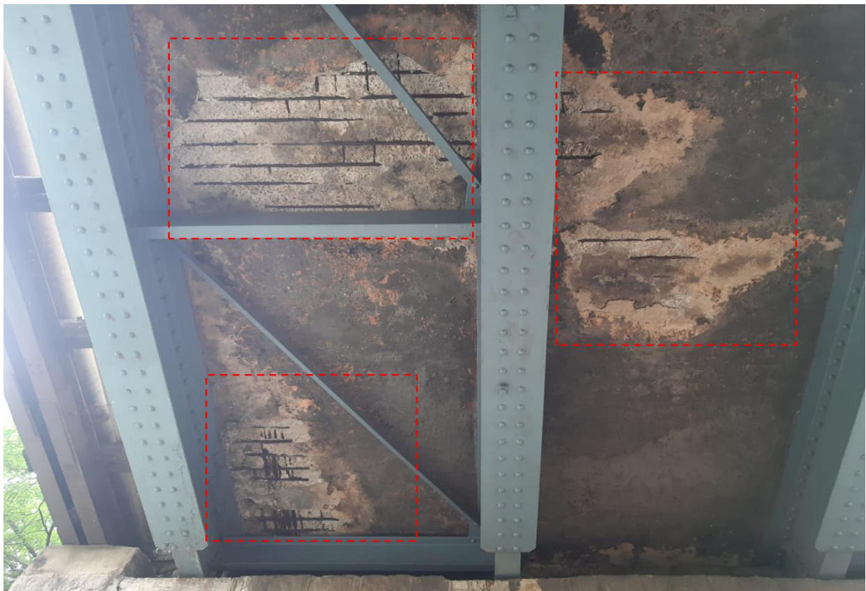
Fig: 5 Exposed reinforcement observed in span 3
