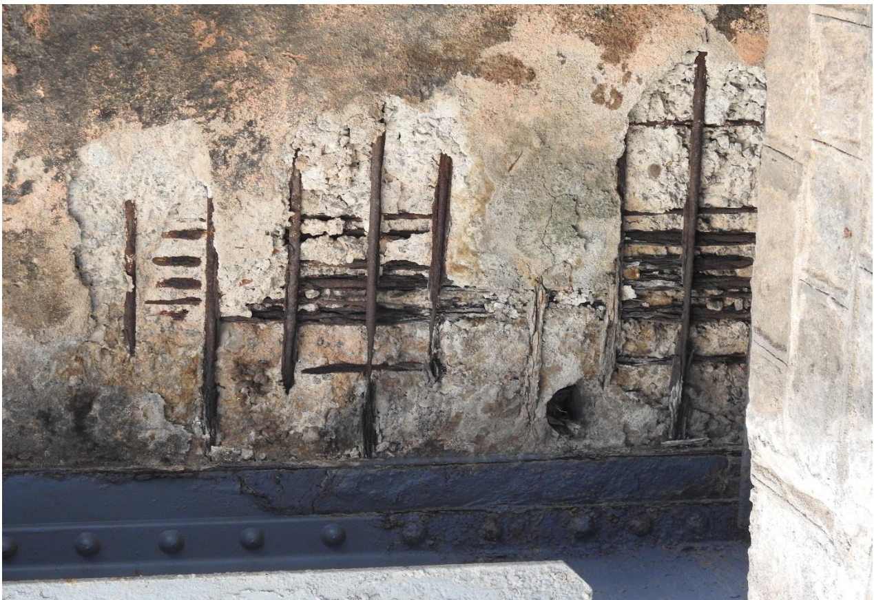
Fig: 11 Reinforcement exposed due to Congested steel, caused no vibrations resulting voids.
