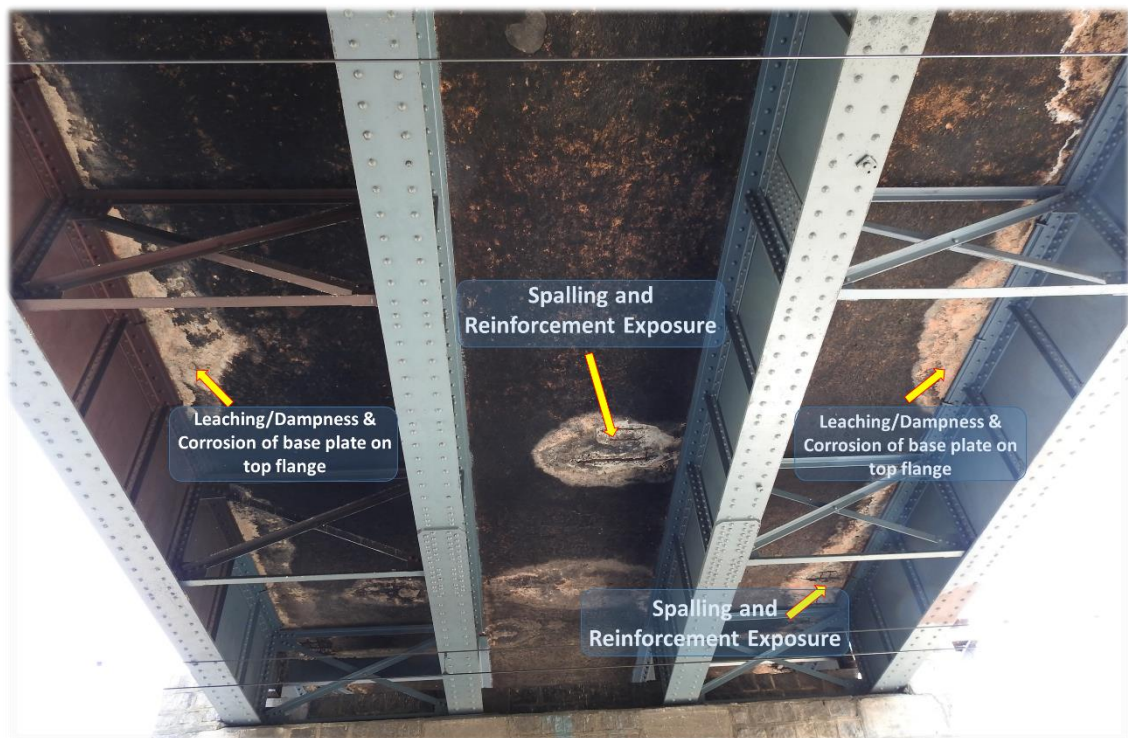
Fig 16: Damage locations identified in span 2 at “e, f & g”
