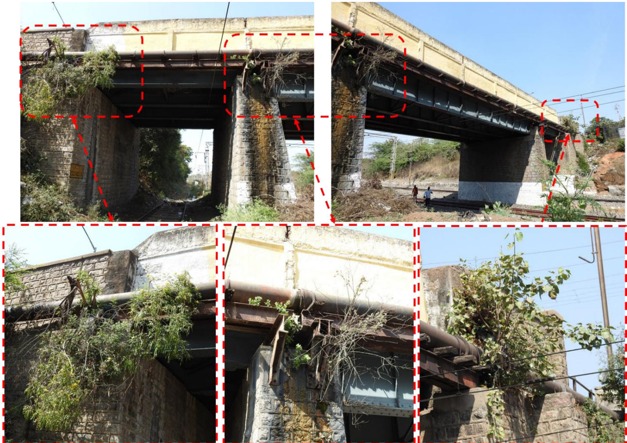
Fig 24: Vegetation observed on the top of the pier (abutment wall)
