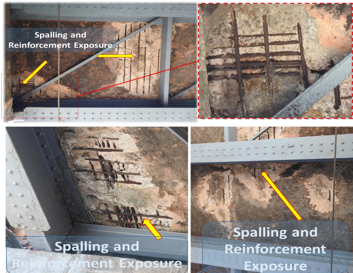
Fig 15: Damage locations identified in span 1 at “a, b, c & d”
