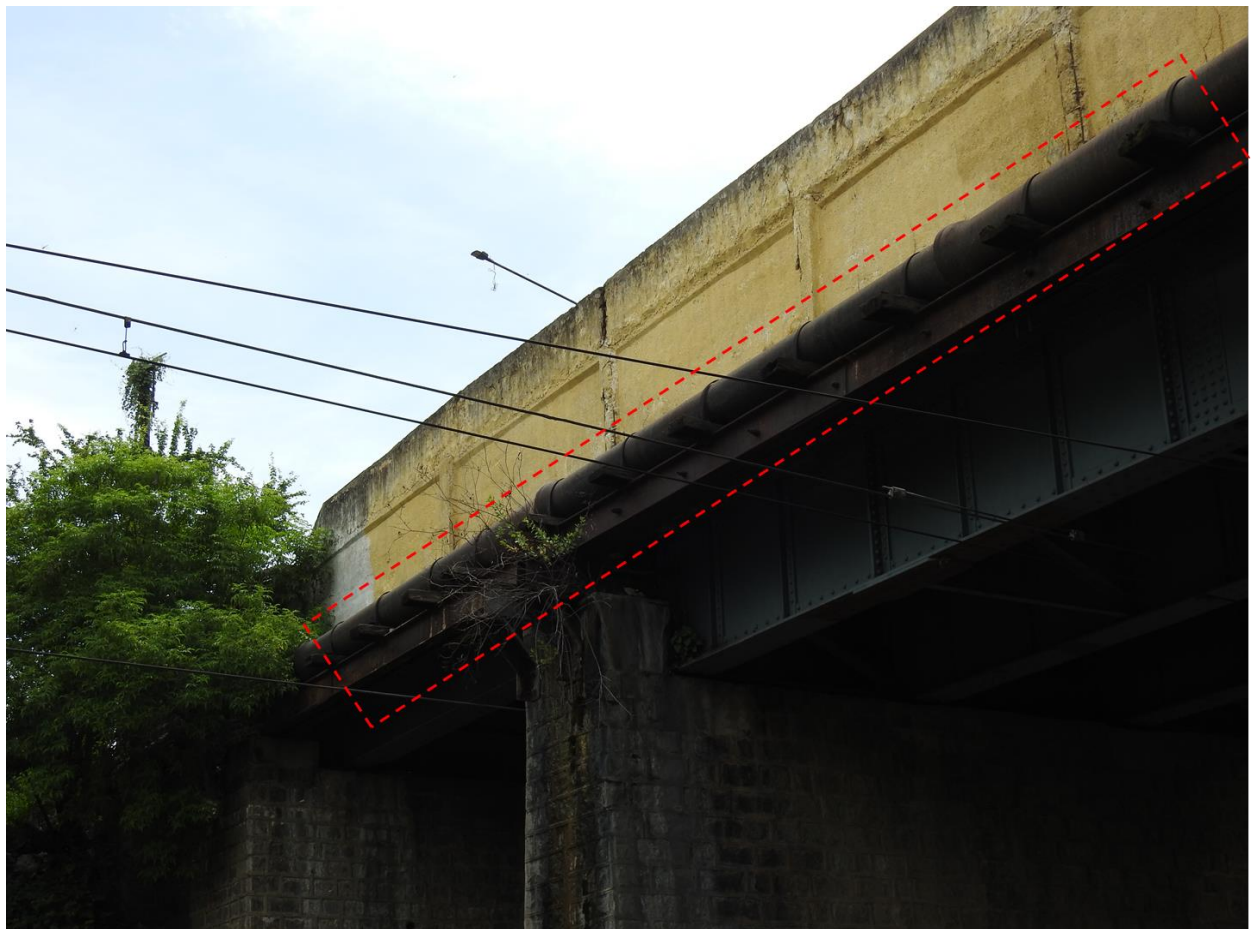
Fig: 9 Additional load of utility is observed
