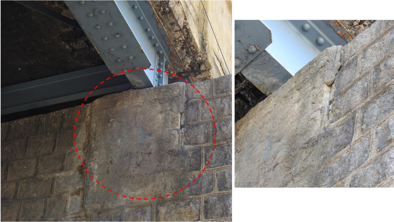
Fig: 12 pointing failure observed at bed block
