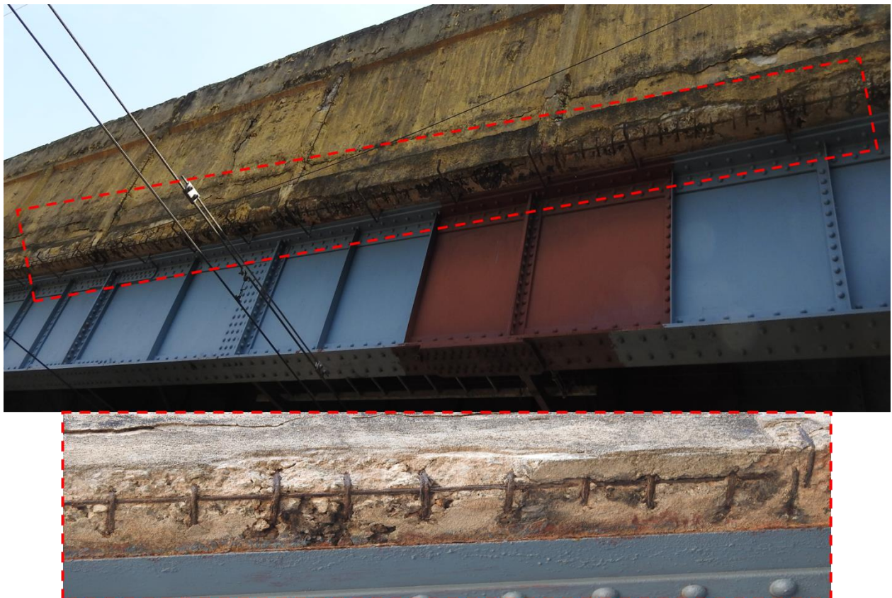
Fig: 7 Spalling and reinforcement exposed at overhang portion of slab due to less cover
