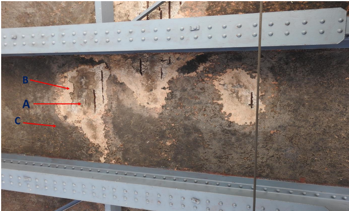
Fig: 10 Patch work observed (A- original concrete, B-old patch work, C-new patch work)
