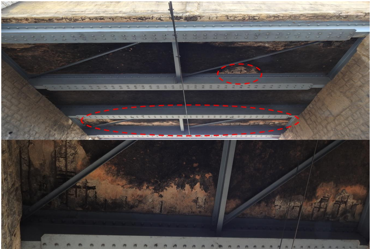
Fig: 8 Spalling and reinforcement exposed at span 1
