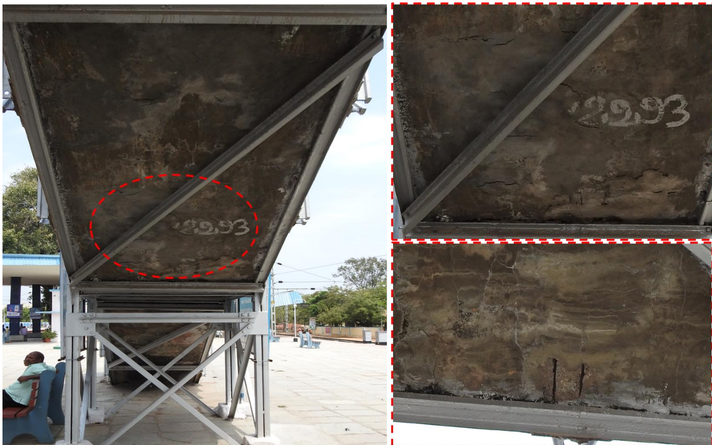
Fig 9: Patch work observed at staircase 2
