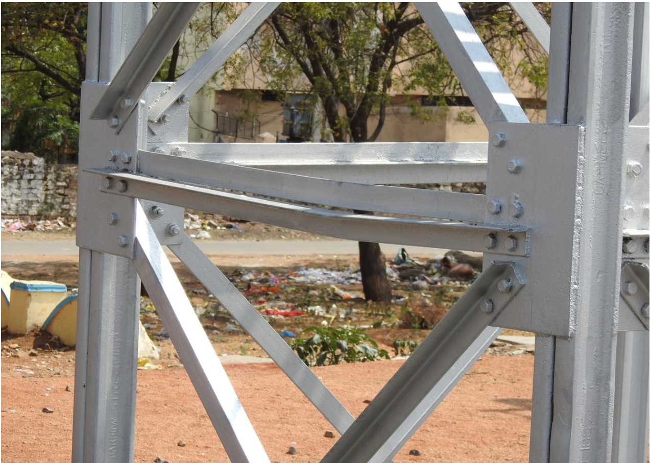
Fig 8: Deformation of bracings at trestle 4
