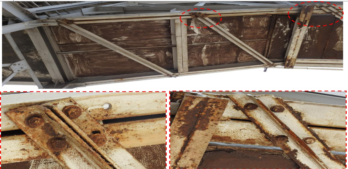
Corrosion observed in Floor beams joints of span 2
