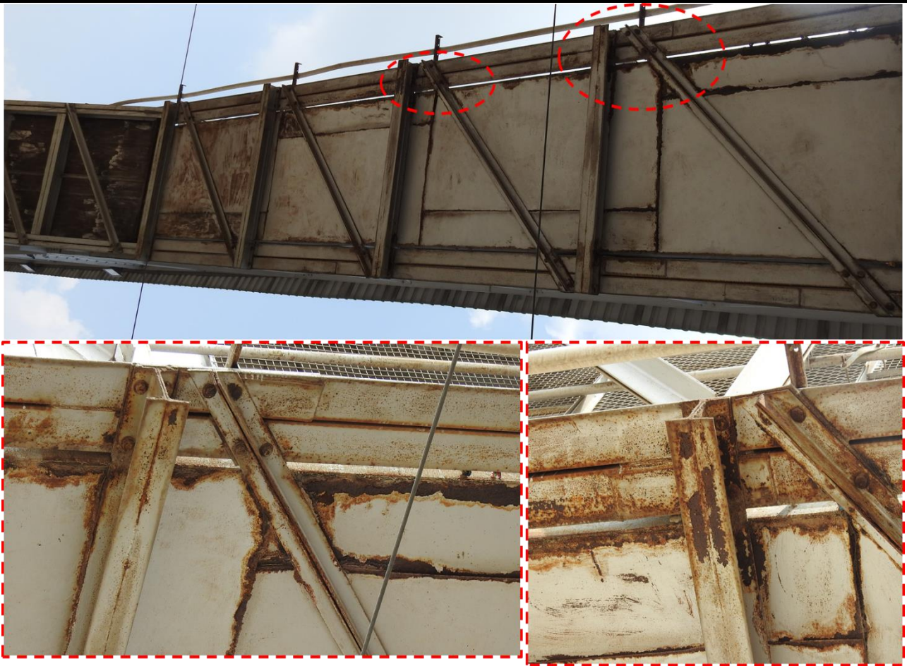
Corrosion of floor beam joints of span 3
