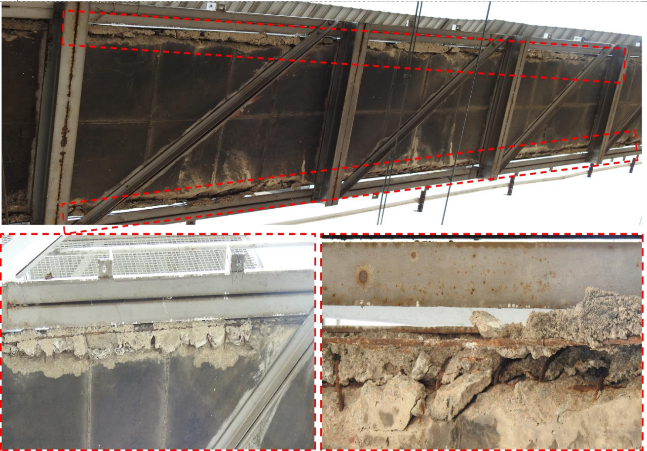
Spalling and reinforcement exposure
