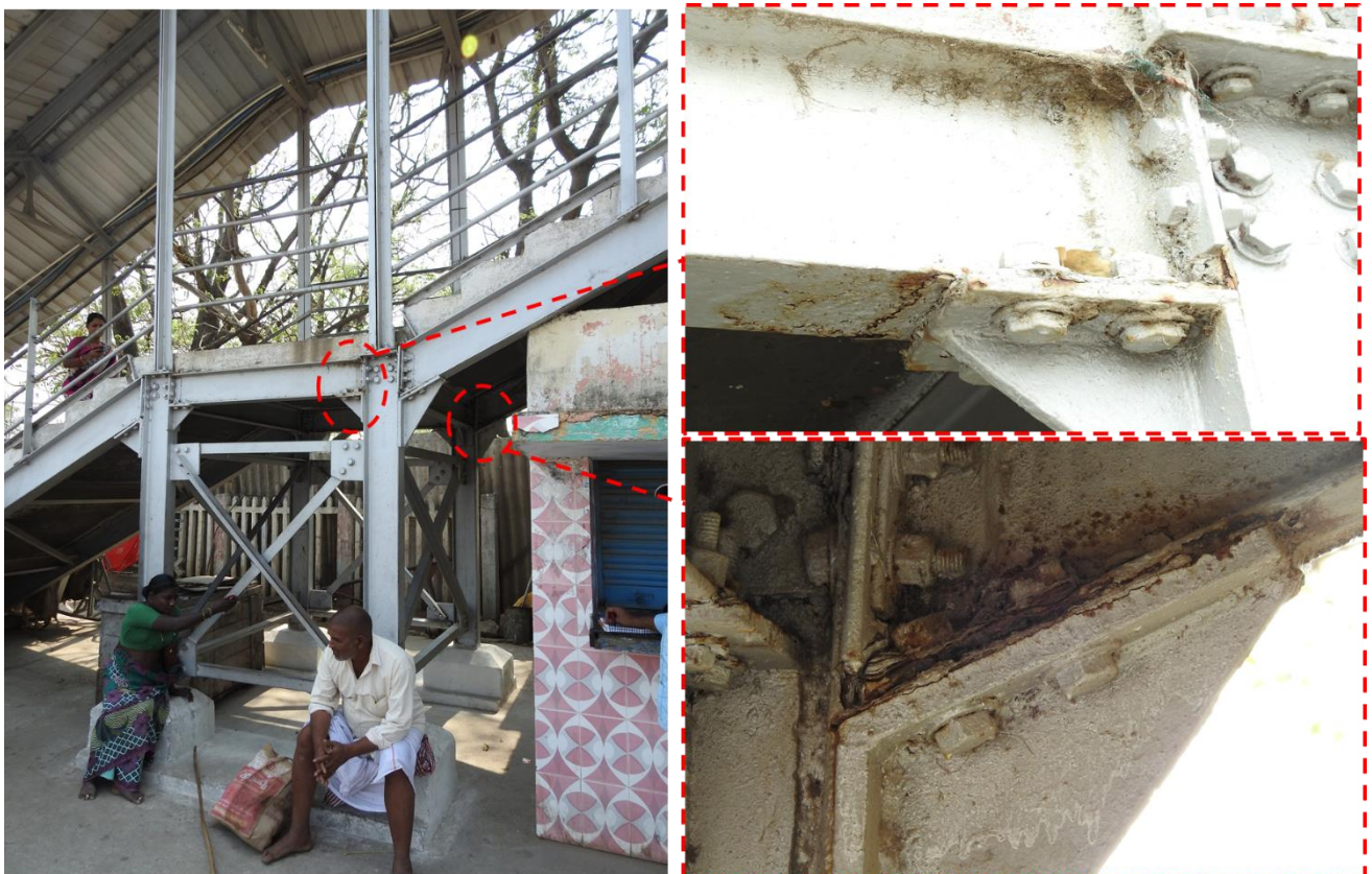
Corrosion at mid landing beam column joint.
