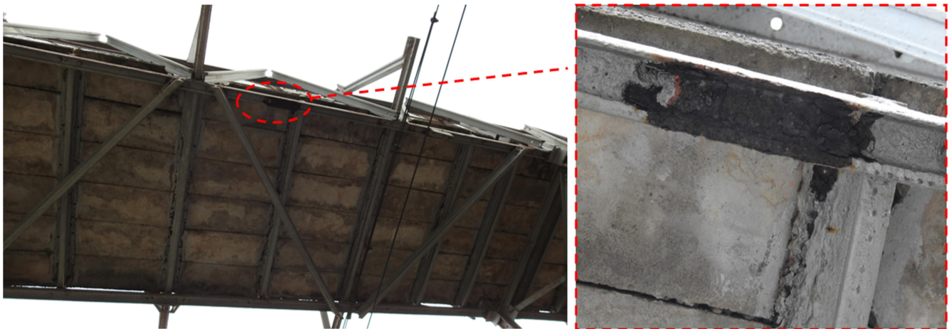
d) Corrosion of Bottom chord in Span 2
