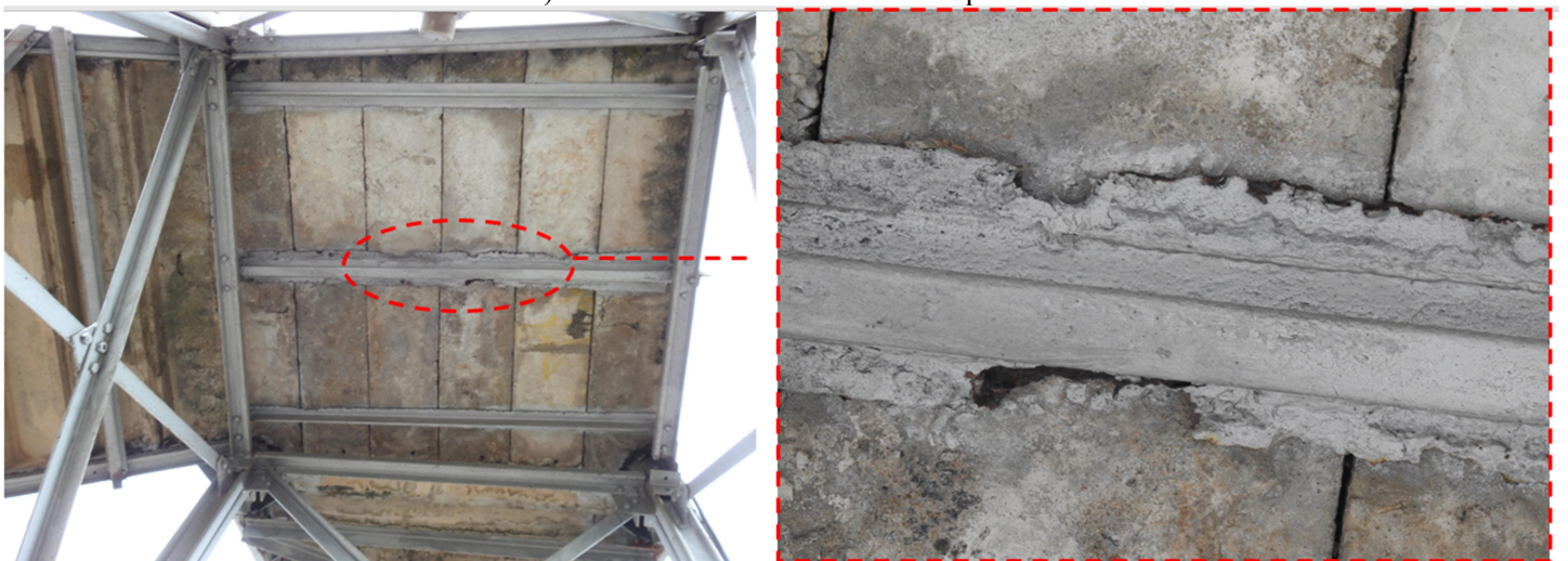
e) Corrosion of Floor beam at landing
