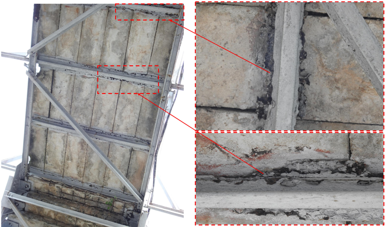
b) Corrosion of Floor Beams at Span-2
