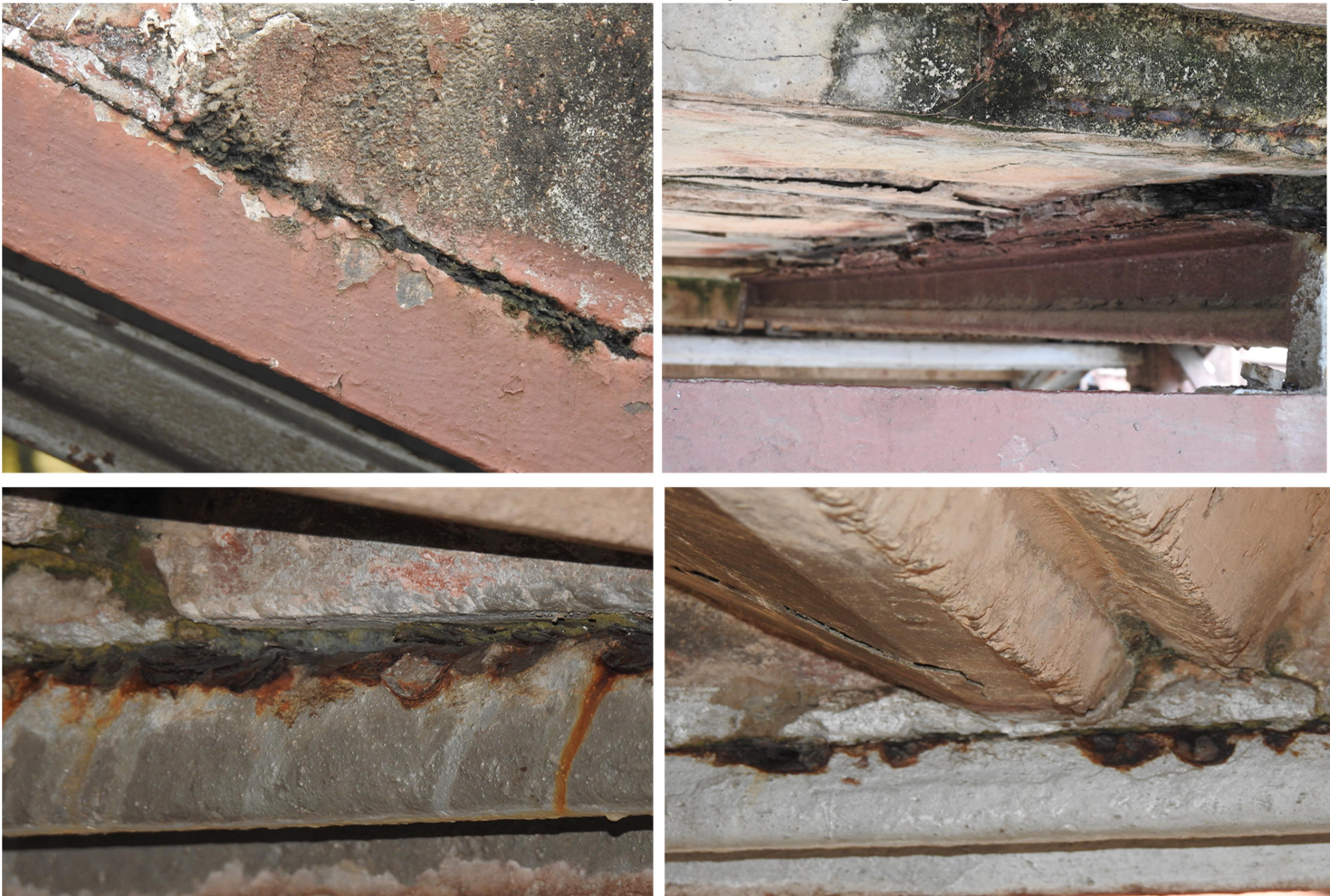
Fig 4: Corrosion is observed at Stringer beam joint
