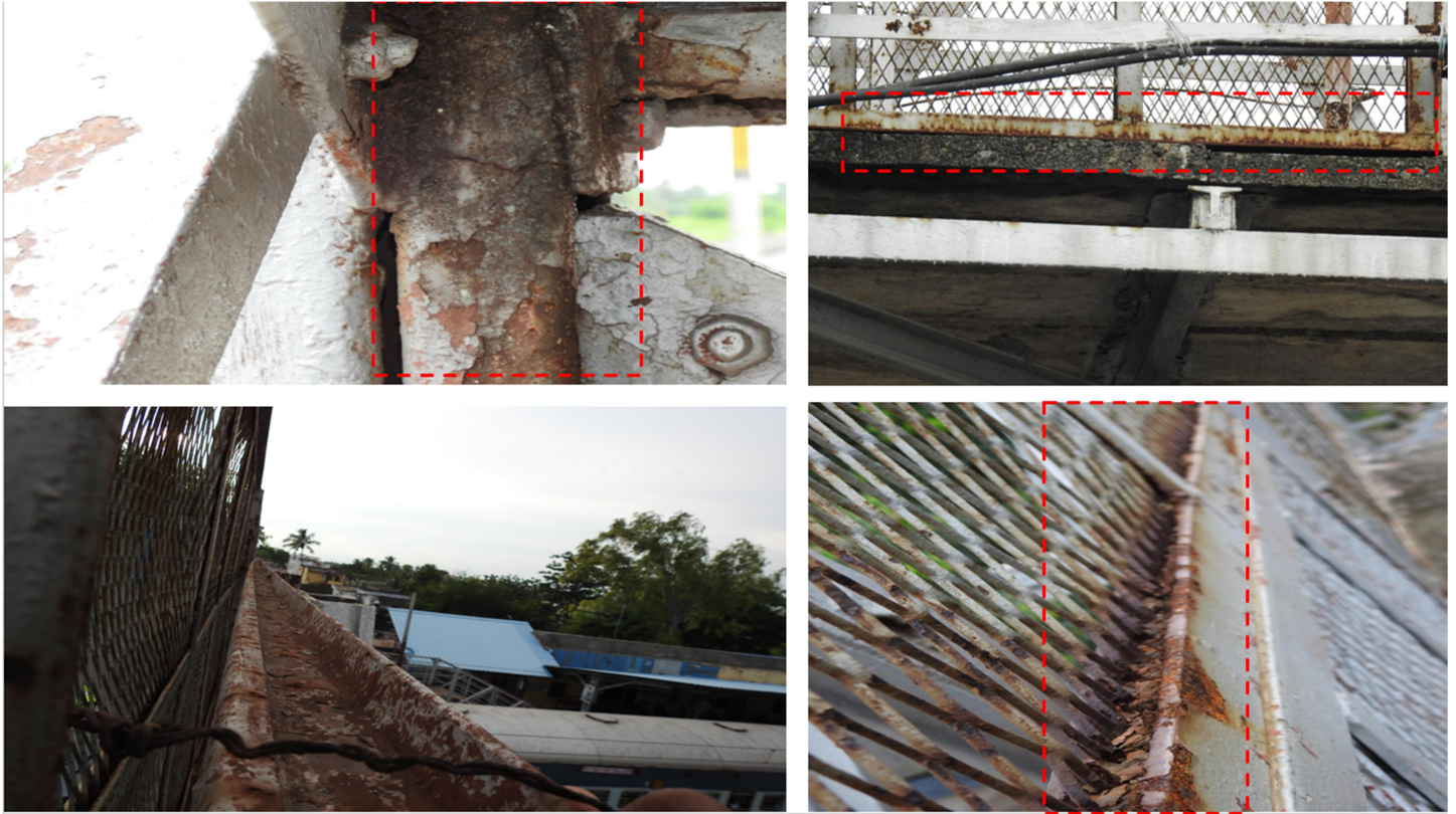
Fig 3: Rusting observed at steel joint & Top chord
