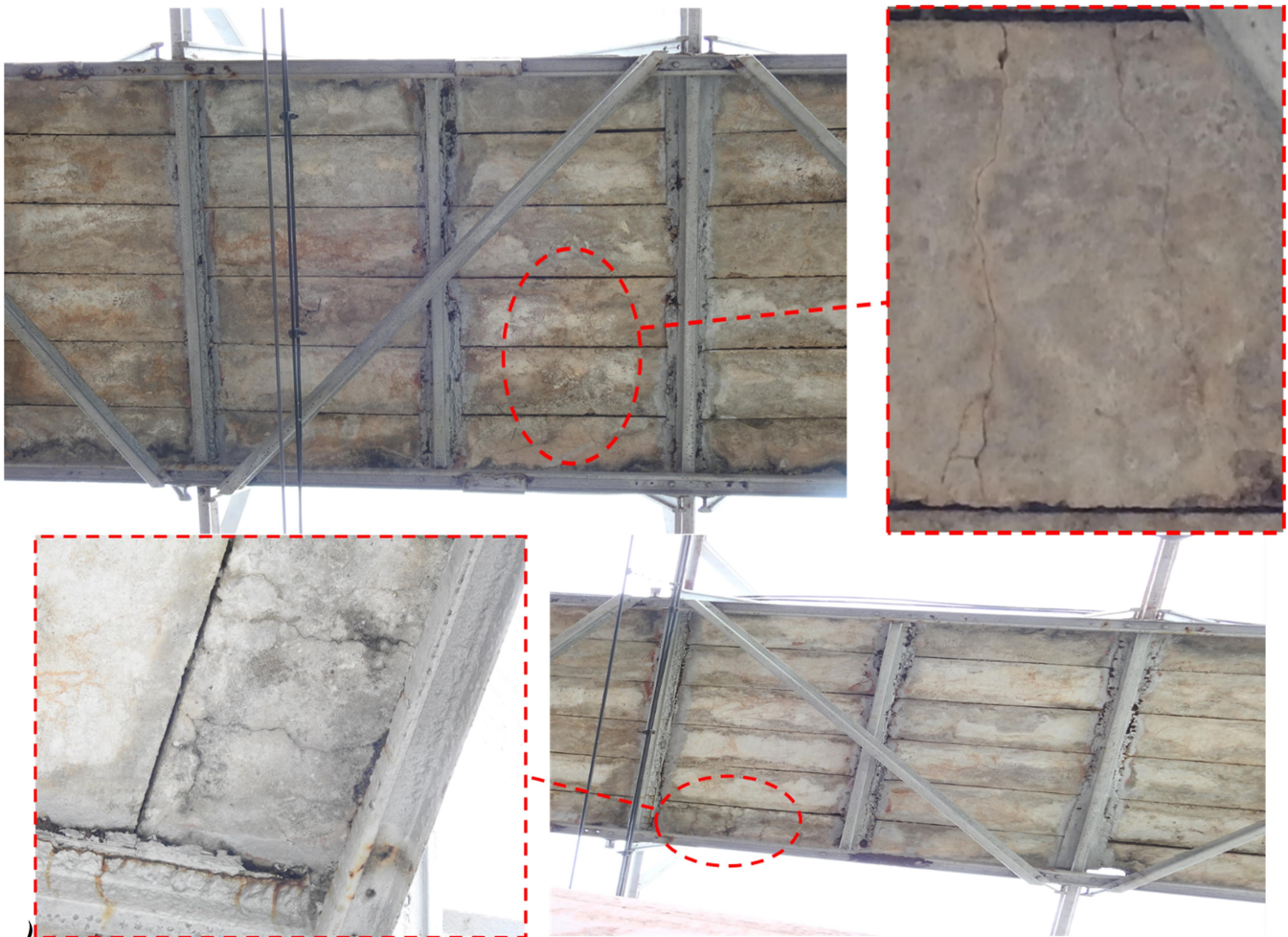
a) Cracks observed at Span-1 & Span 2
