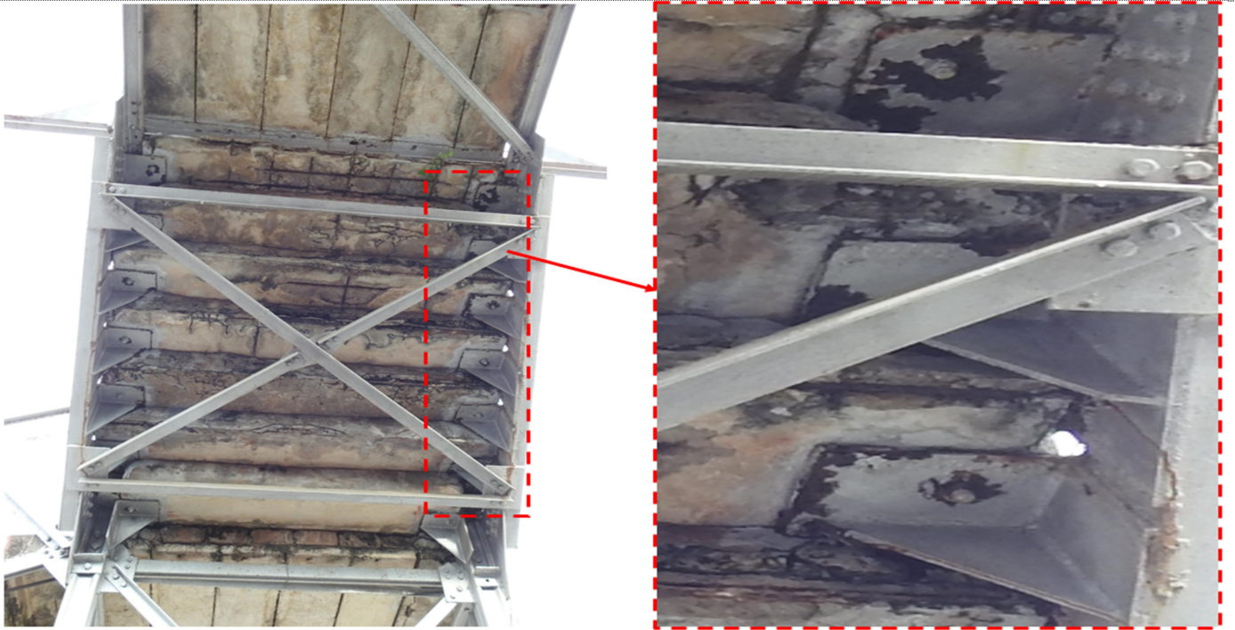
c) Corrosion at Cleat Angles of Stair Case
