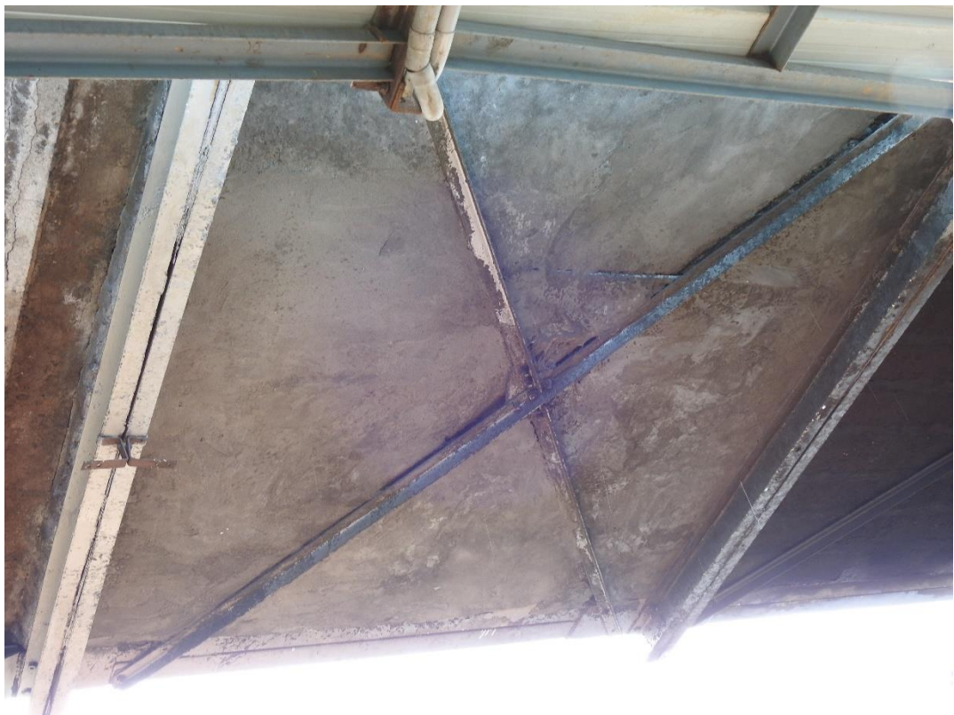
Fig 3.6: pre-cast panels protected with cement mortar from bottom “P9”
