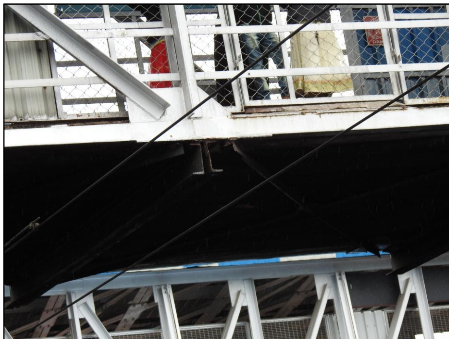
Fig 1.11: Secondary girders joints have severely deteriorated
