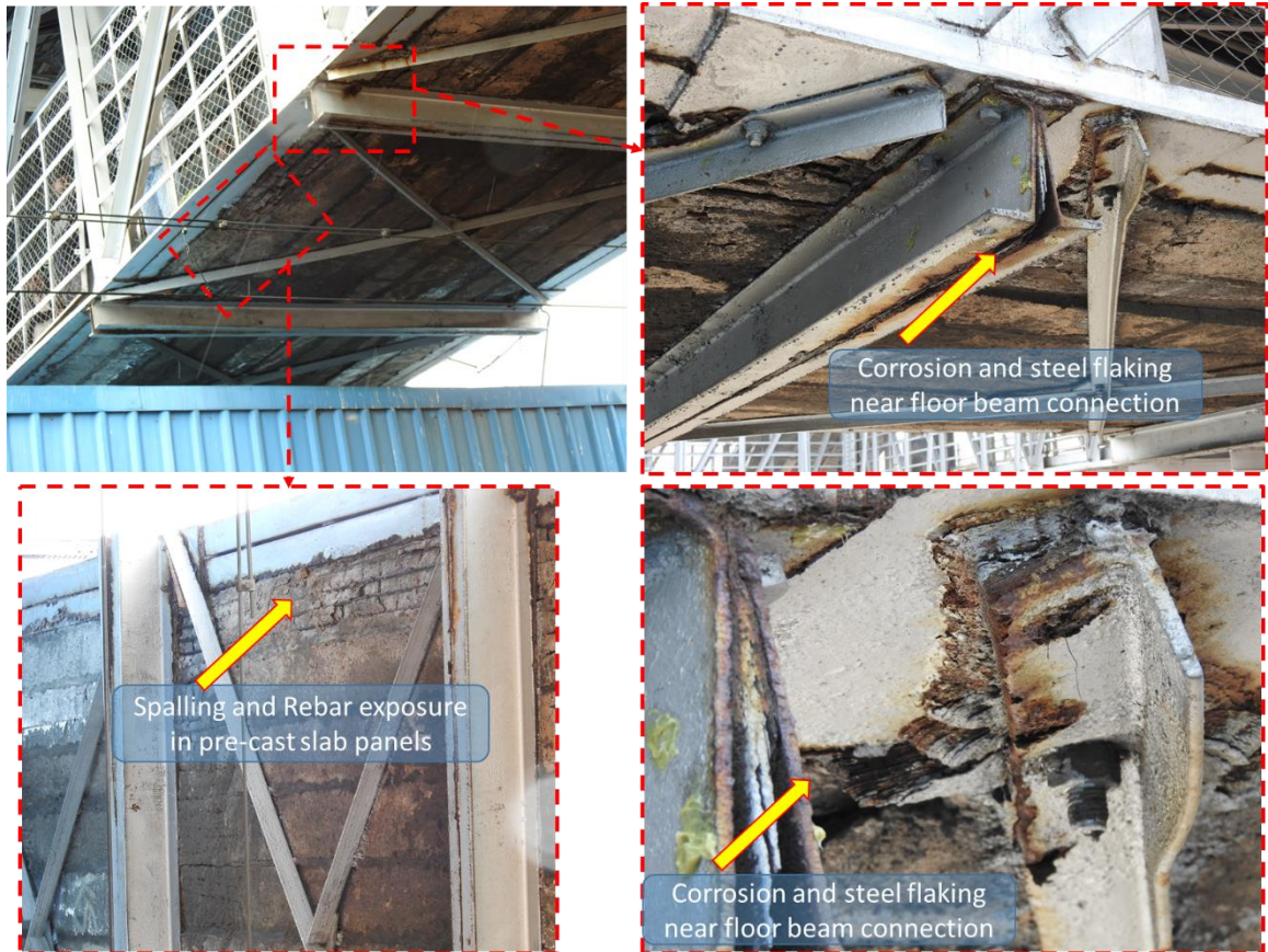
Fig 3.5: Damage locations identified in “P4”
