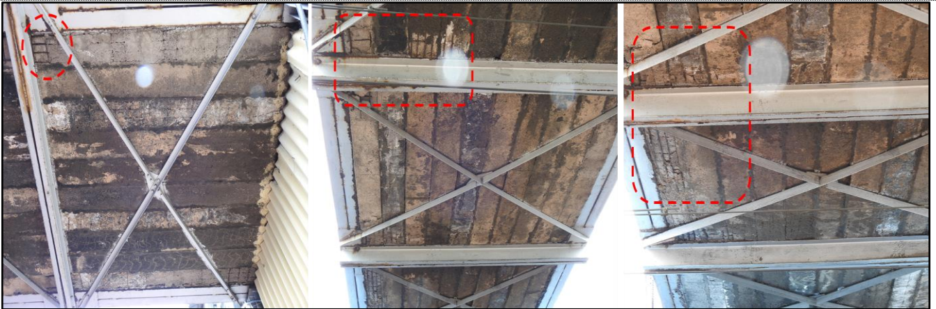
Spalling and leaching effect observed at bottom of slab panels
