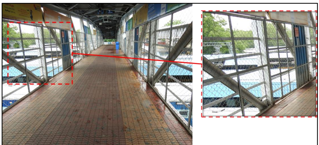
Fig 1.3: Provision of protective screen for passengers over FOB
