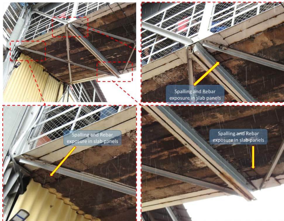
Fig 3.2: Damage locations identified in “P1”
