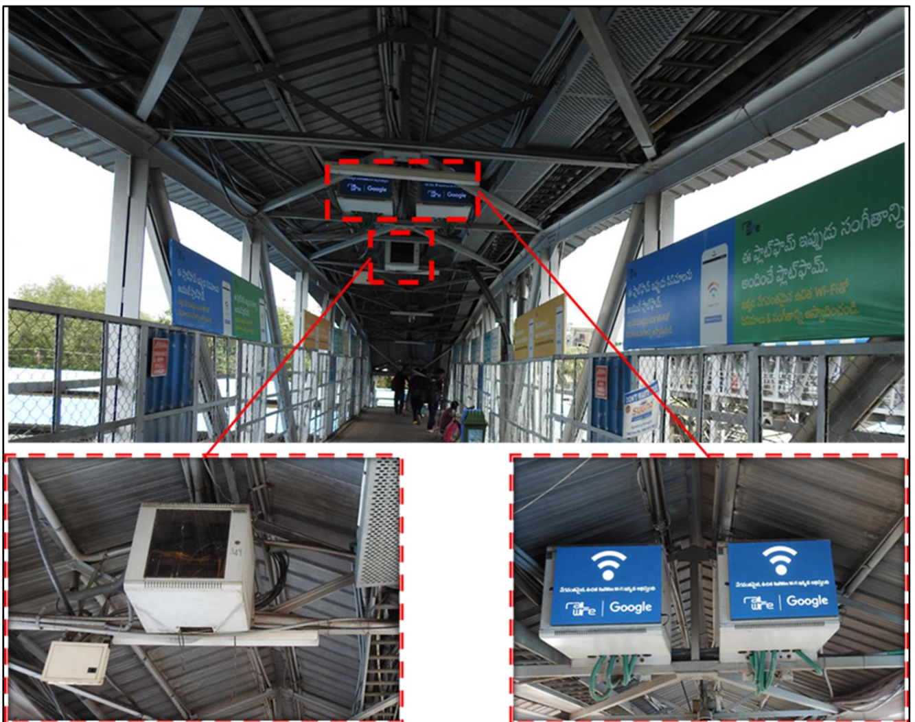
Fig 1.5: Utilities load on roof truss (Ethernet boxes)
