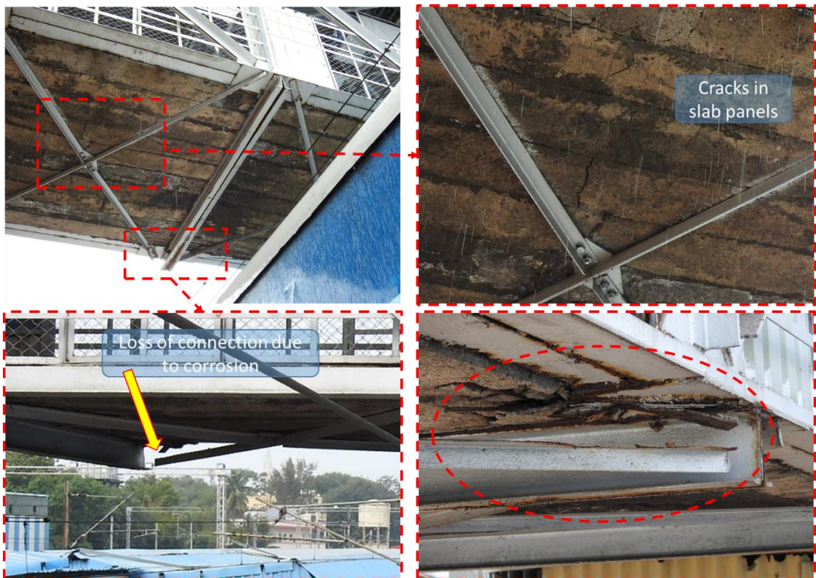
Fig 3.4: Damage locations identified in “P3”
