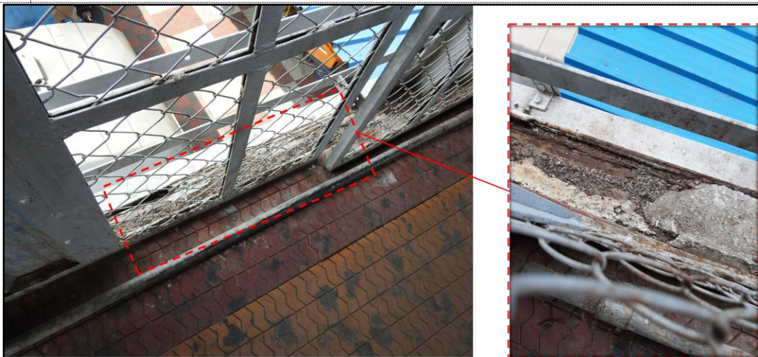
Major Corrosion observed at main girders along the span
