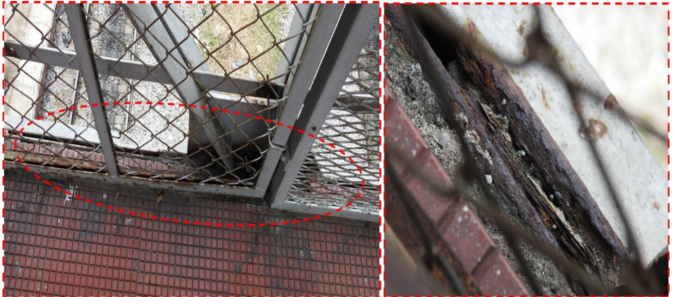
Fig 3.6 corrosion in bottom chord at steel concrete joint
