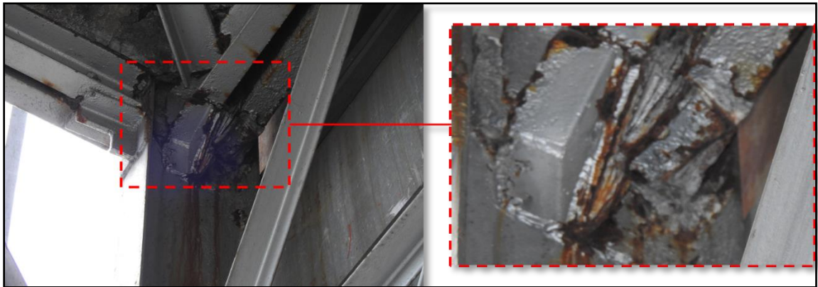
Distressing of Cleat angle is observed at Beam – Column Joint
