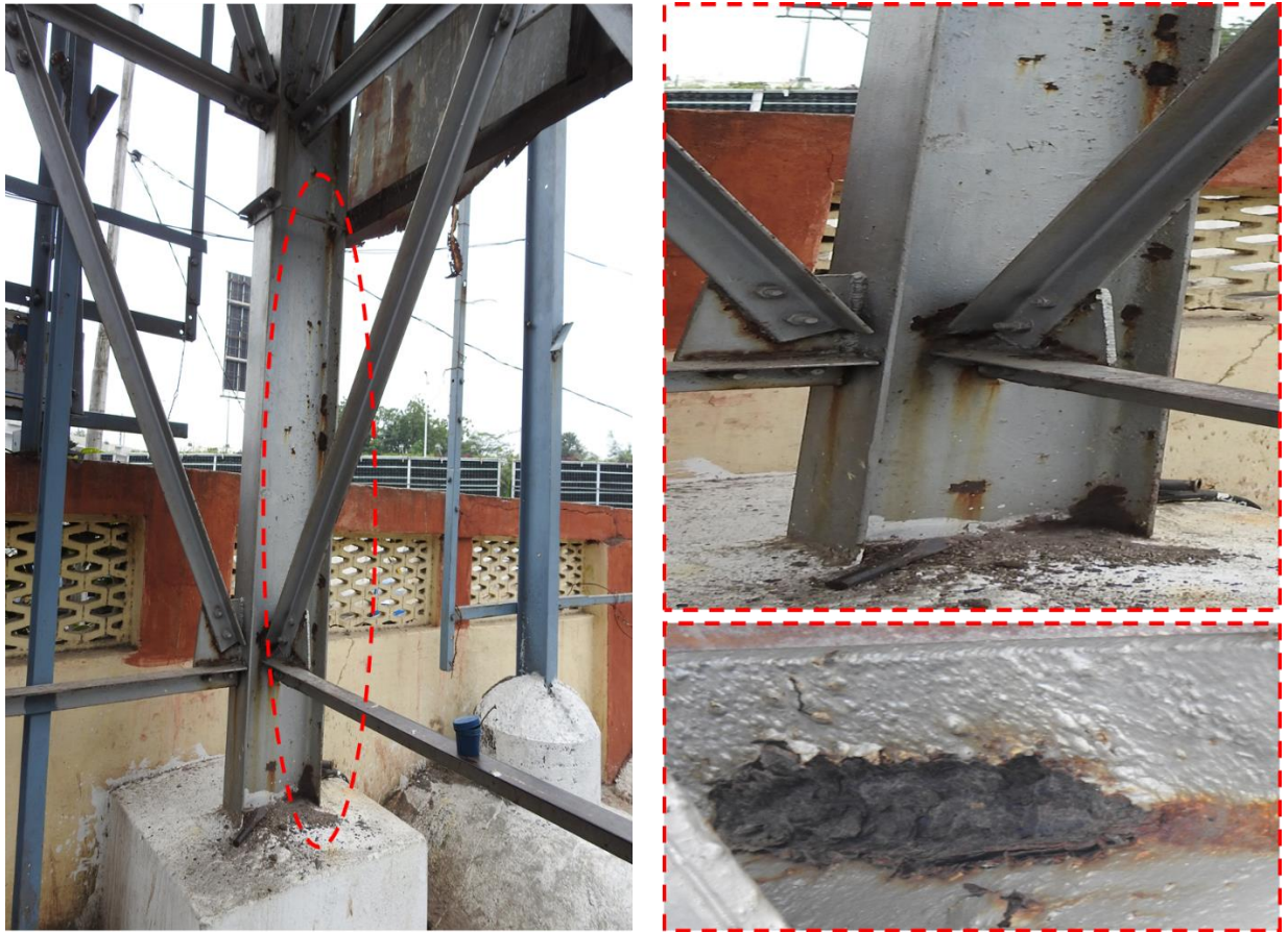
Fig 3.5 Corrosion at column section
