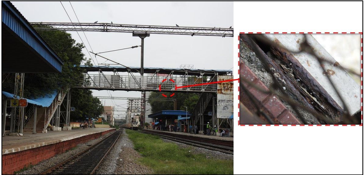
Fig 1.9: Corrosion at concrete-steel joint along the span
