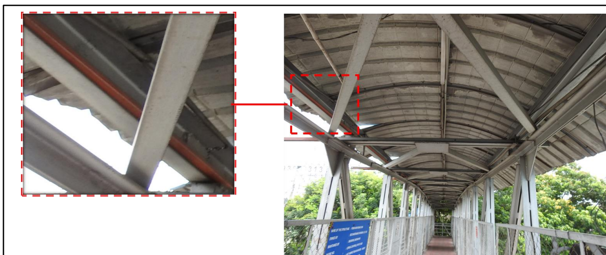
Fig 1.1: Electrical Cables, Roof truss and Roof sheet
