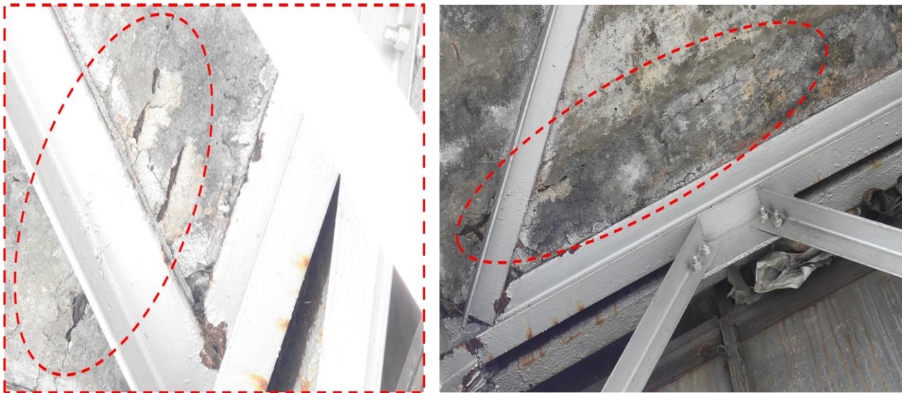
Fig 3.2: Spalling and cracks observed at precast panels
